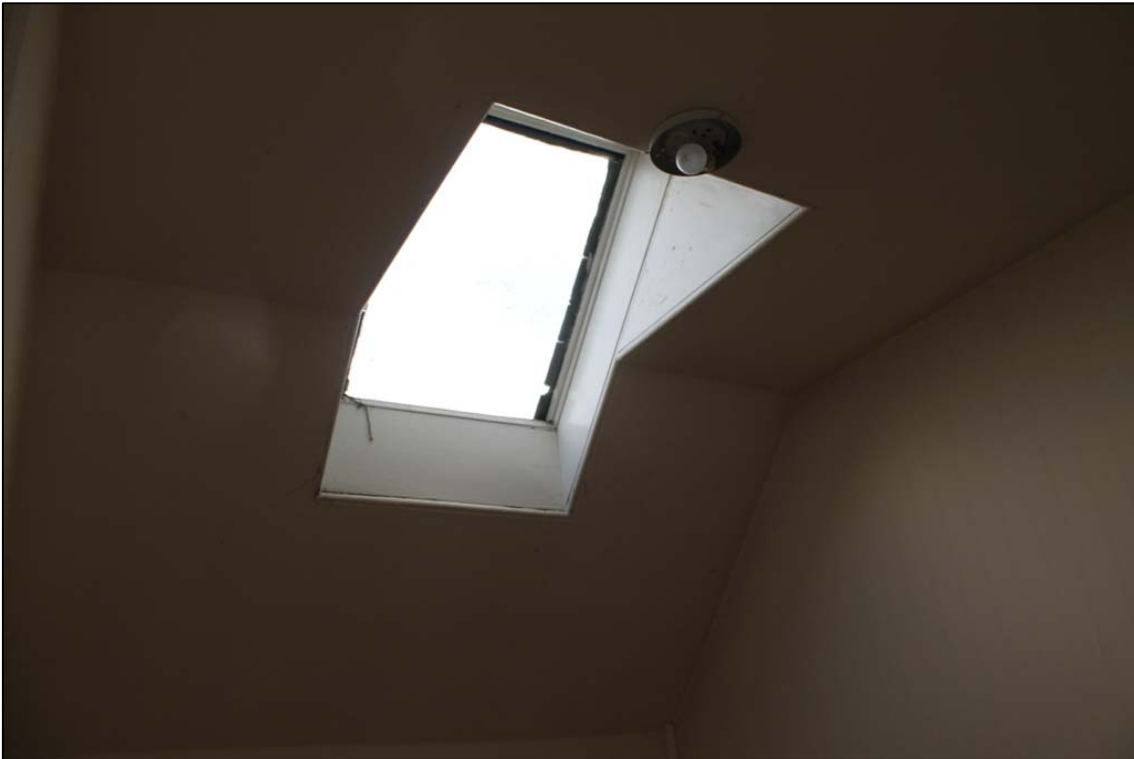
Figure 40b: 1 st floor landing, N wall and modern skylight taken from S
