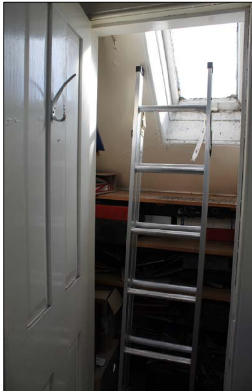
Figure 39b: 1 st floor landing, S wall and Window C taken from N.
