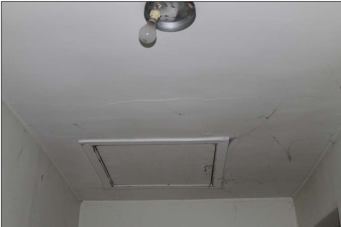
Figure 25b: Hallway of Building B, blocked access to attic taken from the S.
