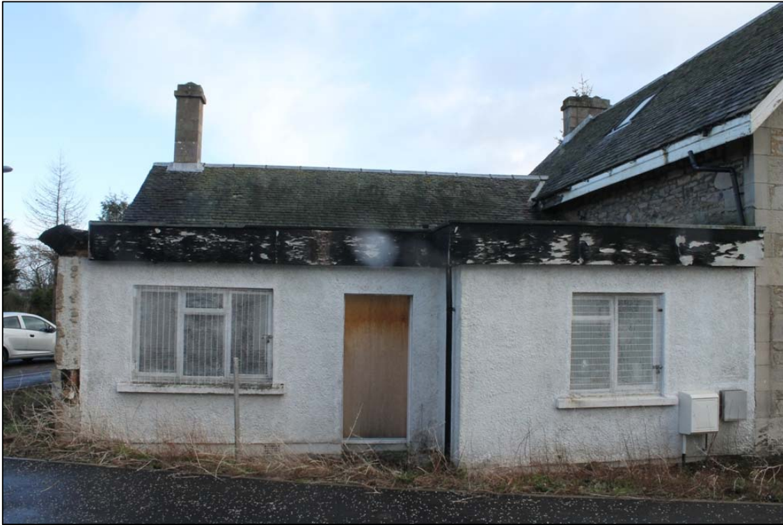
Figure 13a: Doorway and Windows A and B on E elevation of modern extension taken from W.
