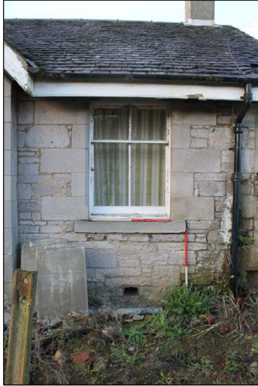
Figure 10a: Detail of Window B on W elevation taken from the E.
