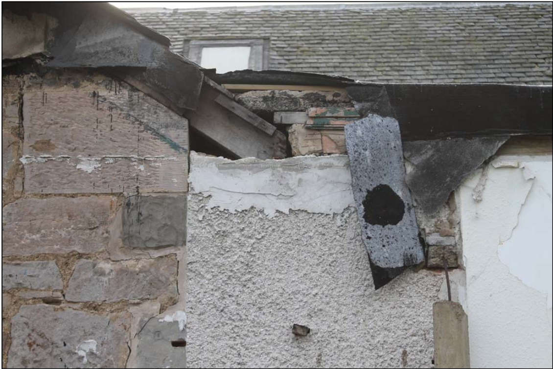
Figure 12a: Detail of damage on the S elevation taken from the north.
