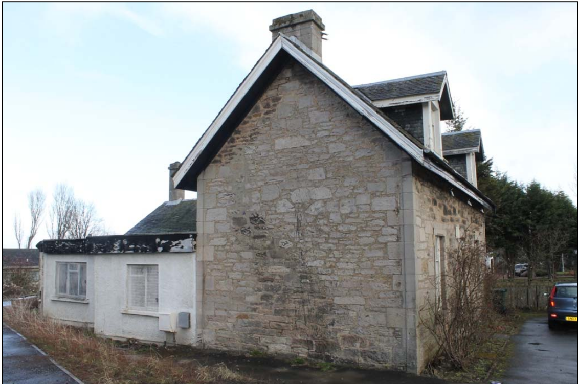
Figure 12b: E elevation of Building A and modern extension taken from the SW
