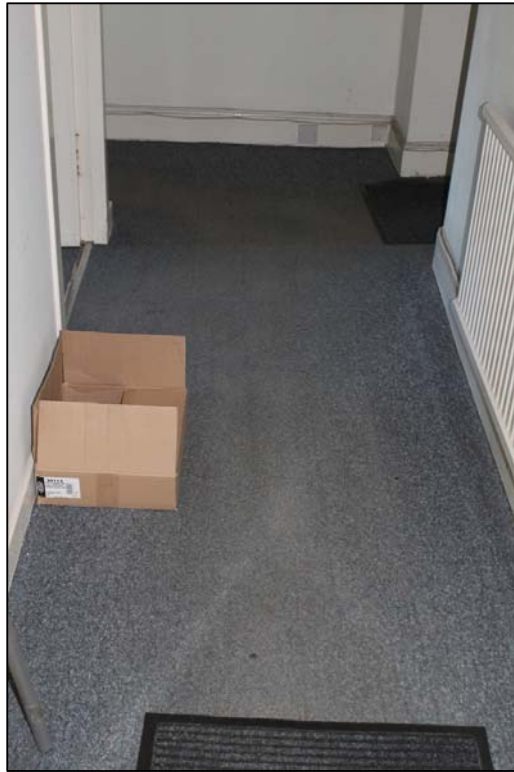
Figure 15a: Detail of carpet present throughout all rooms. Taken in the hallway of Building B from the N.
