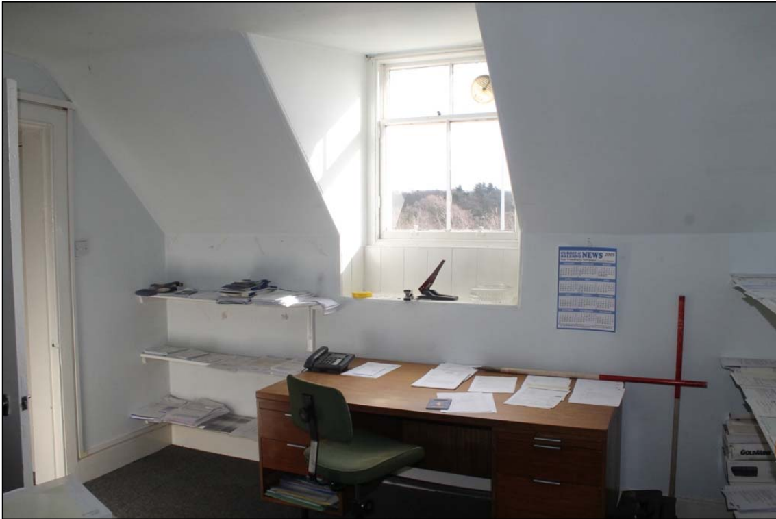
Figure 35a: 1 st floor Room A, S wall and Window A taken from N
