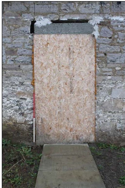
Figure 11b: Detail of boarded up doorway on S elevation taken from the N.
