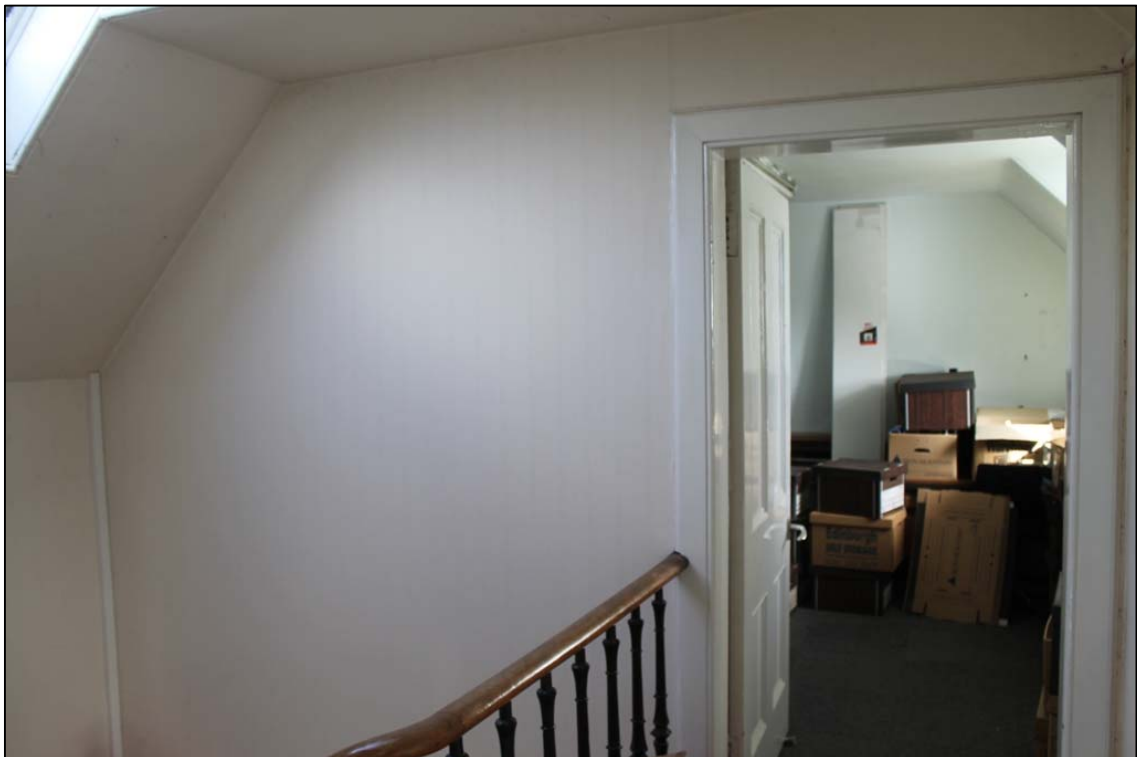
Figure 38b: 1 st floor landing E wall and doorway to Room B taken from W.
