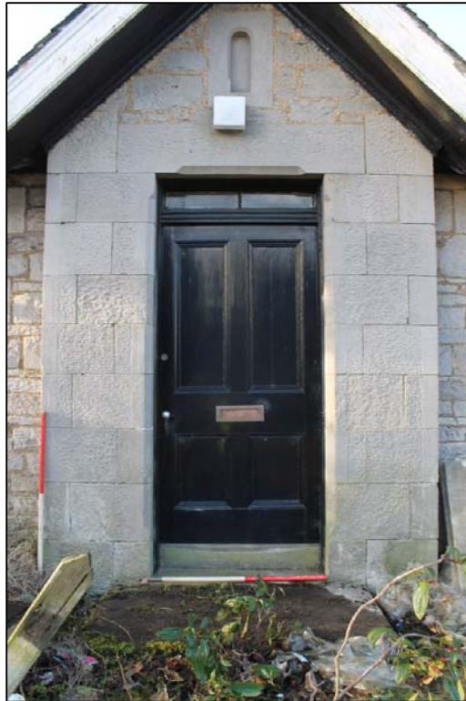
Figure 9b: Detail of alternate access and bell recess on W elevation taken from the E.
