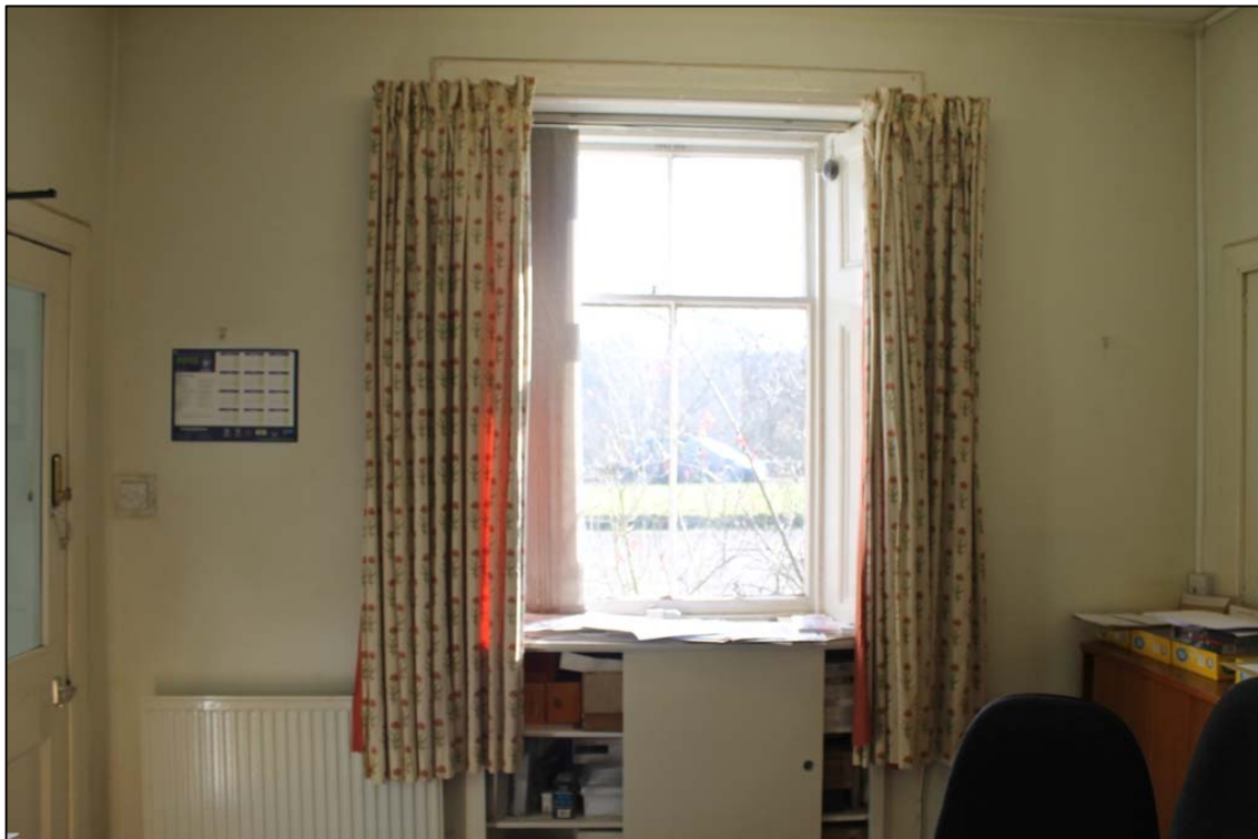
Figure 18b: Room A (ground floor), Window A on S wall taken from the N.
