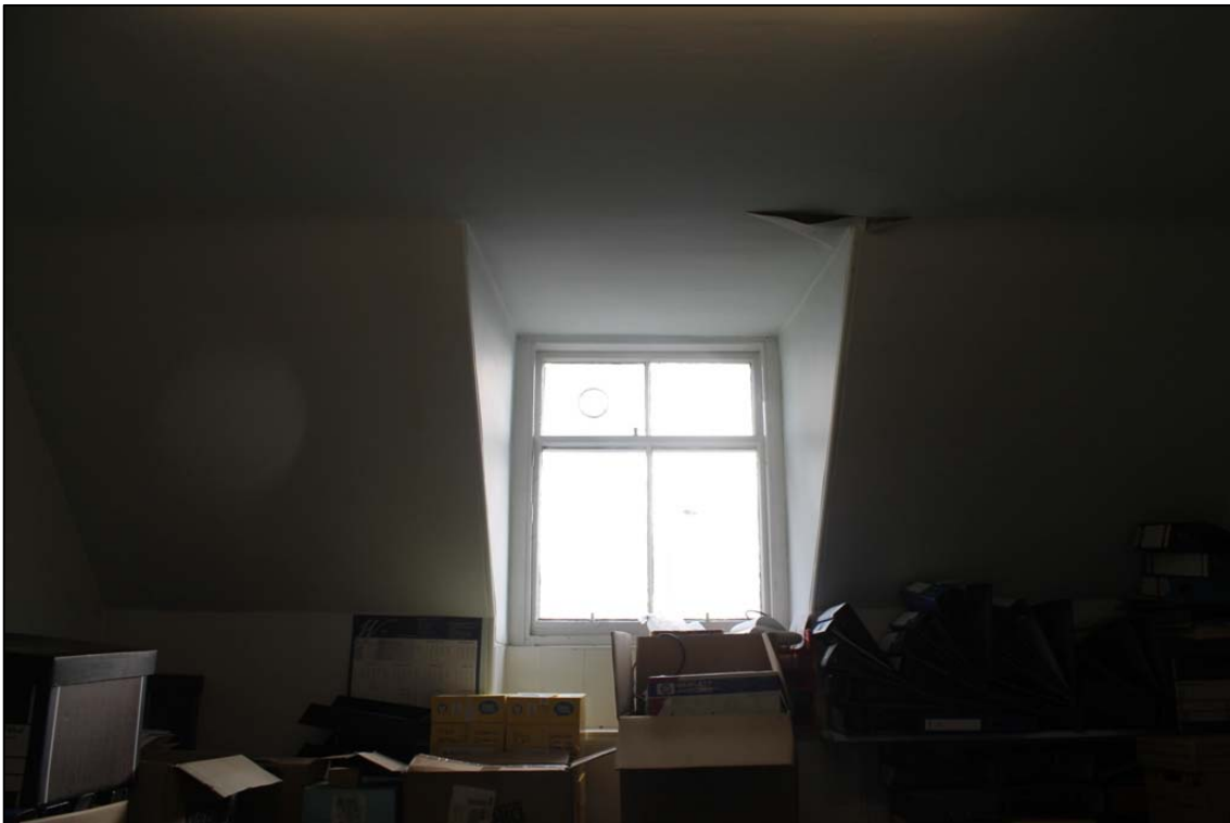
Figure 35b: 1 st floor Room B, S wall and Window B taken from N.
