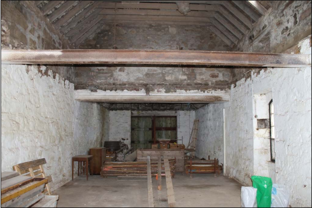
Figure 11a: Room A looking east showing where the extension has been added
