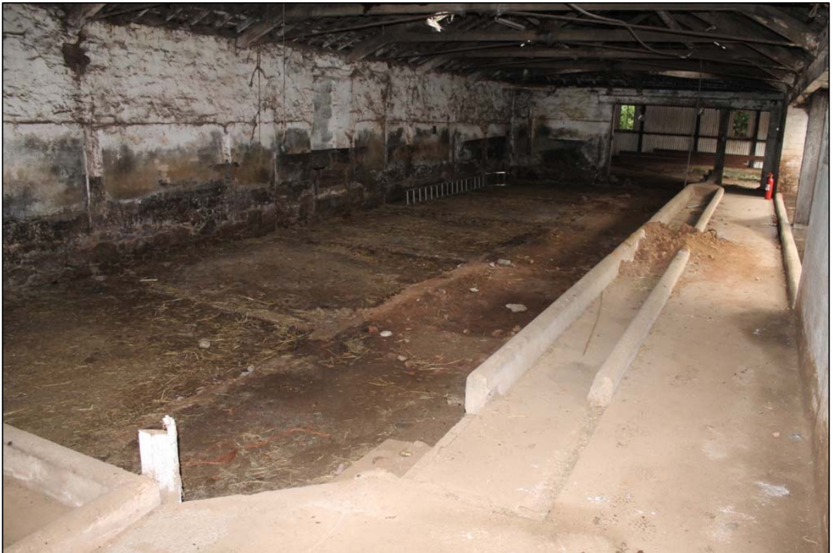
Figure 14b: Room D demonstrating trough III and the remains of the removed animal pens
