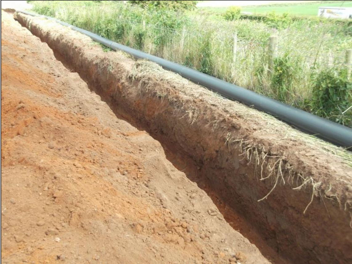
Figure 3b: Shot of pipe trench in northern section in Area 1 from the southwest
