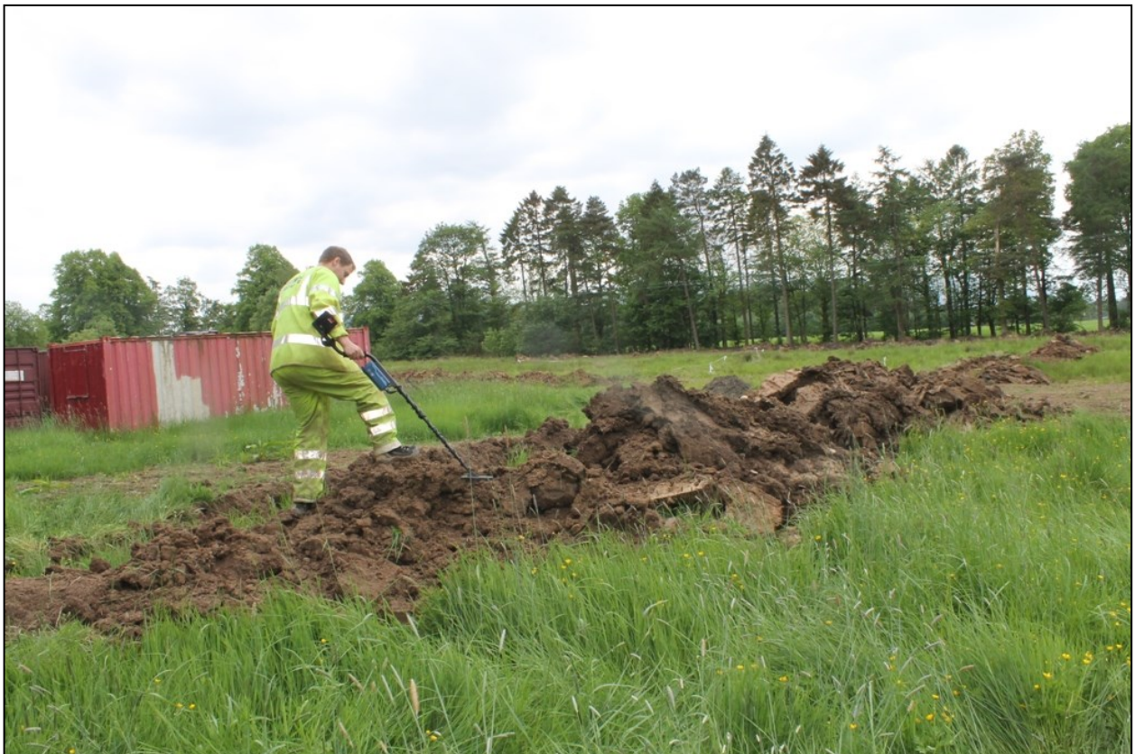
Figure 3b: Metal detecting spoil from trenches located in areas of reasonable potential.
