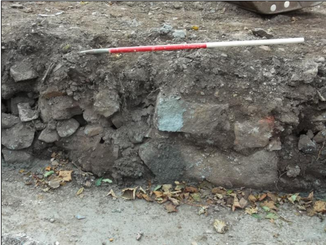
Figure 7a: Wall footing (111), abutting stony layer (112) in NNW-facing section of Trench b/g
