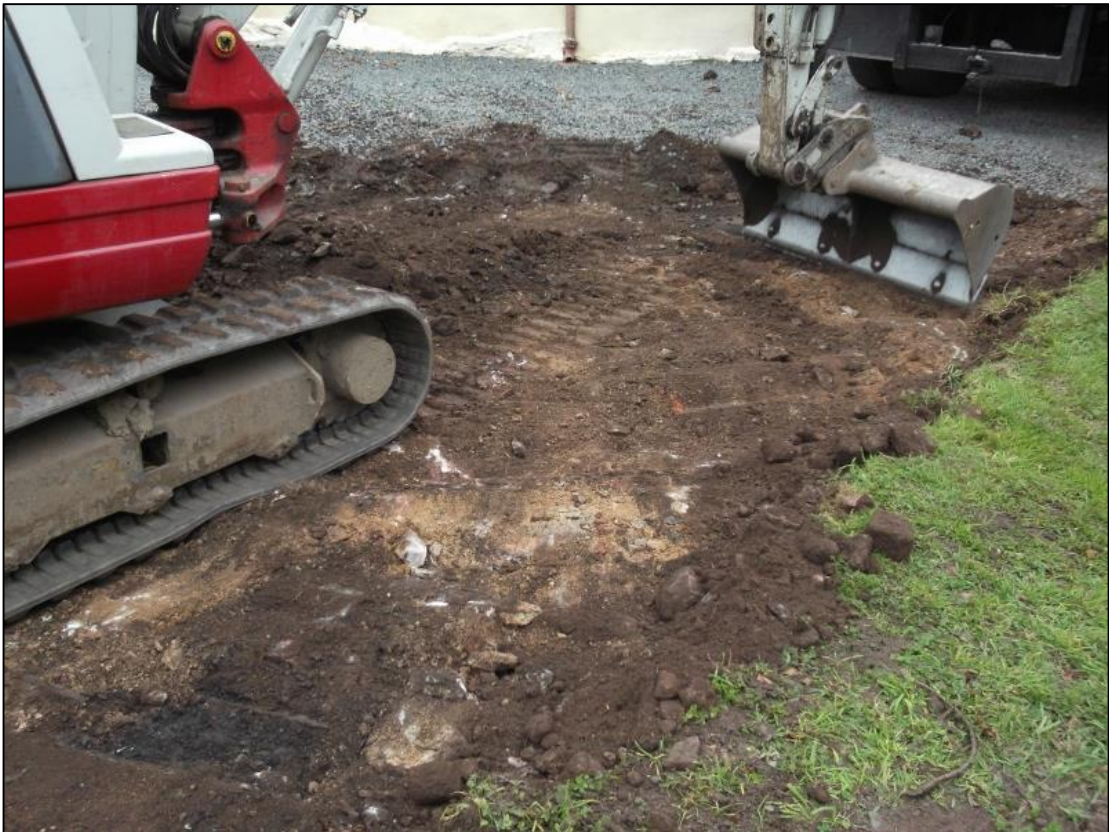
Figure 5b: Demolition layer (105) still in situ at end of ground reduction works
