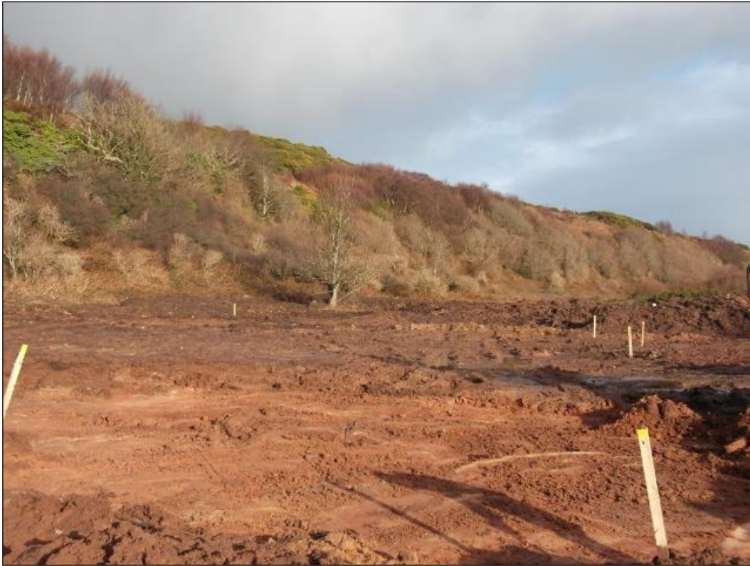
Figure 4a: Post Excavation view of building 3 and surrounding area. From the SW
