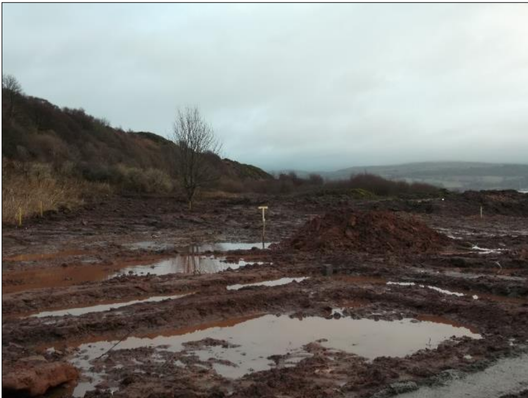
Figure 3b: Post excavation view of building 2 with the carpark area in the background. From the SW
