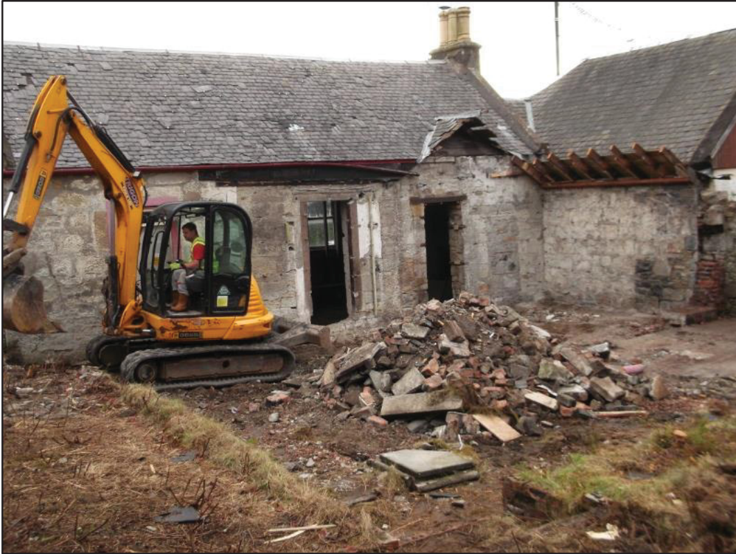
Figure 3a: Pre-excitation view from W, showing SW end of extant mid-19 th century cottage and upstanding SE wall of outshot
