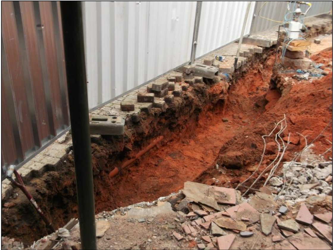
Figure 6: View of the western part of the outer foundation trench from the SSE.
