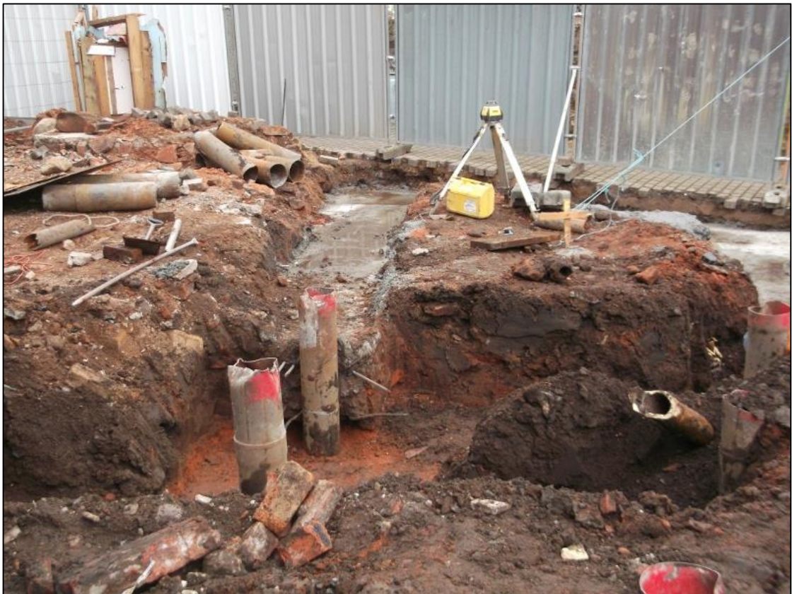
Figure 7: View of the internal foundation in the northern part of the development area from the E.
