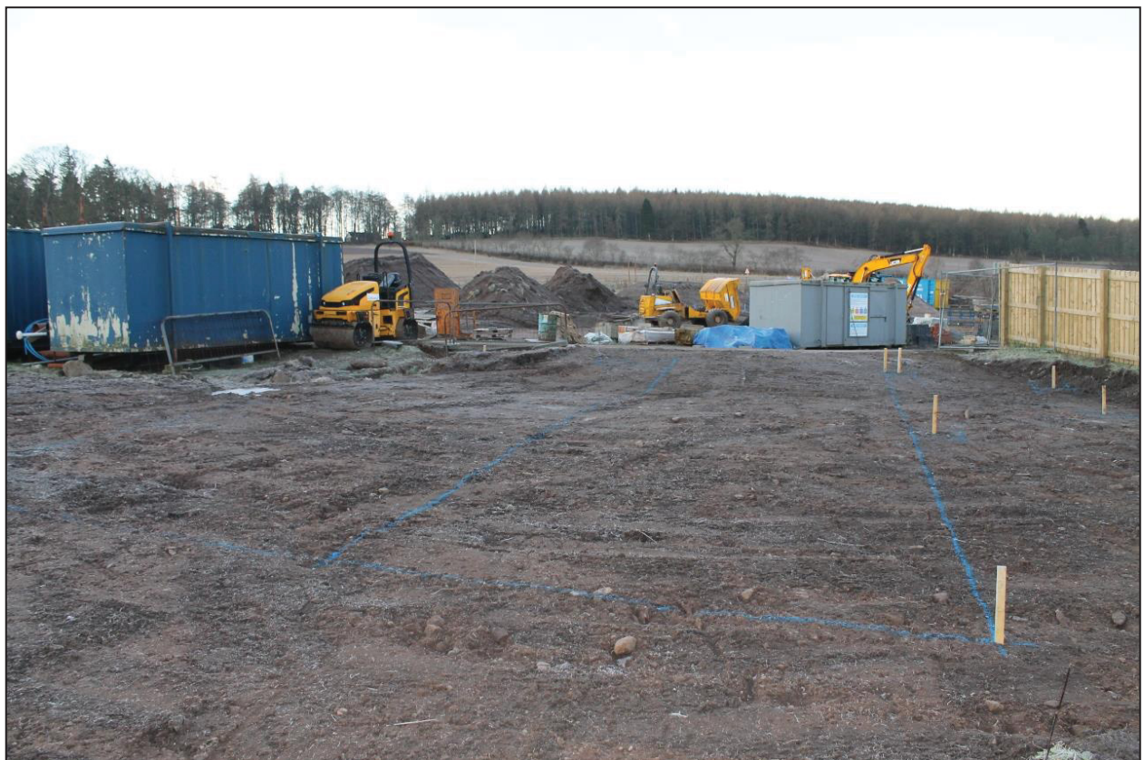
Figure 4b: Demonstrating the northeast area of the site that had topsoil removed prior to the evaluation works commencing
