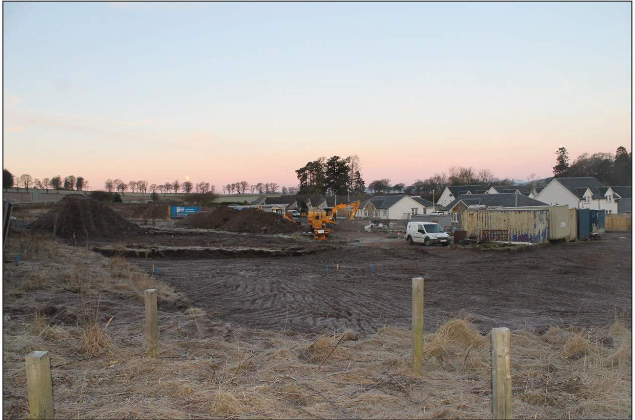
Figure 4a: Demonstrating the east and southeast areas of the site that had topsoil removed prior to the evaluation works commencing and the slight south-north slope
