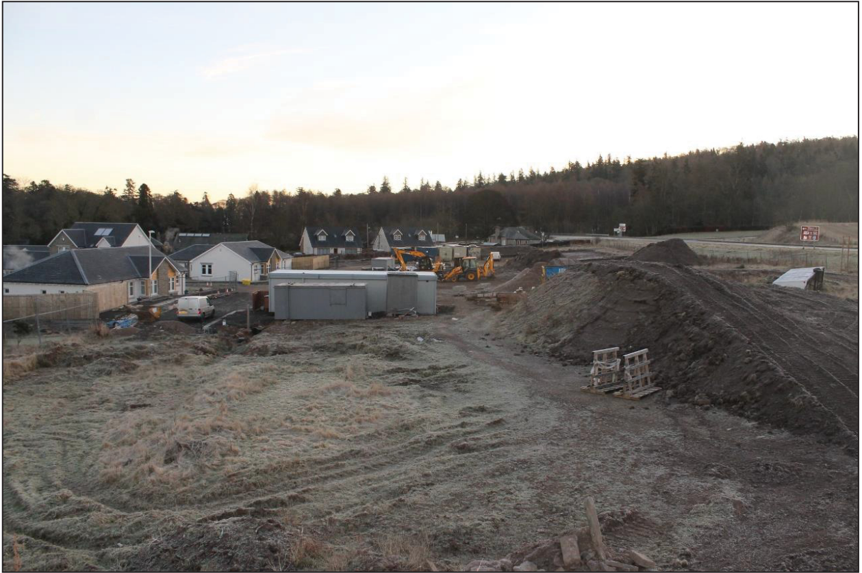
Figure 3a: View to the east demonstrating welfare/storage cabins and previously disturbed areas and soil bunds
