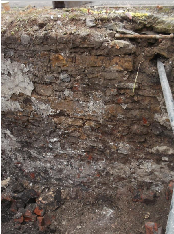
Figure 3b: The SSE wall of the cellar [004] and concrete floor (005). From the NNW.
