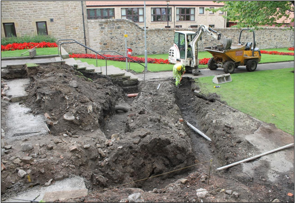
Figure 8a: Showing the lower northern area of the ramp and foundation trenches
