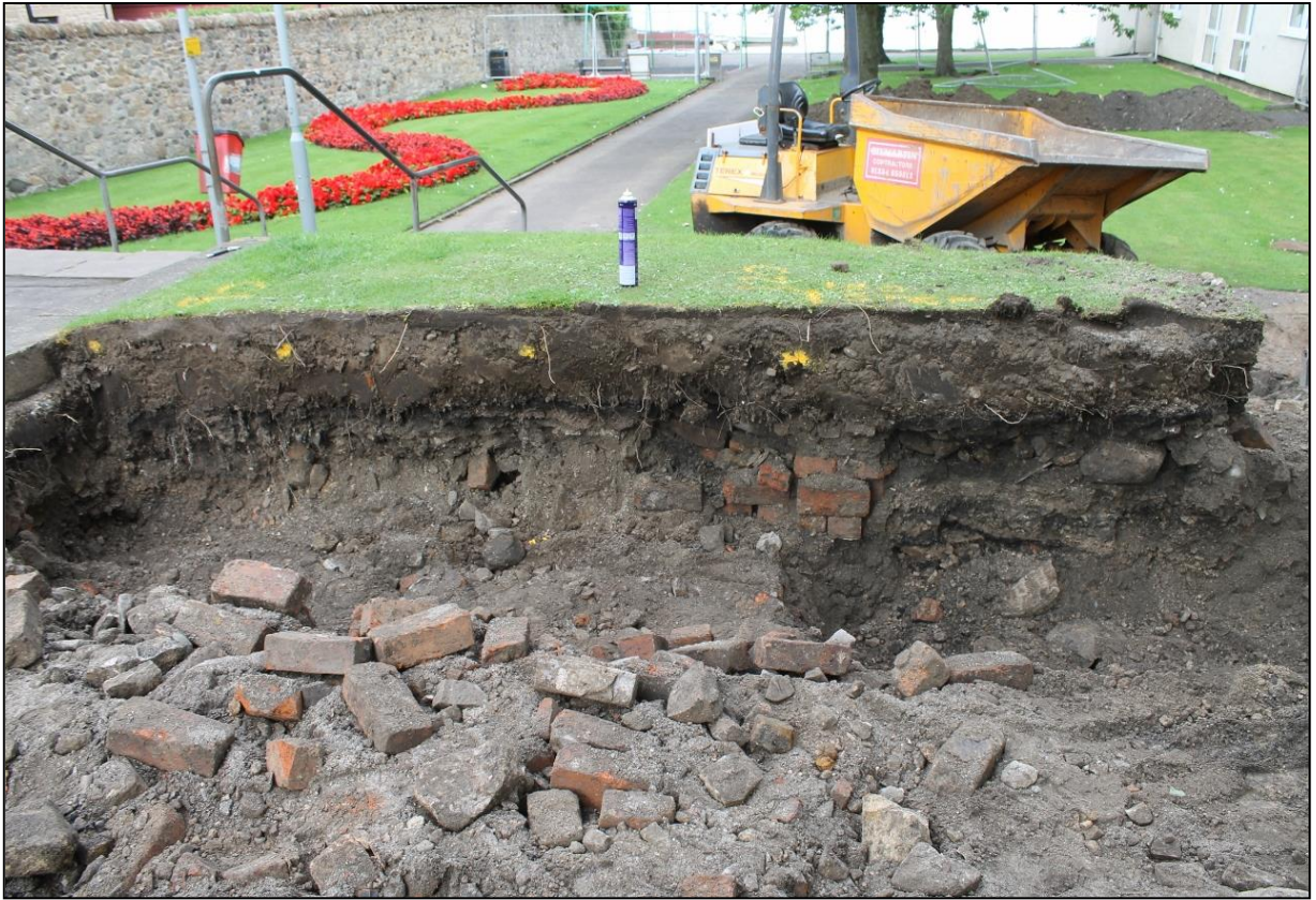
Figure 6a: South facing section in the upper southern area of the ramp
