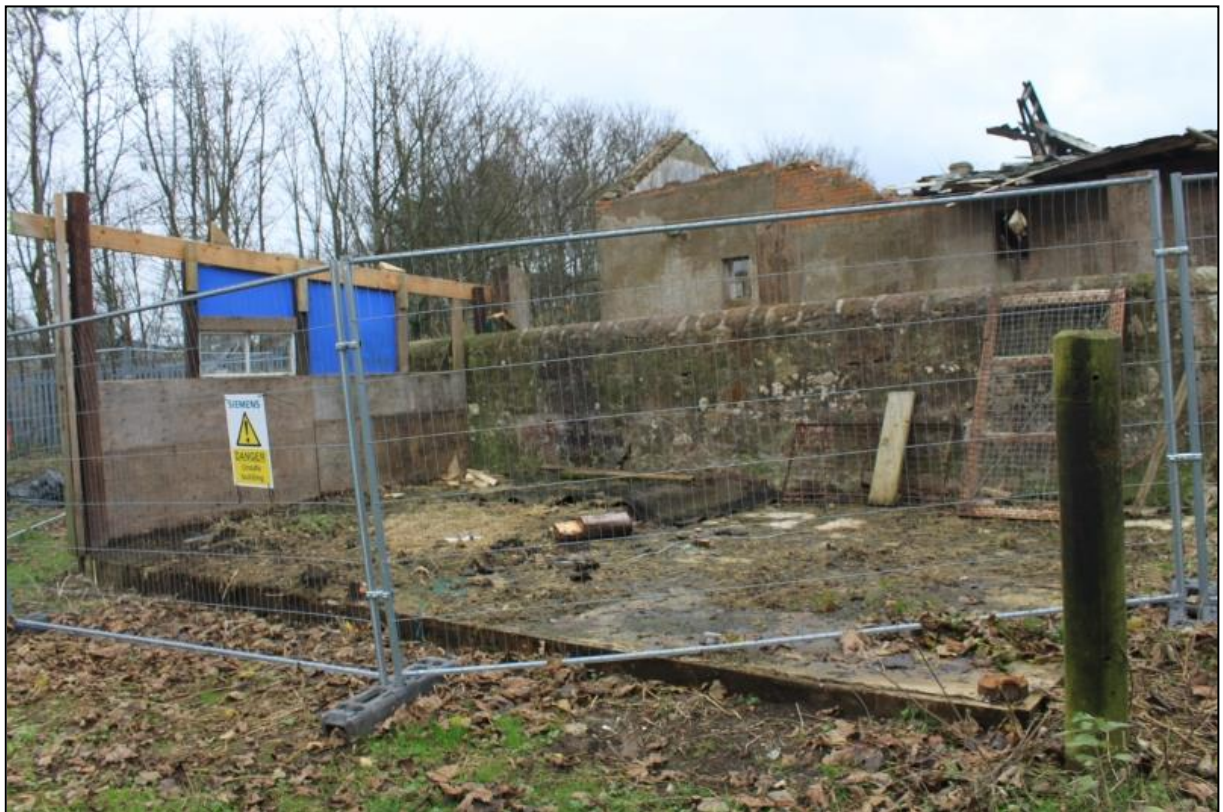
Figure 7b: Remains of structure 'h', comprising concrete apron and one upstanding stud wall (unnamed wall forming external courtyard to rear)
