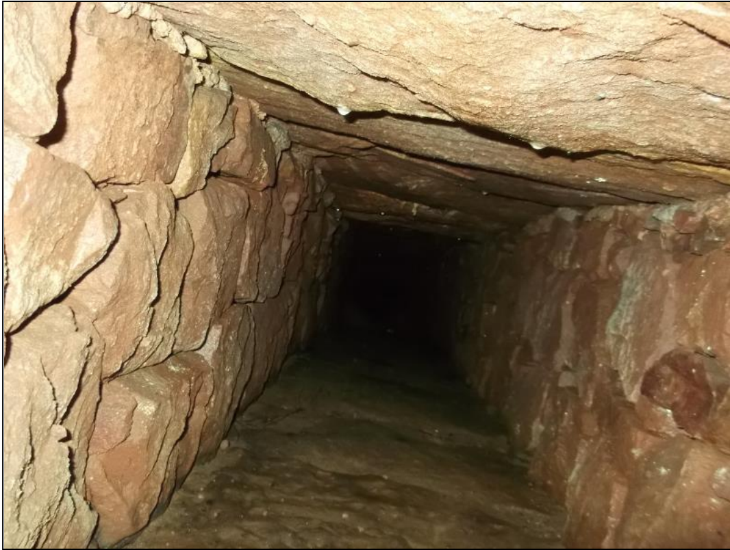
Figure 11a: View looking NNW along interior of culvert [511], with capstones [510] above and supporting walling [509] to either side
