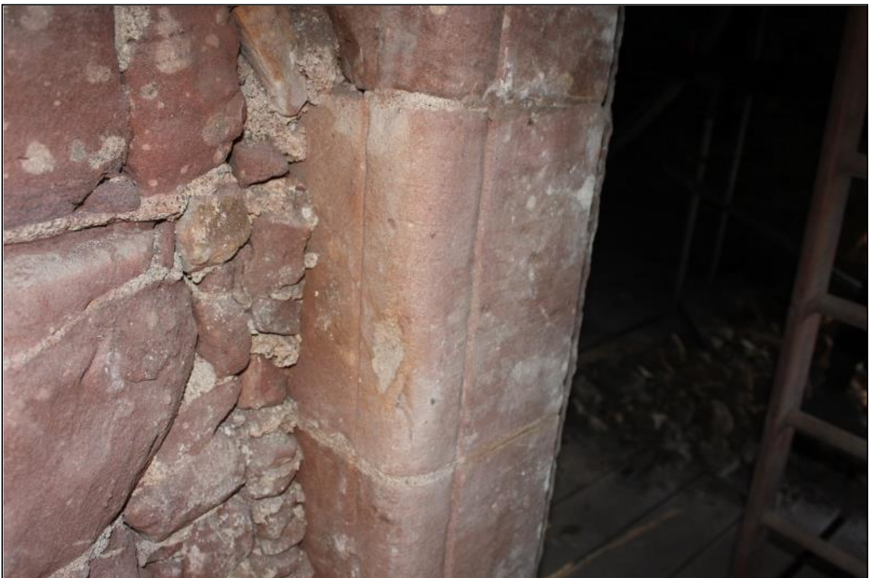
Figure 12b: 1 st floor opening between tower-house and SW stair, showing abutting masonry with no trace of tuskling, and flattened cable-moulding
