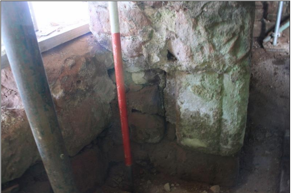
Figure 12a: Ground floor opening, W wall of tower-house, showing straight embrasure and cable-moulding
