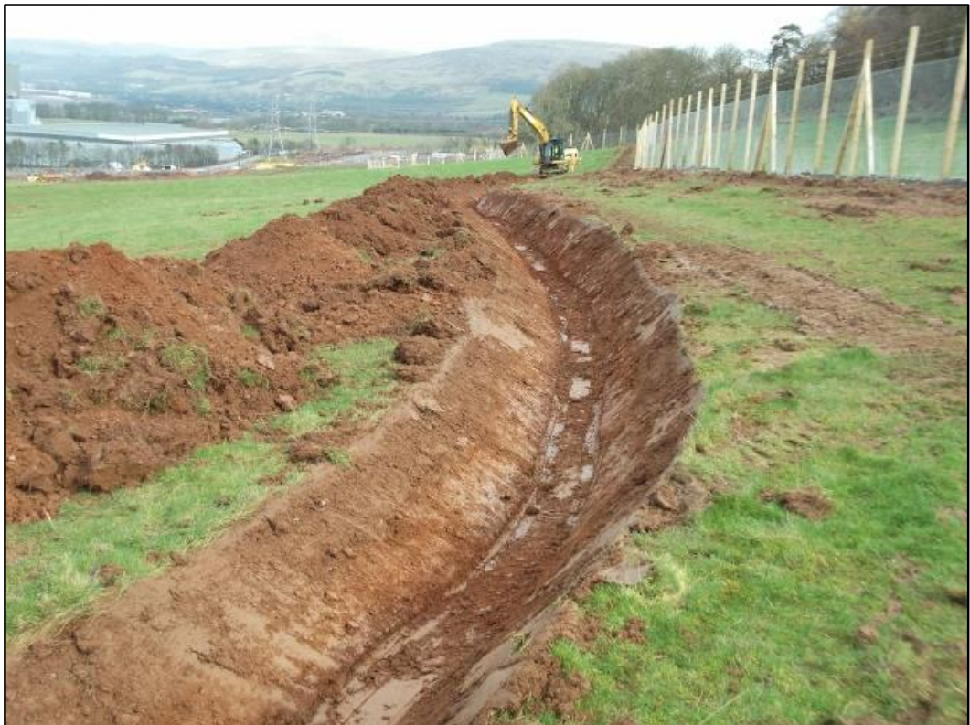
Figure 4b: General shot of drainage ditch, Area 3
