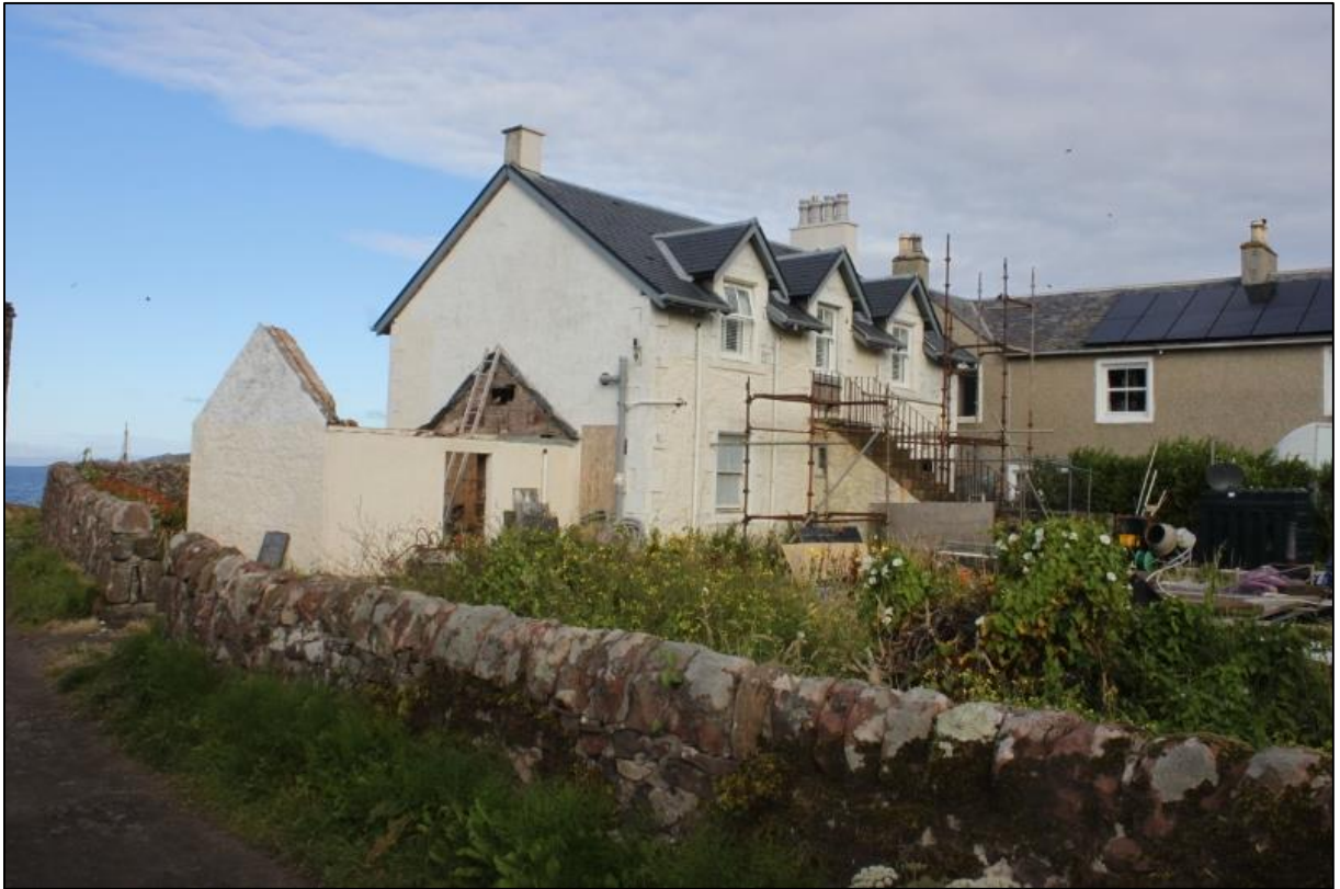
Figure 2a: Looking towards Harbour Cottage from SE, S extension intact prior to demolition
