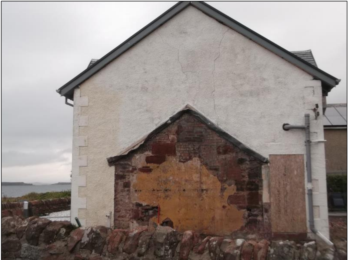
Figure 4b: S elevation of main building following removal of S Extension, with blocked doorway (and threshold step painted red) to right.
