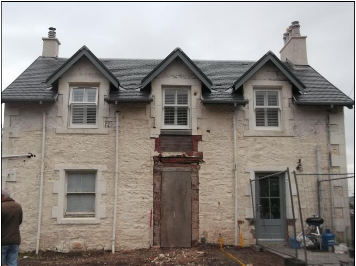
Figure 7b: Rear E elevation of main building following removal of external stair
