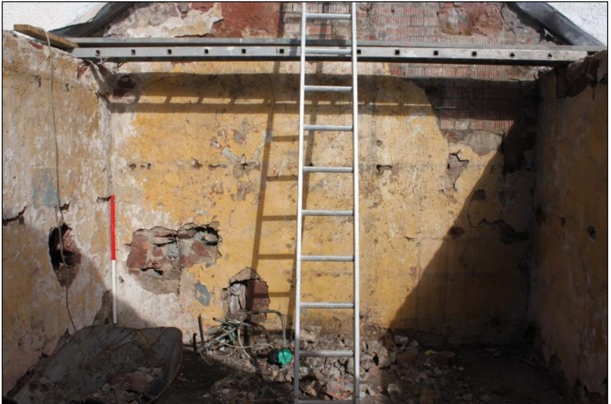
Figure 3b: S Extension ('Room a') – View of N wall from S end
