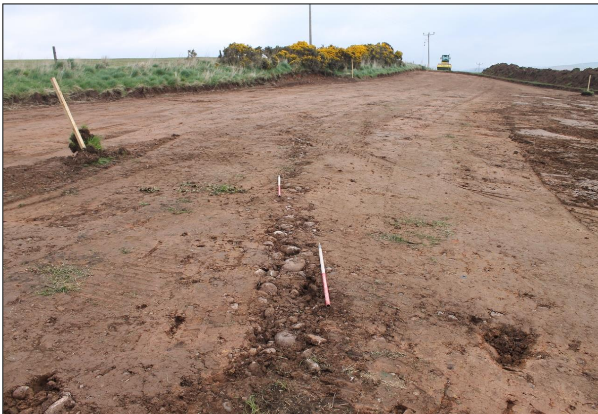
Figure 5a: Feature (003, rubble field drain in located in the north-western area of the turbine area.
