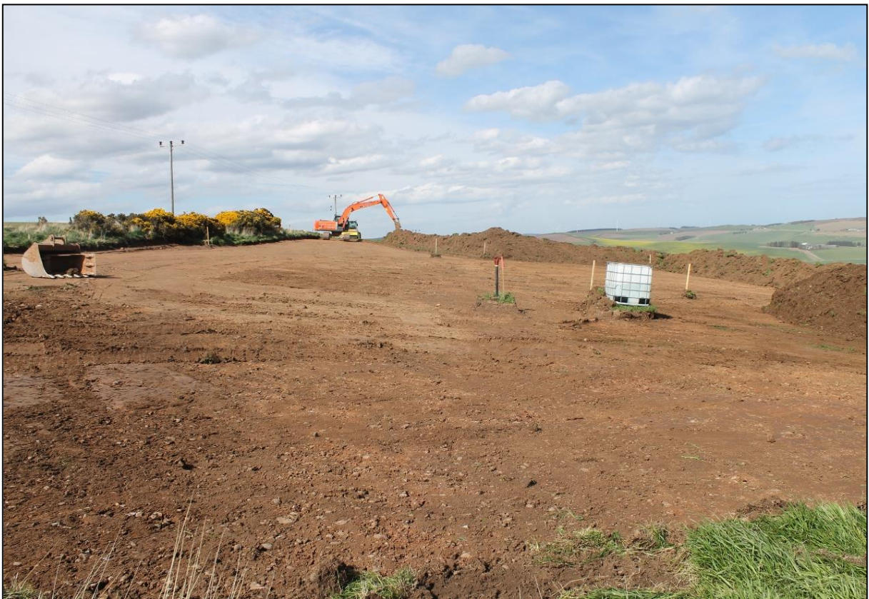
Figure 3b: Turbine storage, crane pad area and turbine area fully excavated. Turbine area located in the foreground of the image. Demonstrating context (002).
