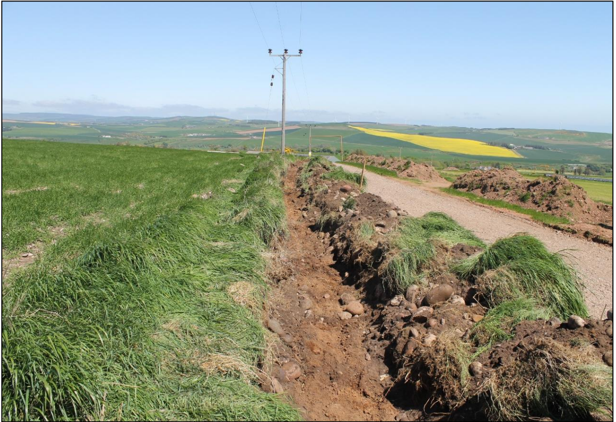
Figure 9a: Cable trench to take the high voltage electricity cable underground looking north.
