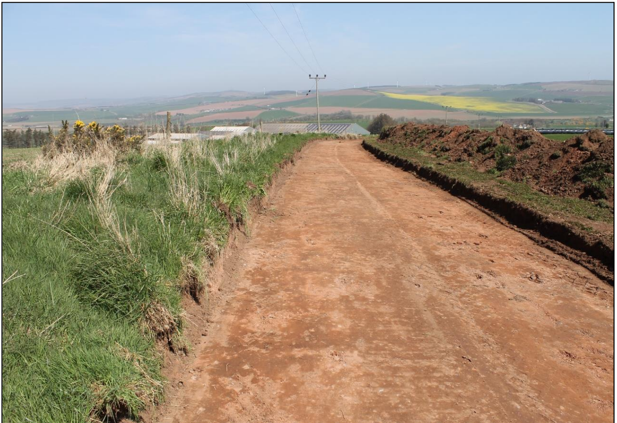
Figure 4b: Upper southern section of haul road and demonstrating context (002) recorded across the excavated areas.
