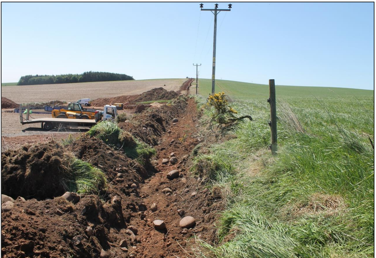
Figure 9b: Cable trench to take the high voltage electricity cable underground looking south.
