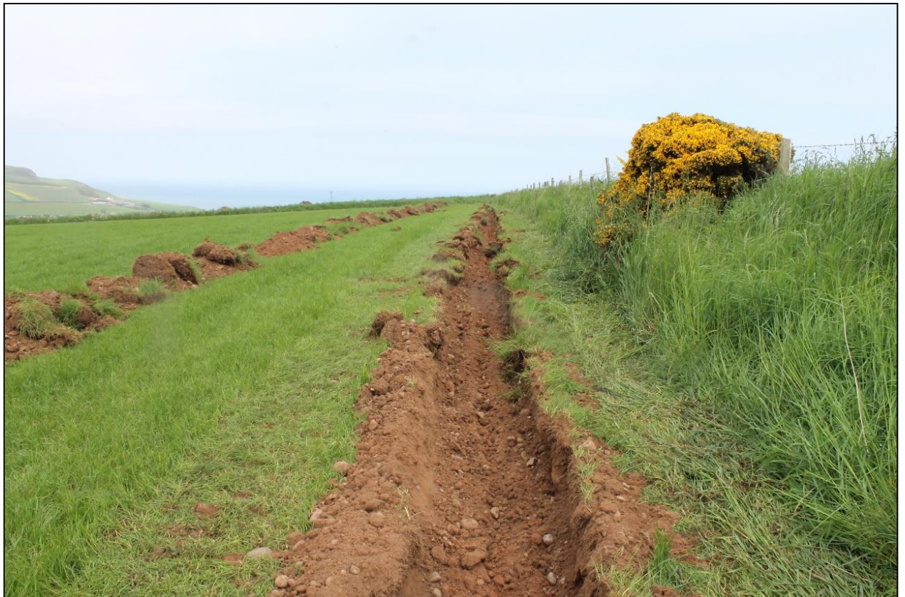
Figure 10b: Topsoil excavated from the lower north-eastern section of the 11kv cable trench.
