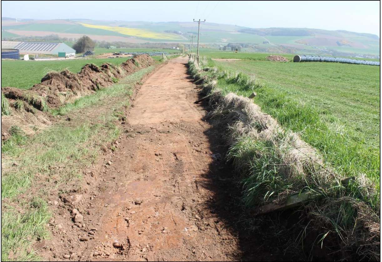
Figure 4a: Lower northern section of haul road and demonstrating context (002) recorded across the excavated areas.
