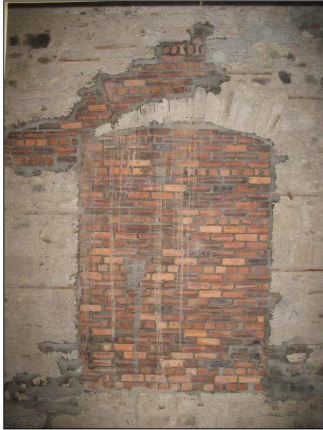
Figure 16a: Bricked up doorway & line of stair, N wall of lift shaft, from Room 221
