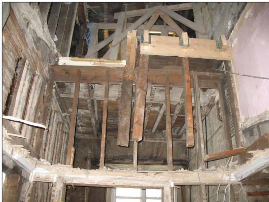
Figure 14b: Room 119 from interior of 113 – site of former stair, with timber flooring still in situ
