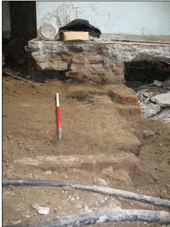
Figure 7b: Line of earlier E-W walling originally forming cross-wall between Room 007 and Corridor 005
