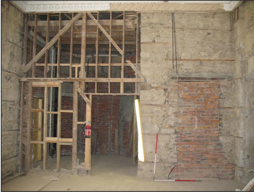
Figure 11a: Room 106 – View from Room 102, showing Masonry Cross-wall (to right) and frame of timber stud wall (to left)
