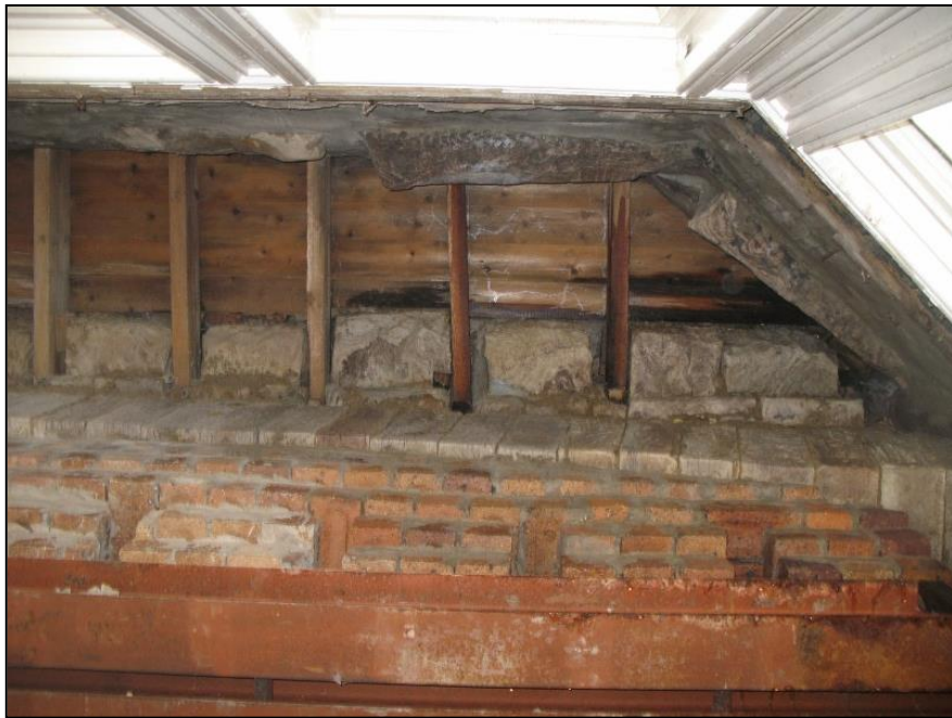
Figure 13b: Reinforcement of main bay window, Room 103, seen from below, showing (bottom to top – steel beams, brick superstructure, original segmental arch lintel, and joists/flooring of 2 nd floor
