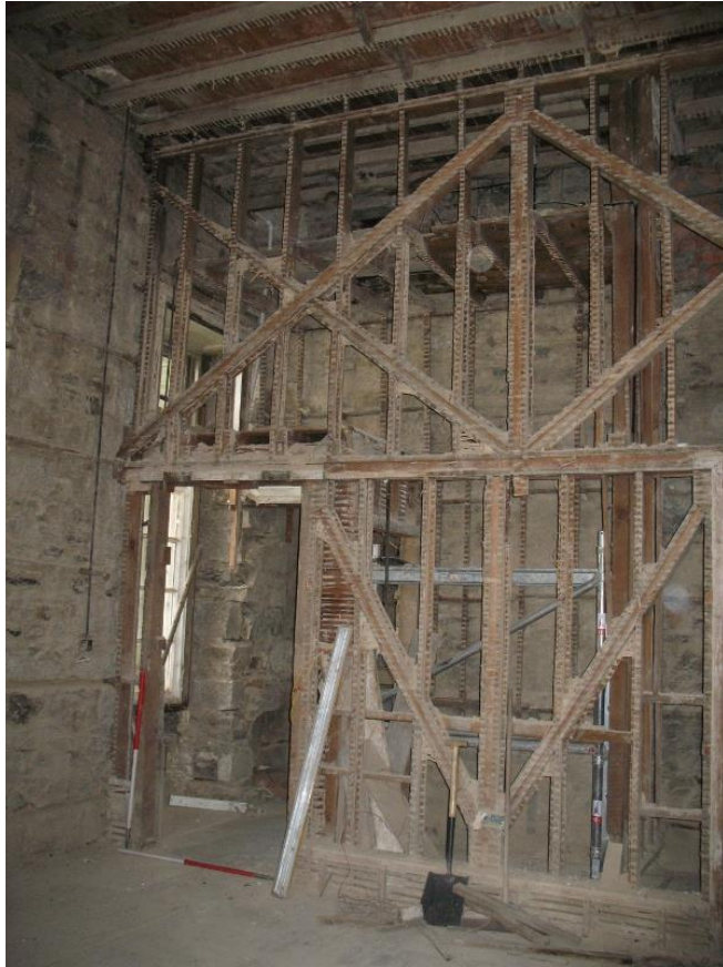
Figure 14a: Room 119 from interior of 111 – site of former stair, with timber flooring still in situ
