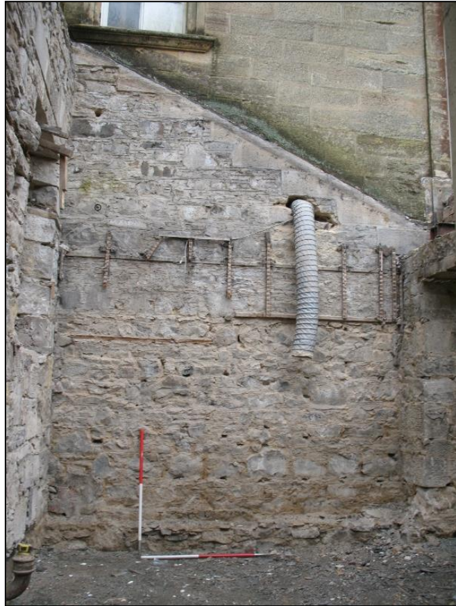
Figure 9a: S Wall of 031, showing shared wall with main house and raggle
