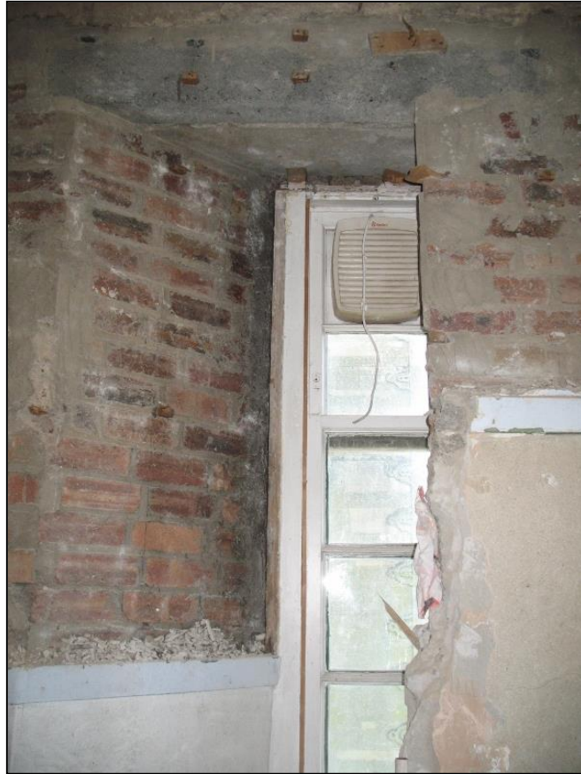
Figure 18a: Splayed window embrasure created through insertion of later brickwork, N wall, Room 216
