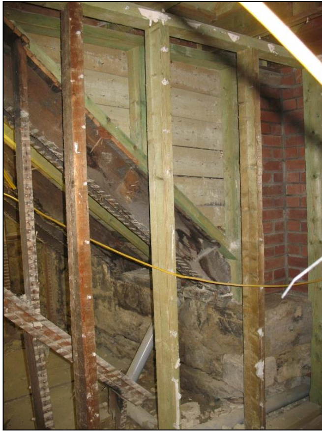
Figure 21a: Looking SW towards junction between original wallhead and modern external access stair, with in situ original timber to left of modern examples
