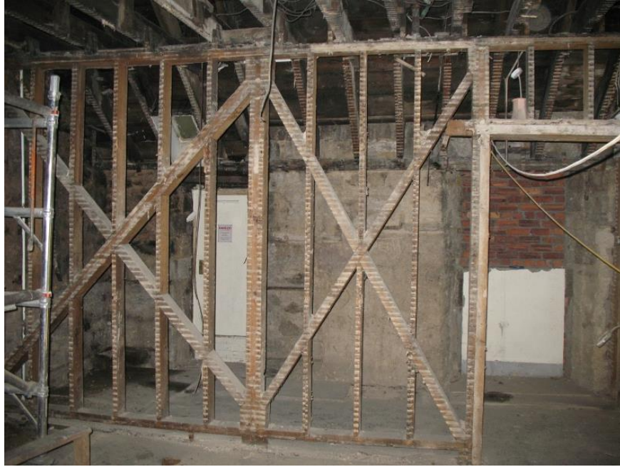
Figure 20a: E wall of Corridor Extension 311 – inserted doorway to left, original doorway to right
