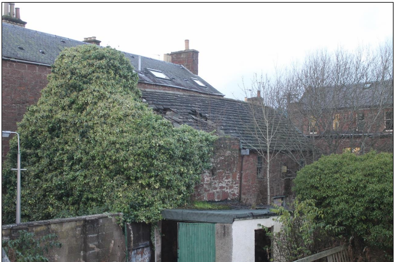
Figure 8b: East and south (ivy covered) elevation of the 'Warehouse' structure to the northwest of the development area
