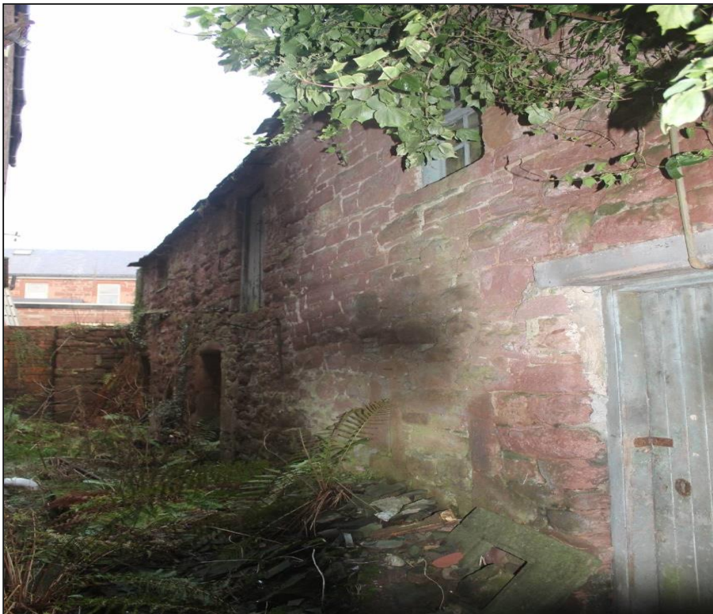
Figure 9b: West elevation of the 'Warehouse' structure to the northwest of the development area
