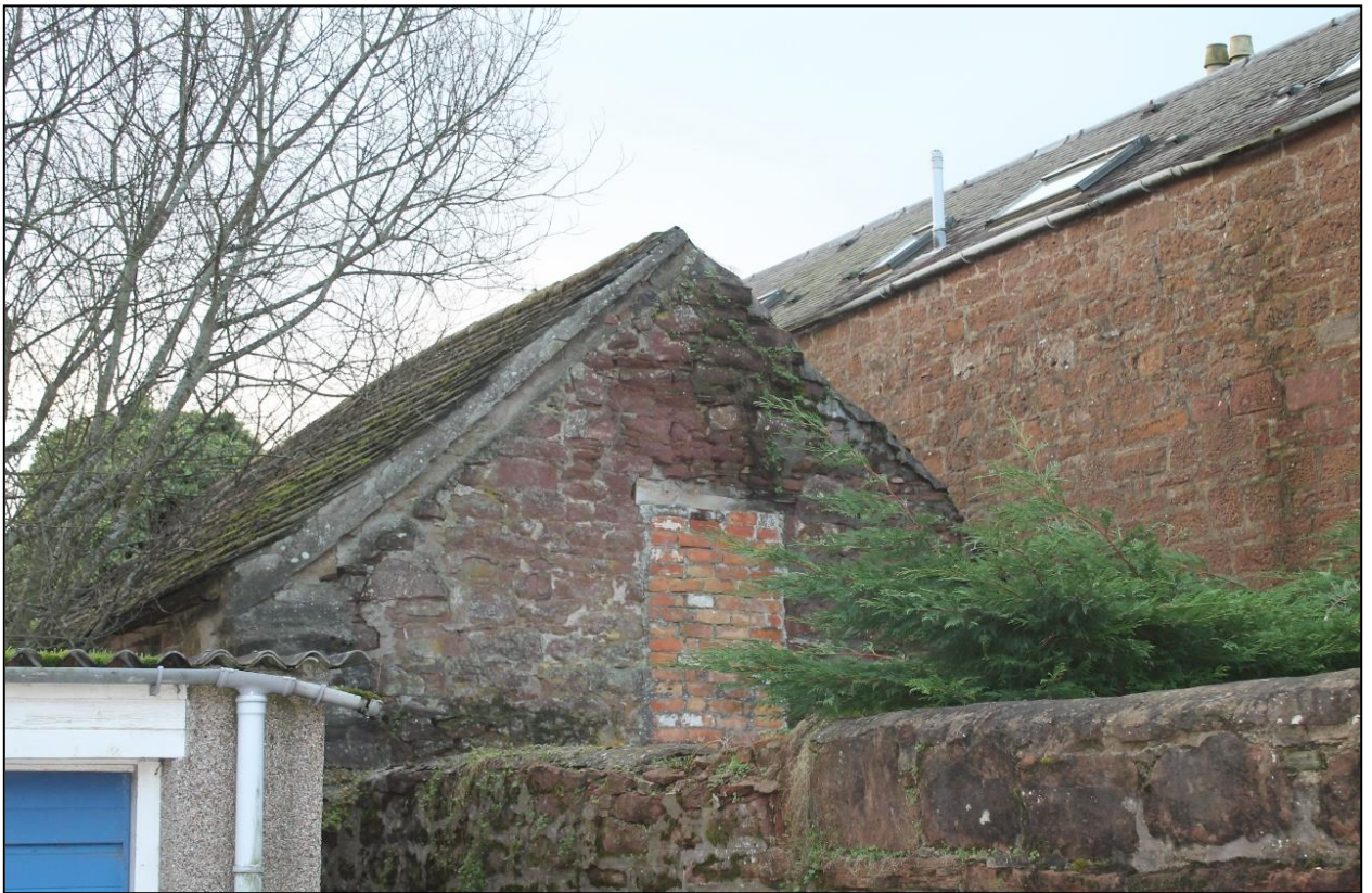
Figure 9a: North elevation of the 'Warehouse' structure to the northwest of the development area
