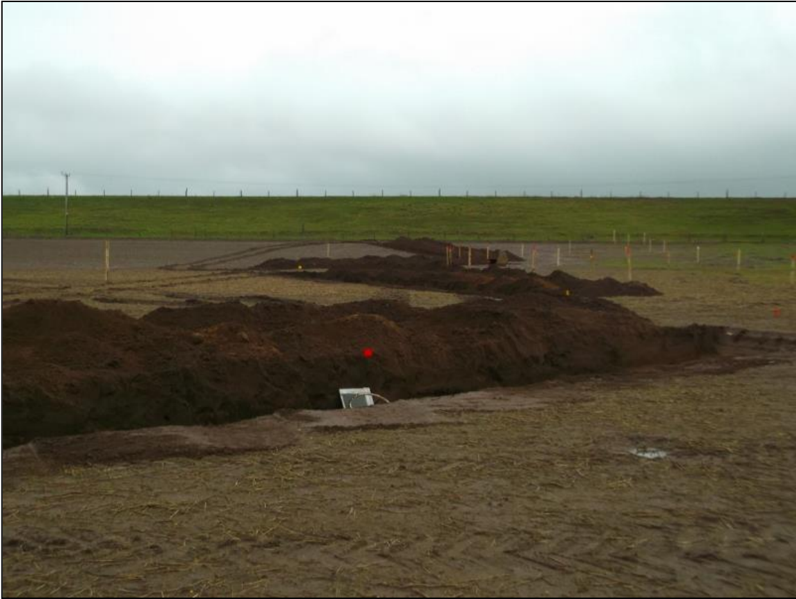
Figure 4: General shot of site from the west, showing the ground sloping up to the east
