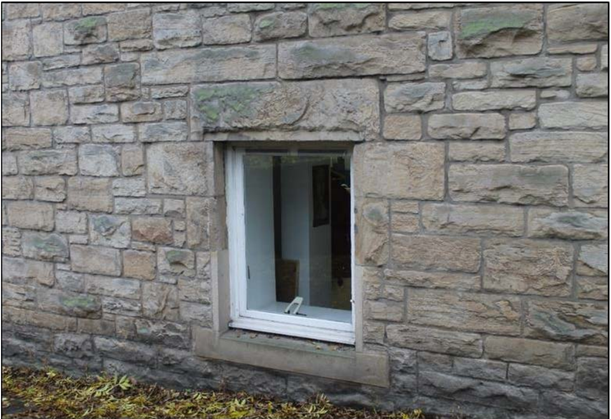
Figure 11b: Window on the north elevation showing historic and modern stonework of garage/office building.
