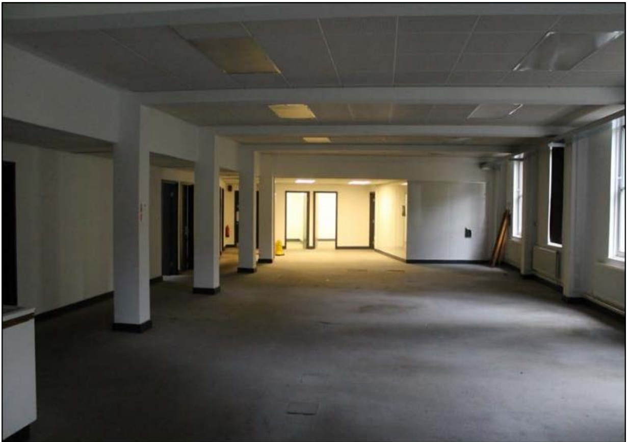
Figure 5b: Basement floor open planned office space and showing the rooms along the south side and at the far northwest side.
