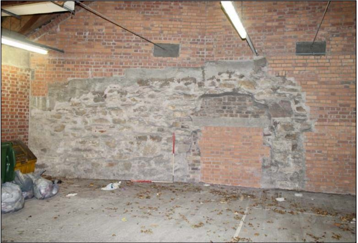
Figure 9a: Historic structural elements on the southwest wall of the interior of the garage area.
