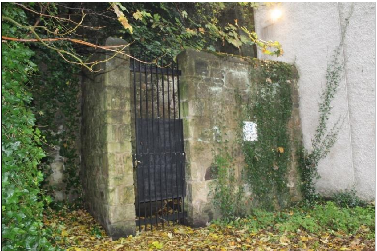
Figure 13b: Fire escape at east end of No.10, historic stonework marking E end of historic structure.
