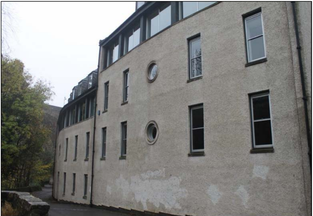
Figure 4b: West end of No.10 Bell's Brae, note brick basal courses under render.
