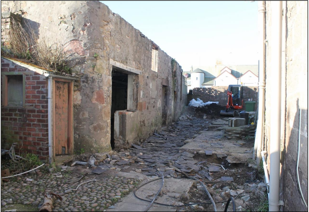
Figure 6a: Demonstrating the area where paving slabs have been removed for the excavation of the service trench
