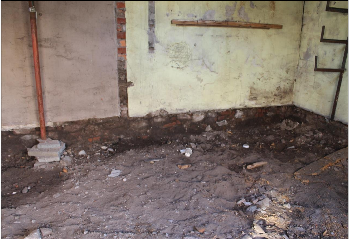
Figure 5a: Demonstrating the depth of removed material from the interior of the redundant store
