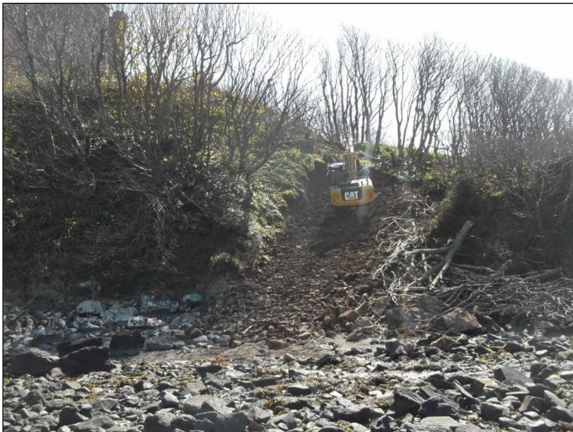
Figure 2b: Machine stripping the access road up the slope, from the W
