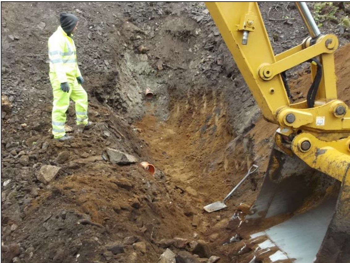
Figure 4b: Deposit (007) exposed in pipe trench at base of the uppermost steep section of the slope before the trench turns to run down the access road
