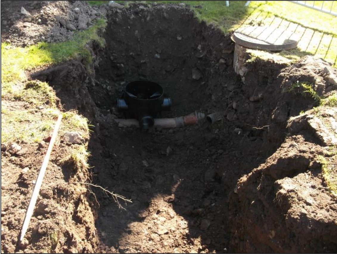
Figure 3a: Pipe trench meeting the septic tank in the garden (with original pipe at the base) showing made ground (003) from the NW
