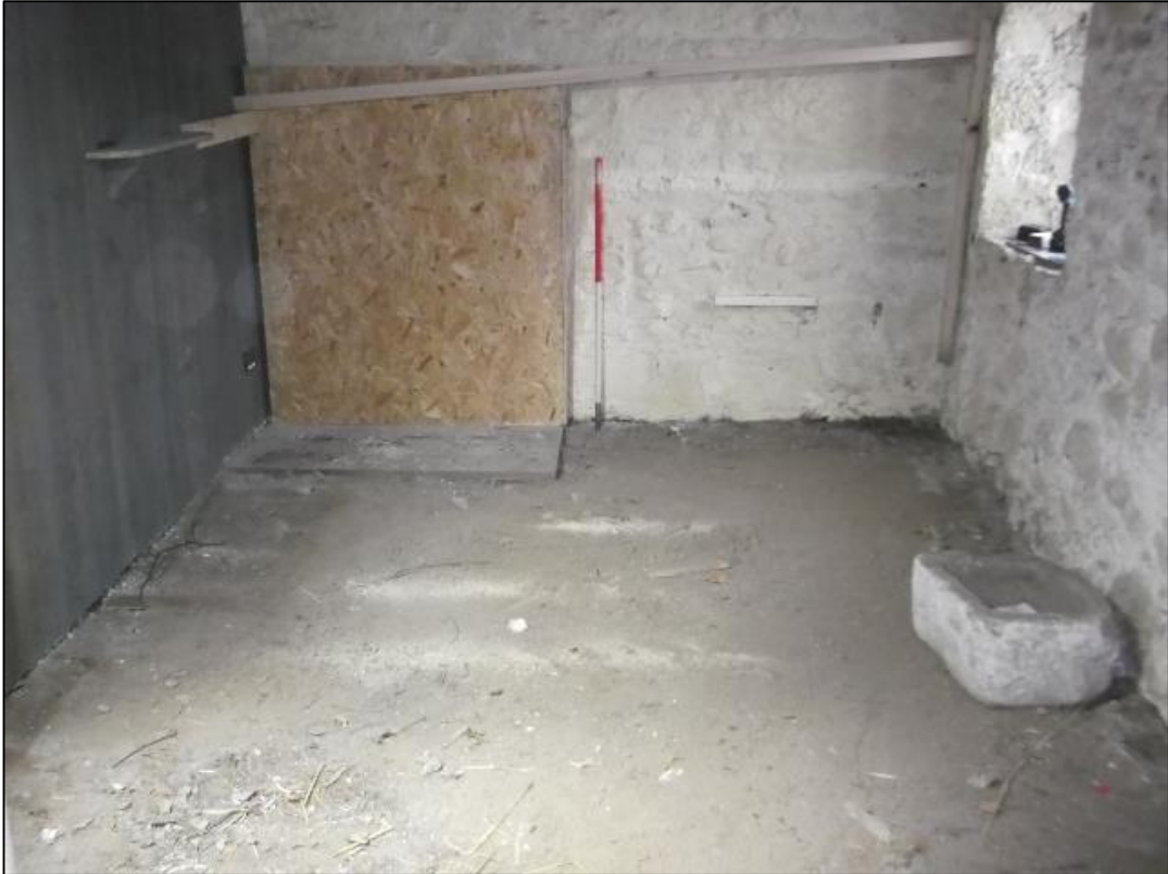
Figure 4a: Pre excavation view of the interior of the cottage from the NNW
