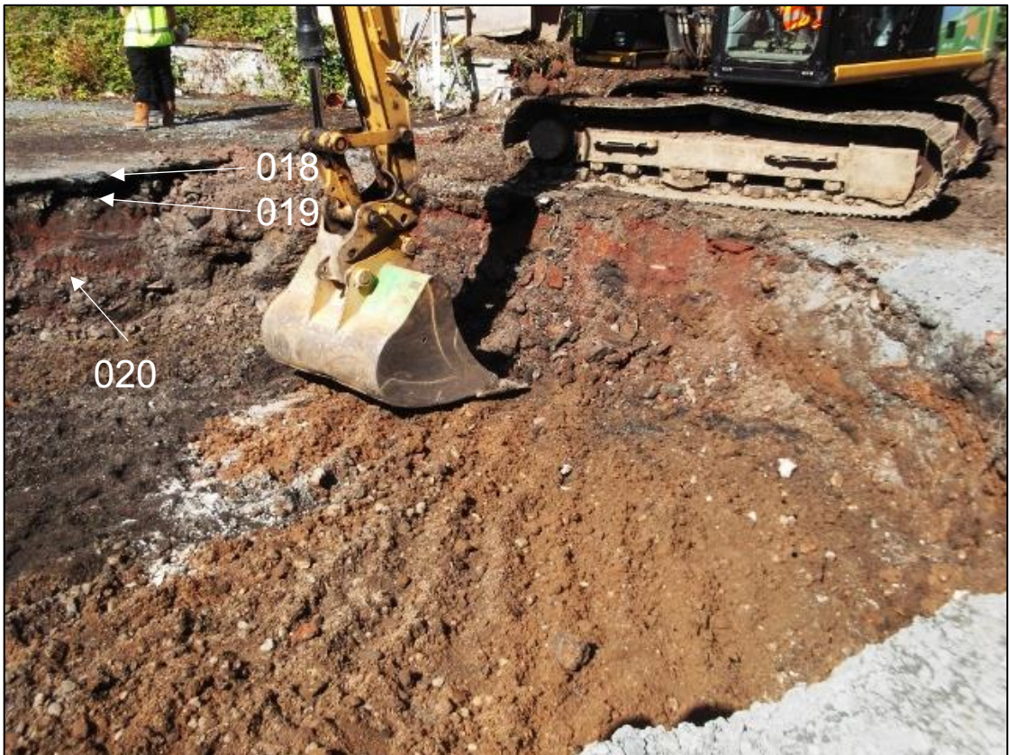
Figure 4b: Post excavation view of Main Manhole Trench showing context numbers. From NNE
