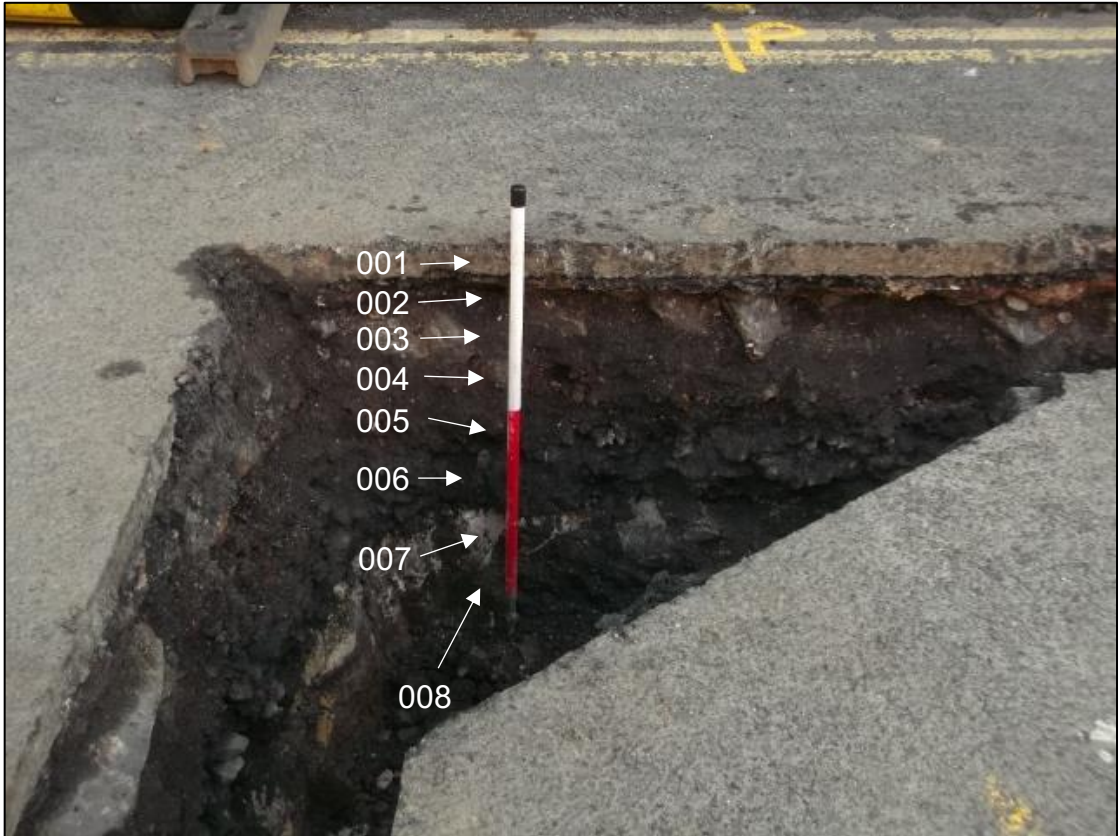
Figure 4a: Post excavation view of Pipe trench showing context numbers. From SSW
