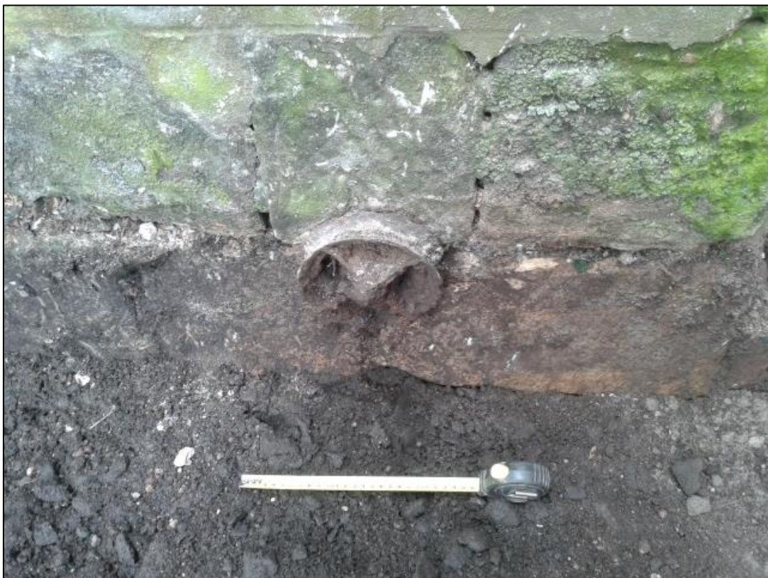
Figure 2b: Close up view of metal cog set into north face of church building.
