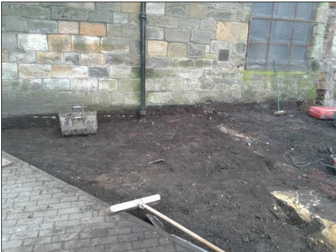
Figure 3b: View of eastern part of area showing disturbed layer (002) from the NE.
