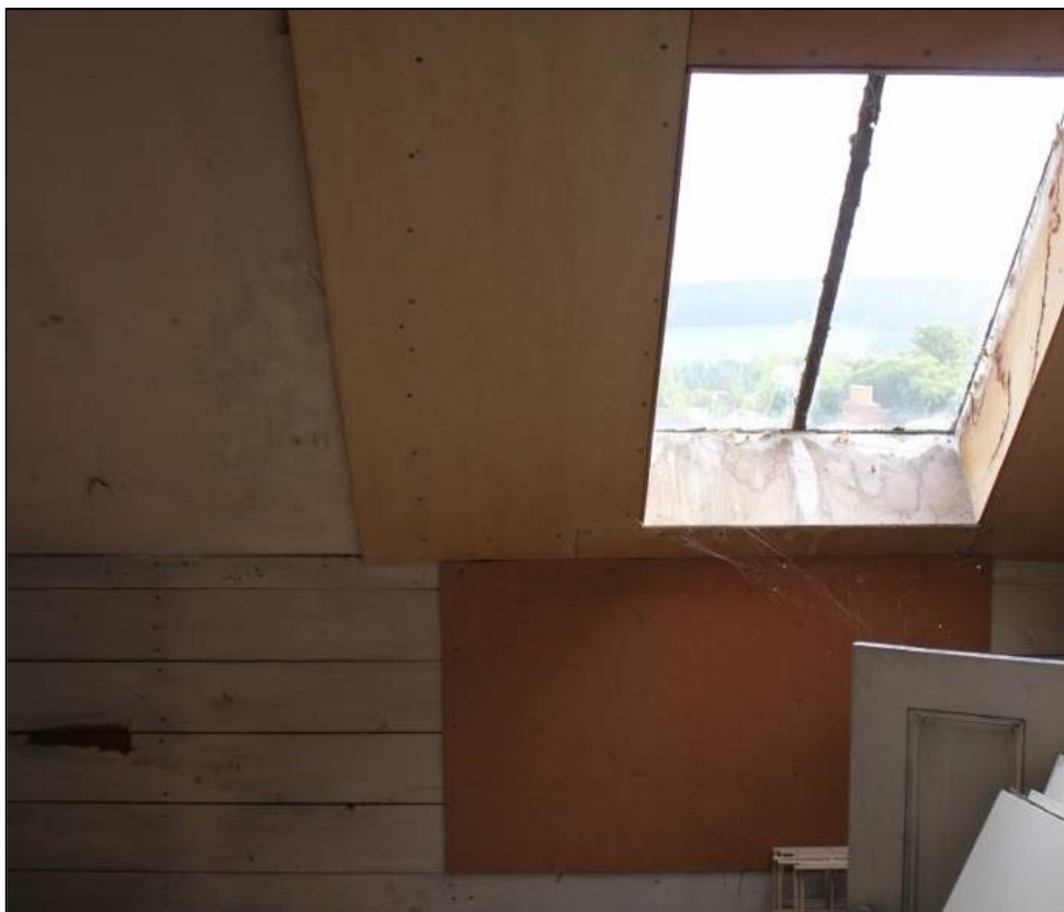
Figure 31b: View of Room 4a, 2 nd Floor, 14-18 Swan St. From the NNW
