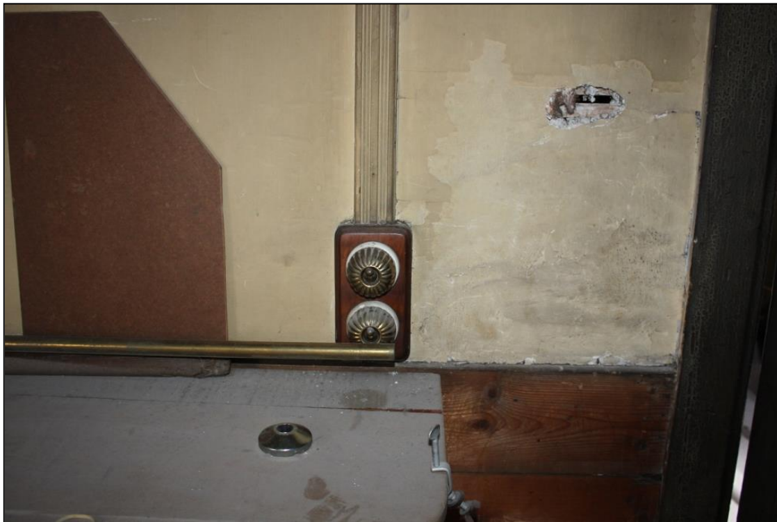
Figure 34b: Light switch W wall, Room 5, 2 nd Floor, 14-18 Swan St. From the WNW
