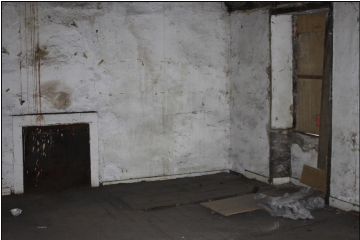
Figure 13b: View of fireplace & blocked floorboards, Room 6, 1 st Floor, 20a Swan St. From WNW
