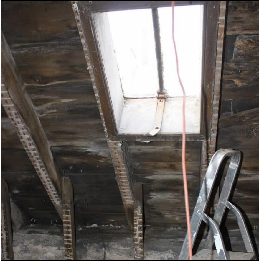
Figure 32a: View of Room 4a, 2 nd Floor, 14-18 Swan St. From the SSE
