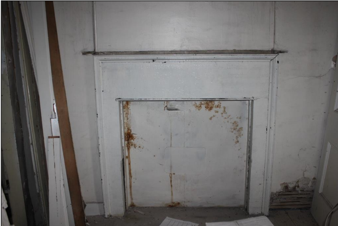
Figure 30a: Fireplace within E wall of Room 3, 1 st Floor, 14-18 Swan St. From the W
