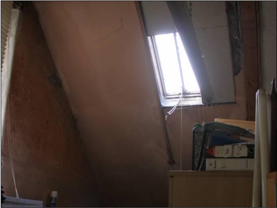
Figure 18a: View of Room 1's skylight, Ground Floor, 20 Swan St. From NE
