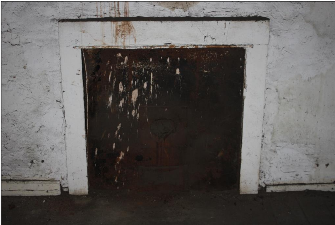
Figure 14b: View of fireplace in WSW facing wall, Room 6, 1 st Floor, 20a Swan St
