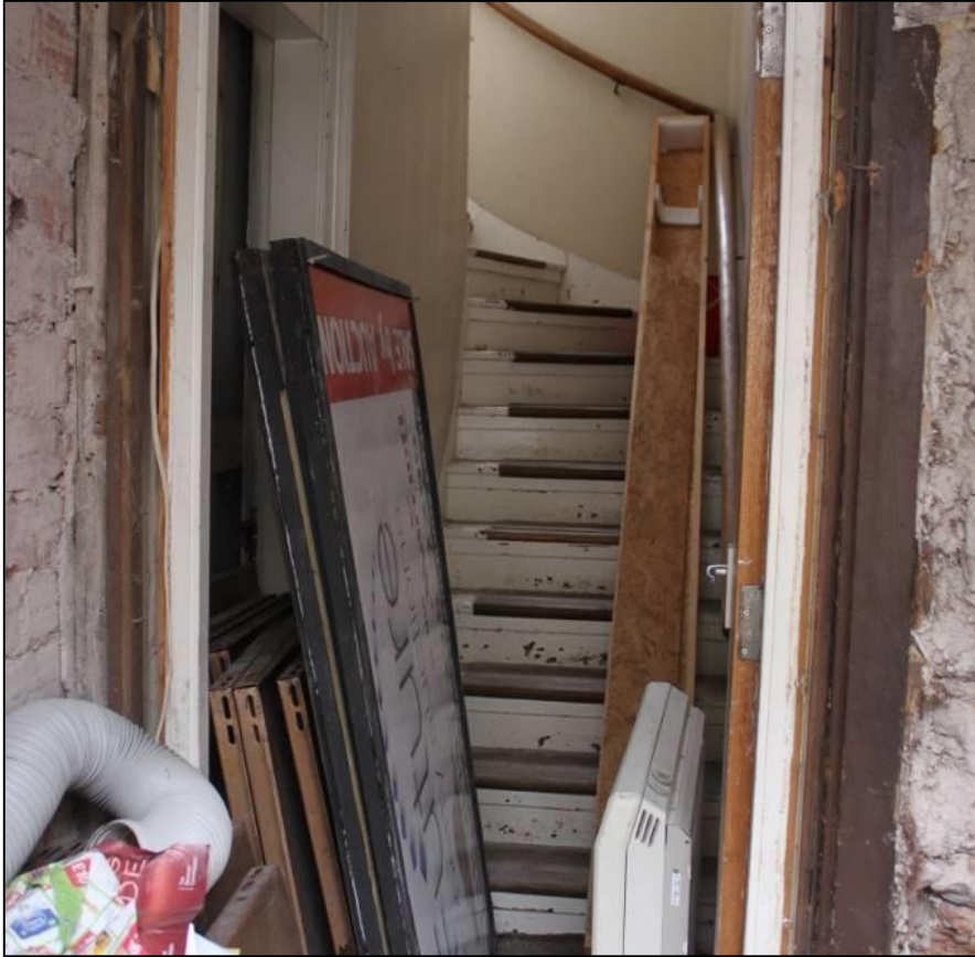
Figure 28a: Stairs to the 1 st Floor from ground level, 14-18 Swan St. From the N
