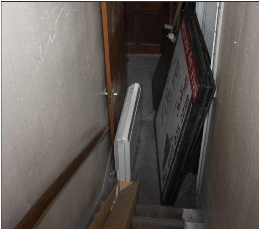
Figure 28b: Staircase from the 1 st Floor to ground level, 14-18 Swan St. From the SSE
