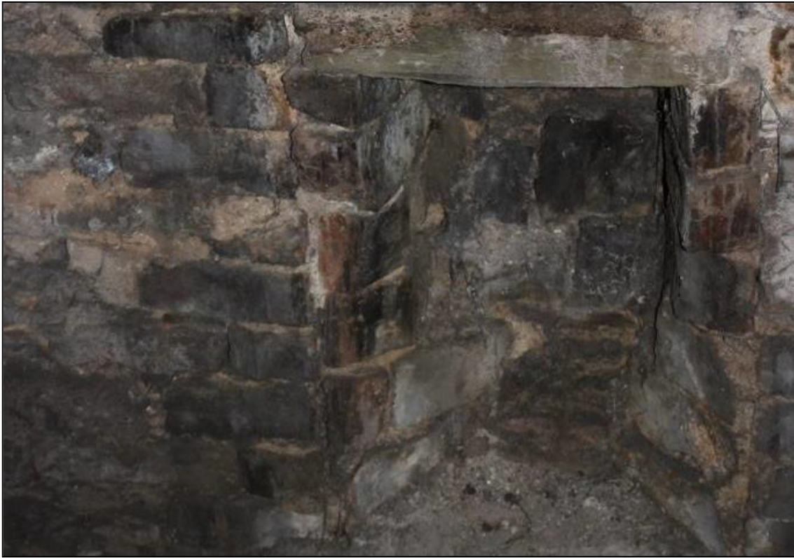
Figure 12a: View of fireplace in NNW facing wall, Room 5, 1 st Floor, 20a Swan St
