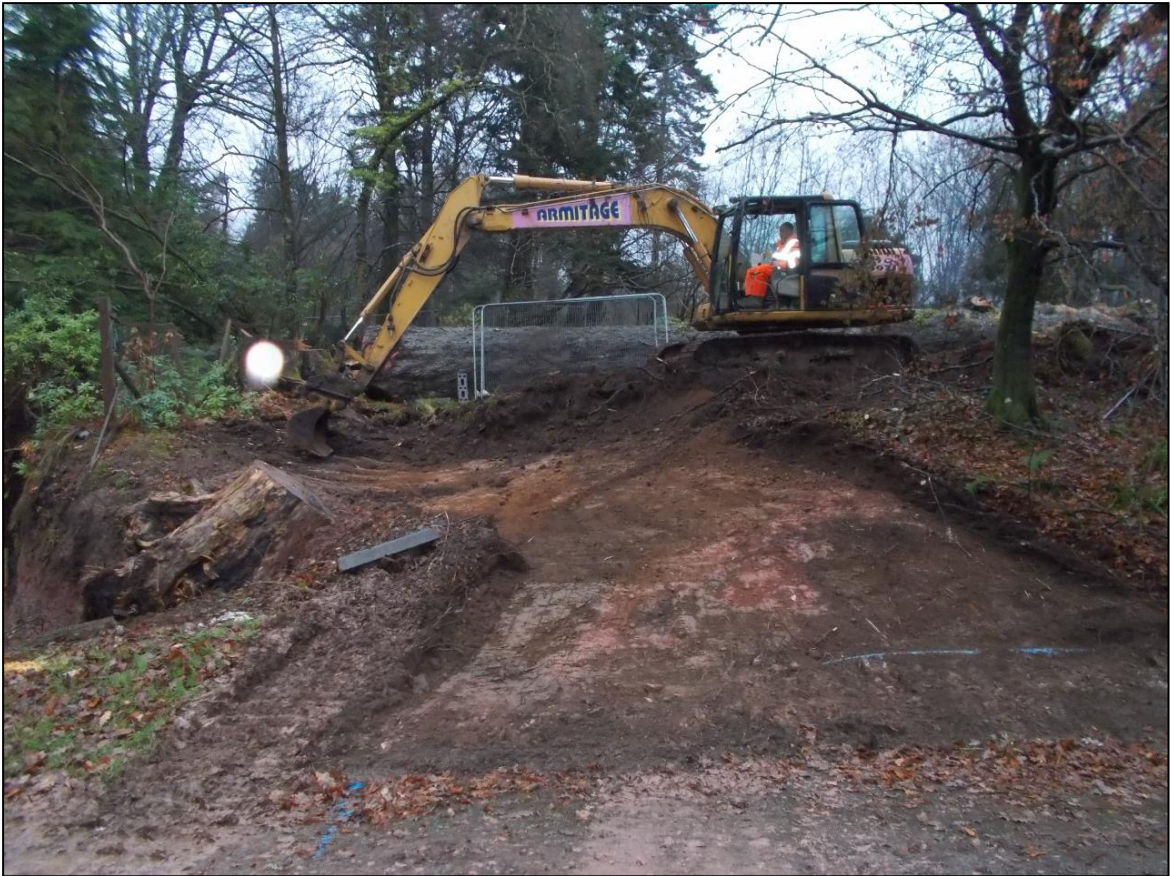
Figure 13: Extension of Area 2 excavated on 15 th December 2016 showing plastic pipe running parallel to the estate road.
