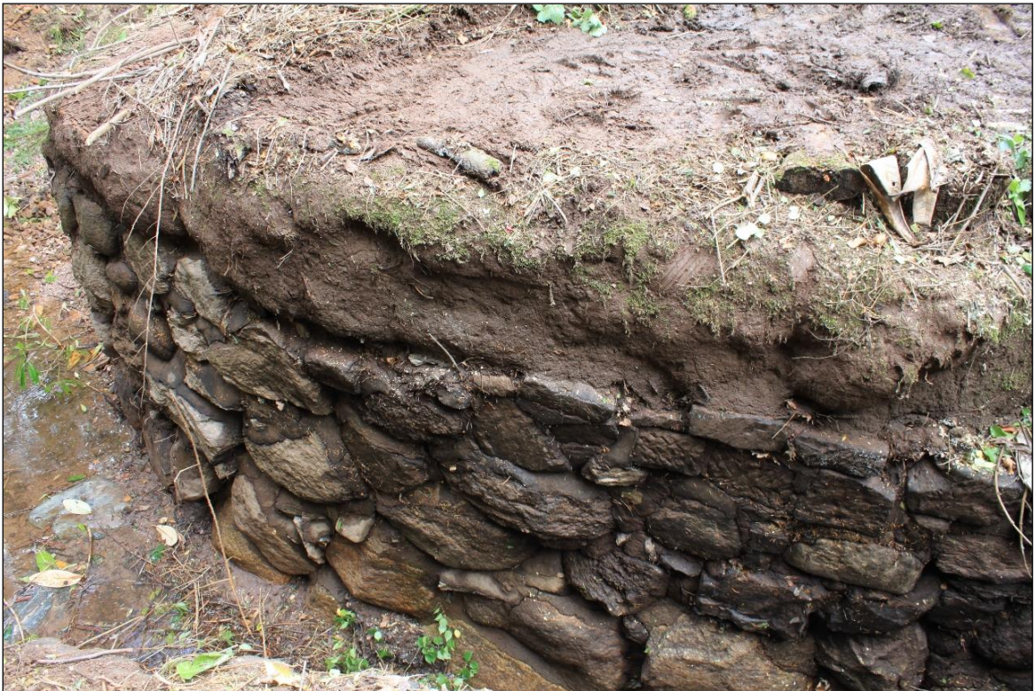
Figure 14: West-facing retaining wall of the sluice structure showing much-worn bonding material.
