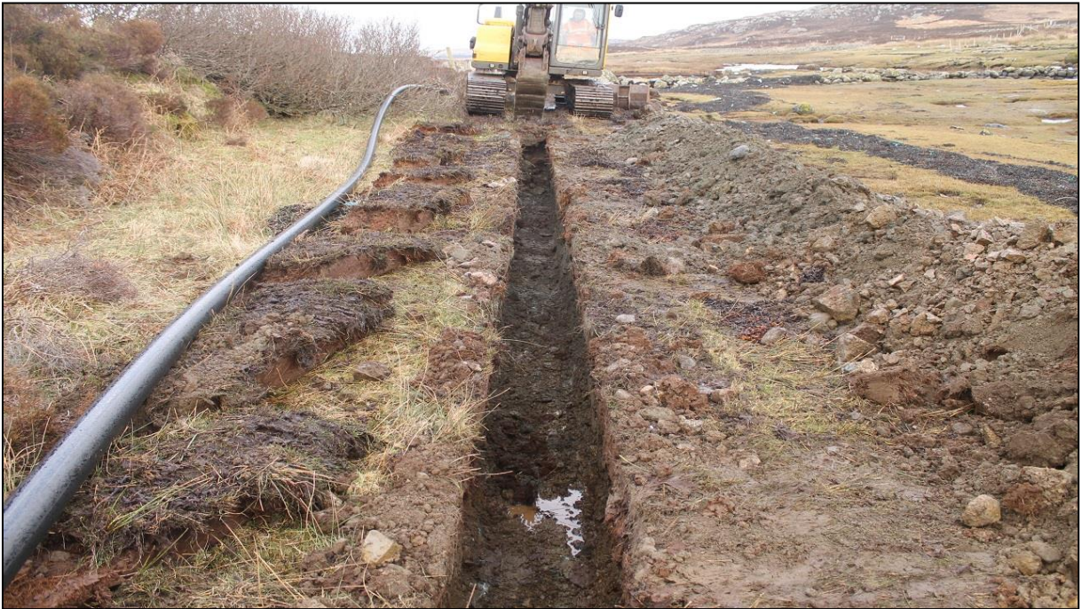
Figure 3a: Working shot of trench excavation at north end of monitoring area
