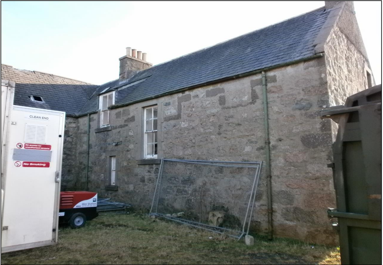
Figure 7a: Northwest elevation of Building J demonstrating the cast iron guttering and downpipe.
