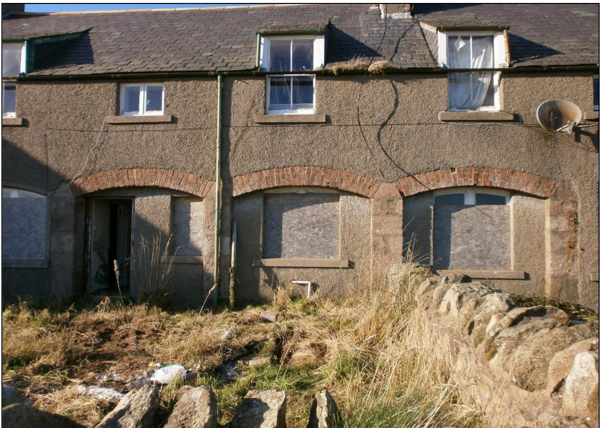
Figure 16b: Building J: southeast elevation with the brick arches and granite columns visible
