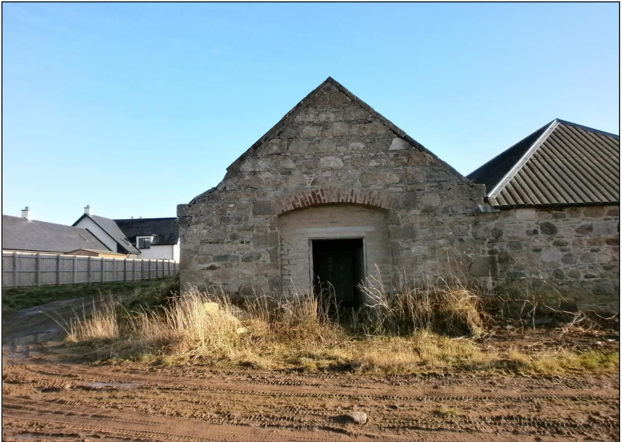
Figure 10a: Building G: southwest elevation showing the original entrance and modern infilling.
