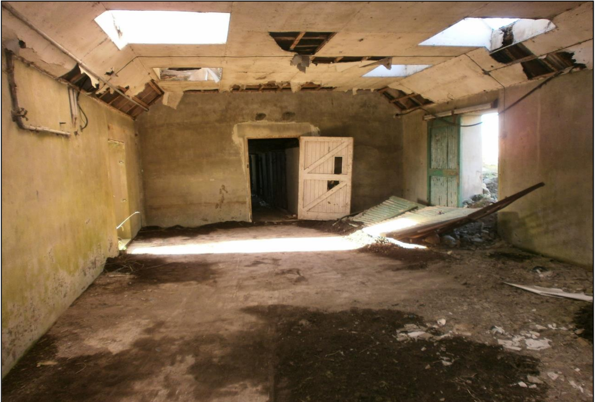
Figure 9a: Building C: showing the southwest end and doorway into Building G.
