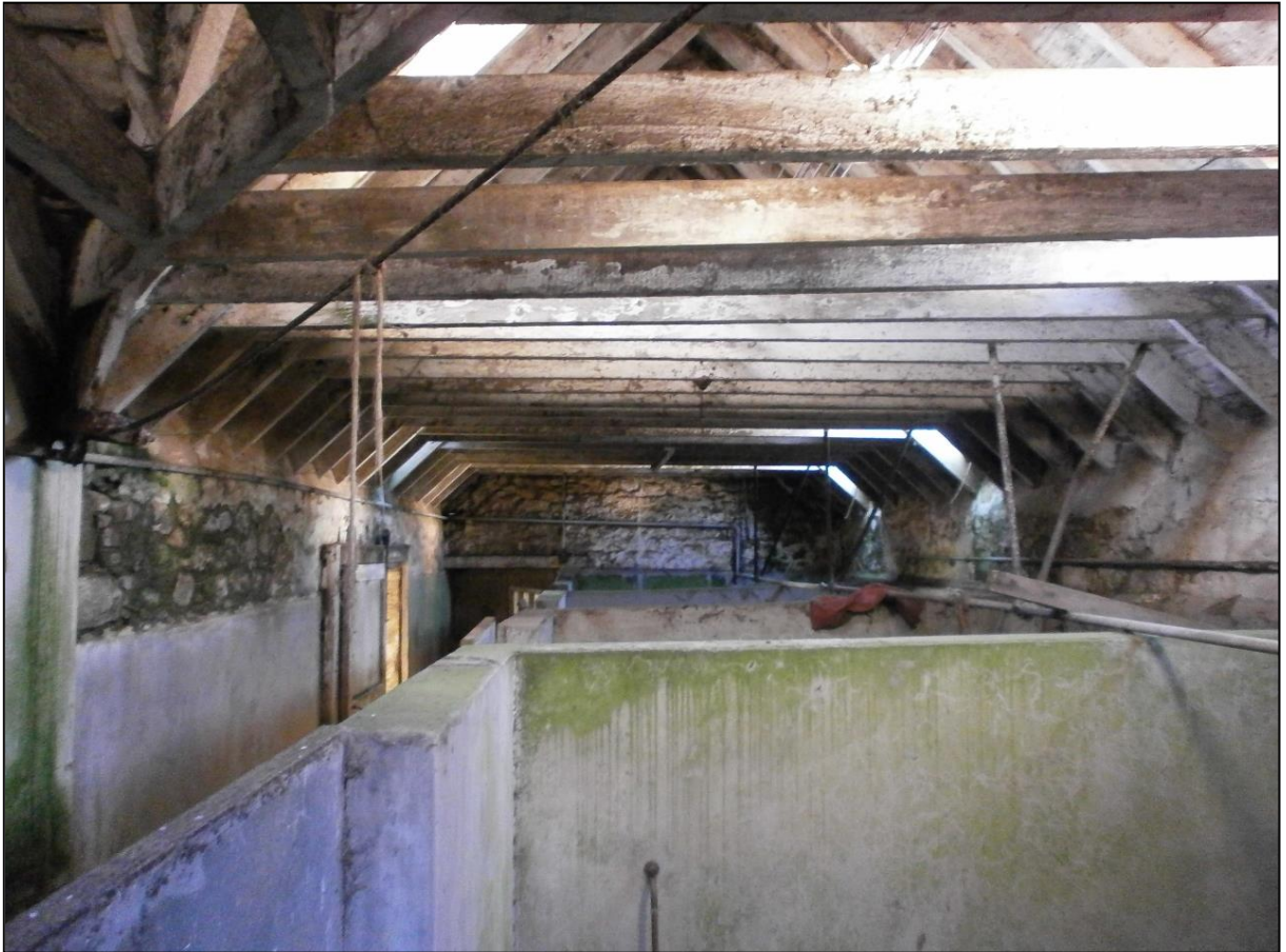
Figure 8a: Building B: view to the southwest showing the concrete livestock pens and timber trusses
