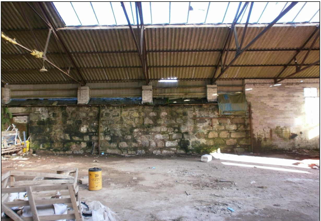
Figure 6b: Building M: northeast elevation showing the sneaked granite rubble and modern roofing.
