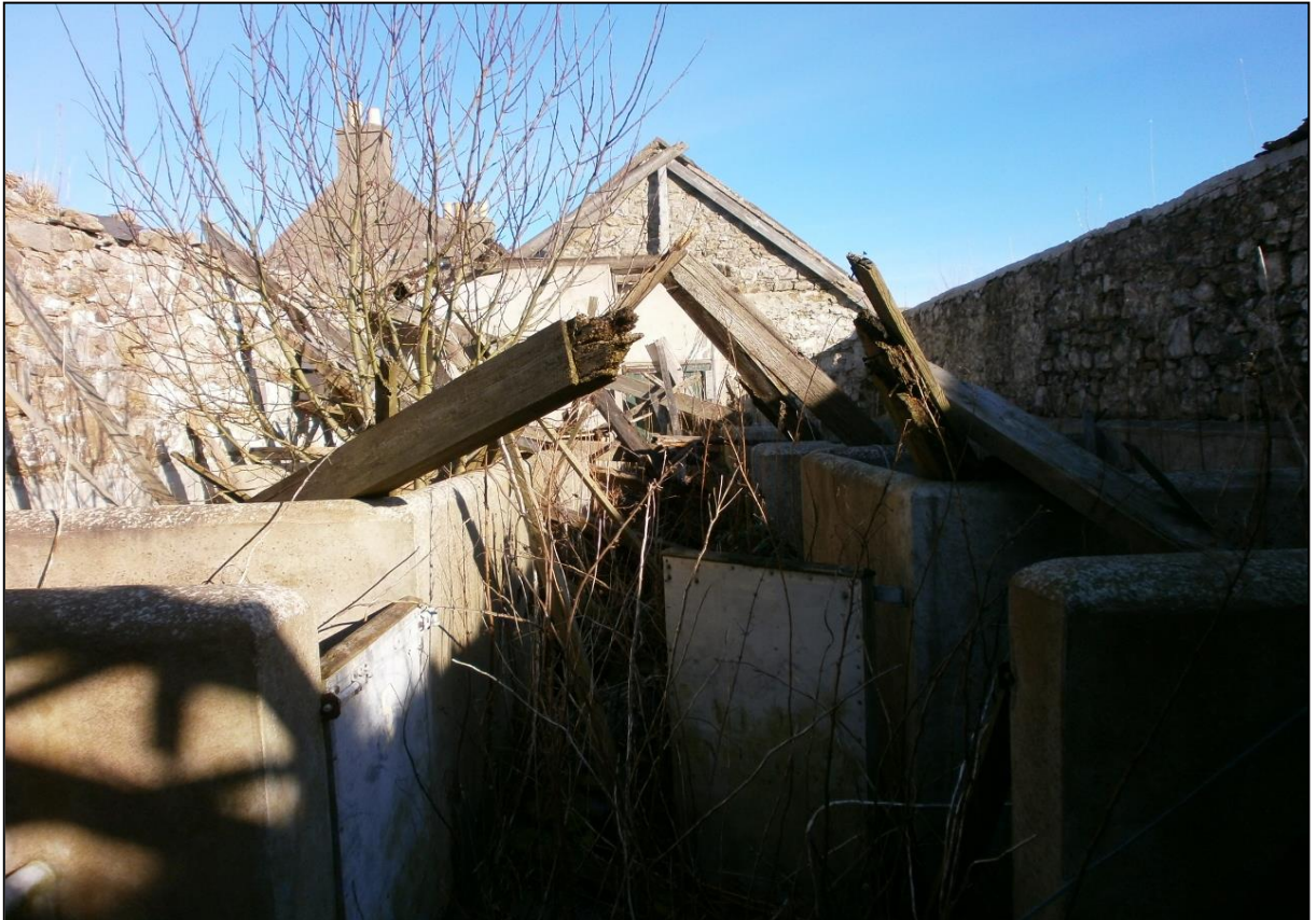
Figure 13a: Building I: showing the structures poor condition and livestock pens
