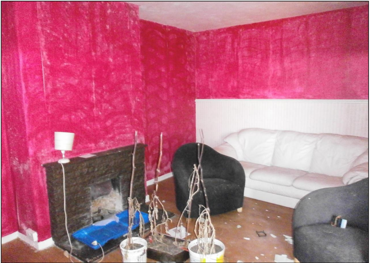
Figure 15a: Building J: Lounge room southwest and northwest walls and fire place
