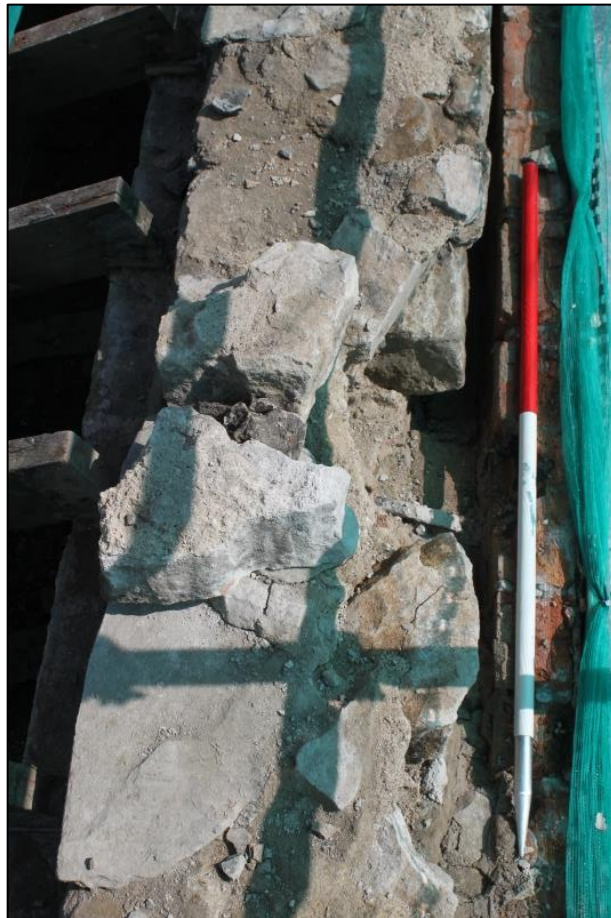
Figure 5b: Wall [006], with Iron Strap [011] to left of Void [010] and modern brick lining [007]
