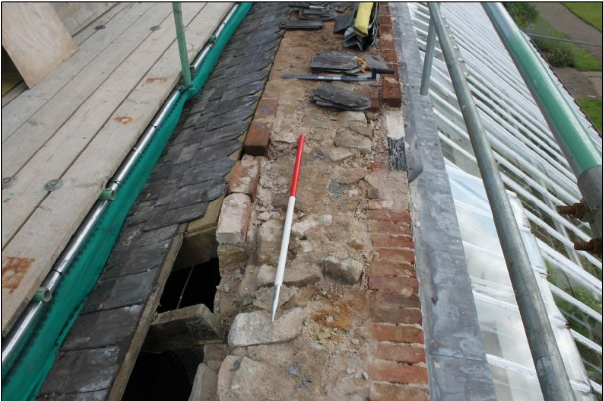
Figure 4b: Transition between Consolidated Fabric [001] & [002] and Original Wall Fabric [006] and Scarcement Ledge [008], with Relaid Bricks [004] and Modern Lead Flashing [005] at SE edge (Looking NE)
