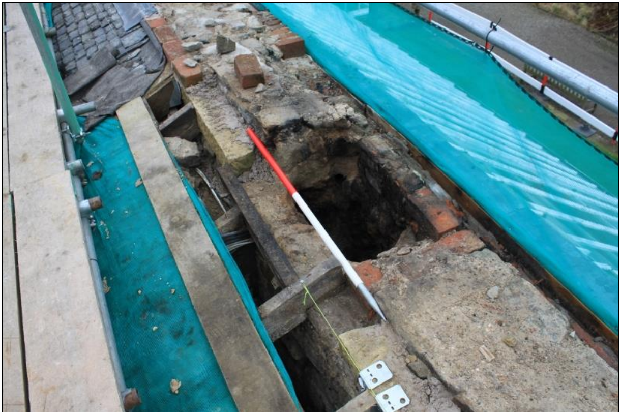
Figure 7b: Flue [029] showing heavy sooting of interior
