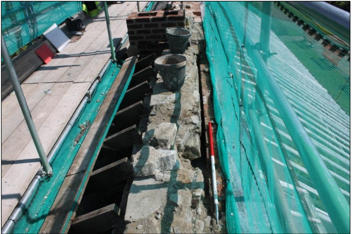
Figure 5a: Rubble Wall [006], with Scarcement Ledge [008] to left and Modern Brick Lining [007] to Right, with Void (010) to rear
