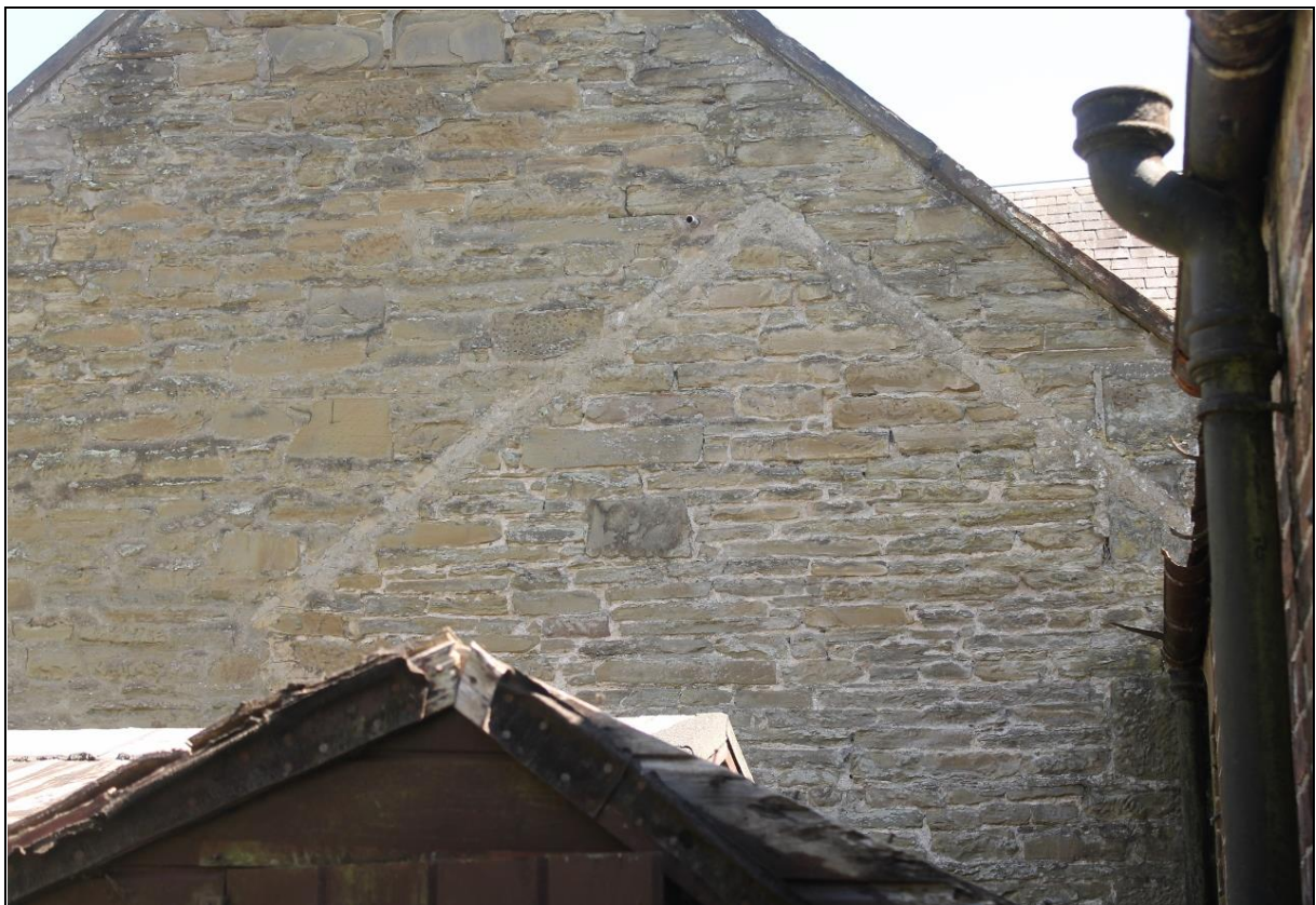
Figure 8b: Rear northeast elevation of the Preaching Hall showing evidence for a previous roof line
