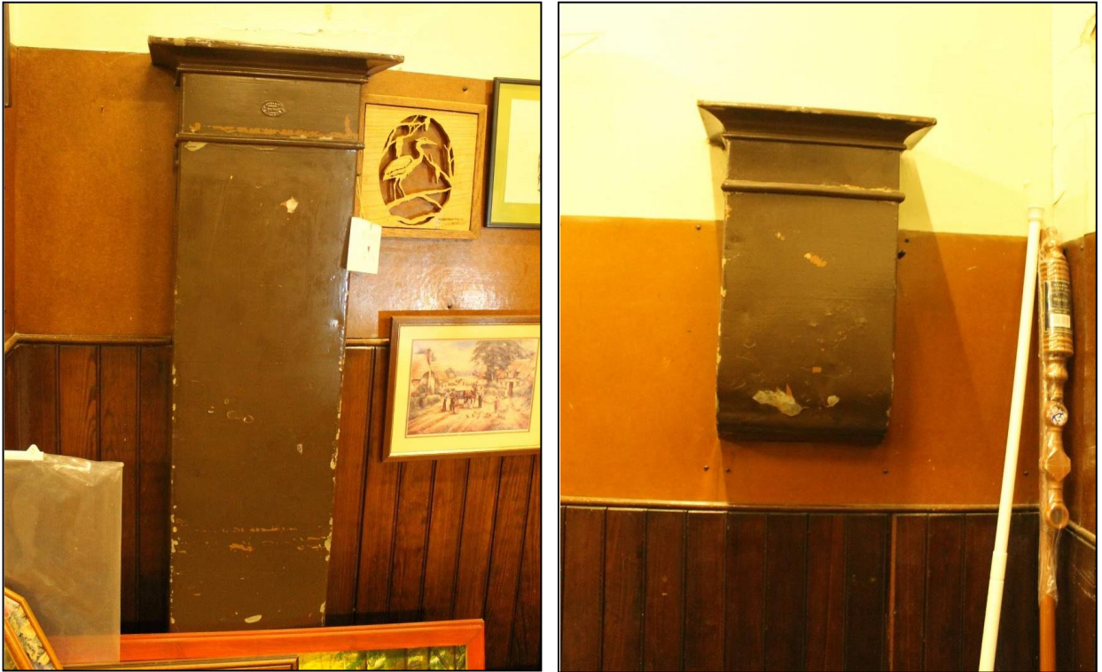
Figure 10a: Heating ducts/vents in the Main Room
