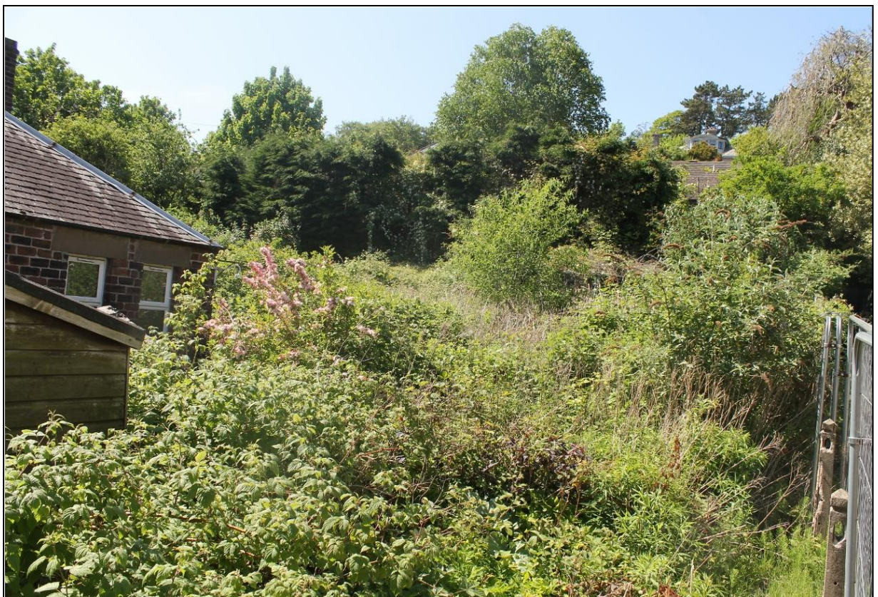
Figure 2b: Thick vegetation at the side and rear of the building made it difficult to gain a clear view of the northwest and northeast elevations
