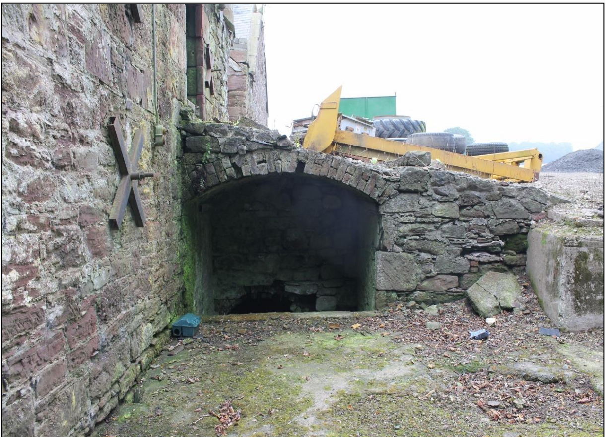
Figure 16b: Access into the underground part of the lade that runs along the side of the South Barn.
