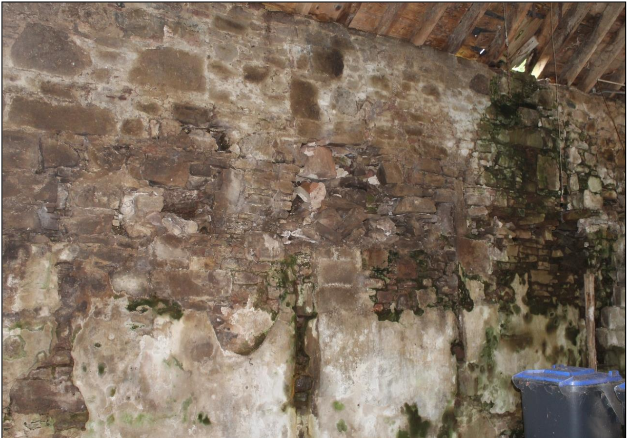
Figure 10b: Northeast wall in North Barn showing damp and evidence of white wash wall.
