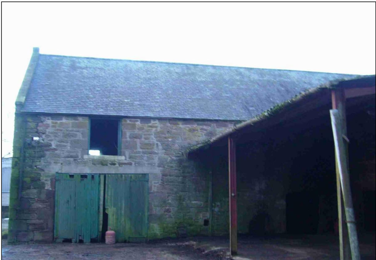
Figure 6b: Structure to the southwest of the South Barn partially taken down
