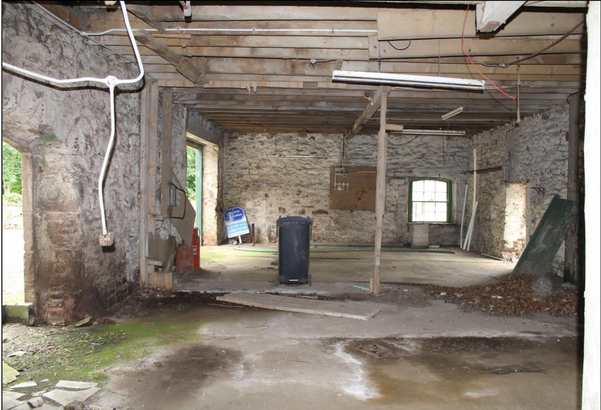
Figure 14b: The southwest-northeast aligned element of the South Barn, showing the white washed walls.
