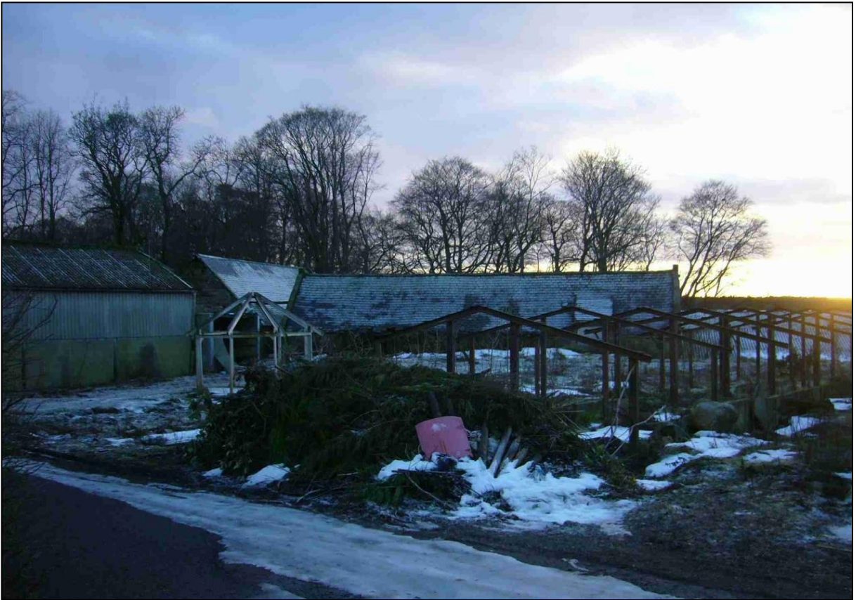
Figure 4b: The Northeast area of the site with building C (Ruinous Greenhouse) in the middle of the image and Building D to the left.
