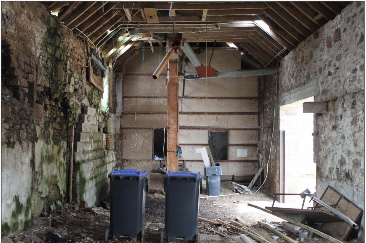
Figure 11a: The North Barn showing the timber roof trusses and grain storage at the southeast end.
