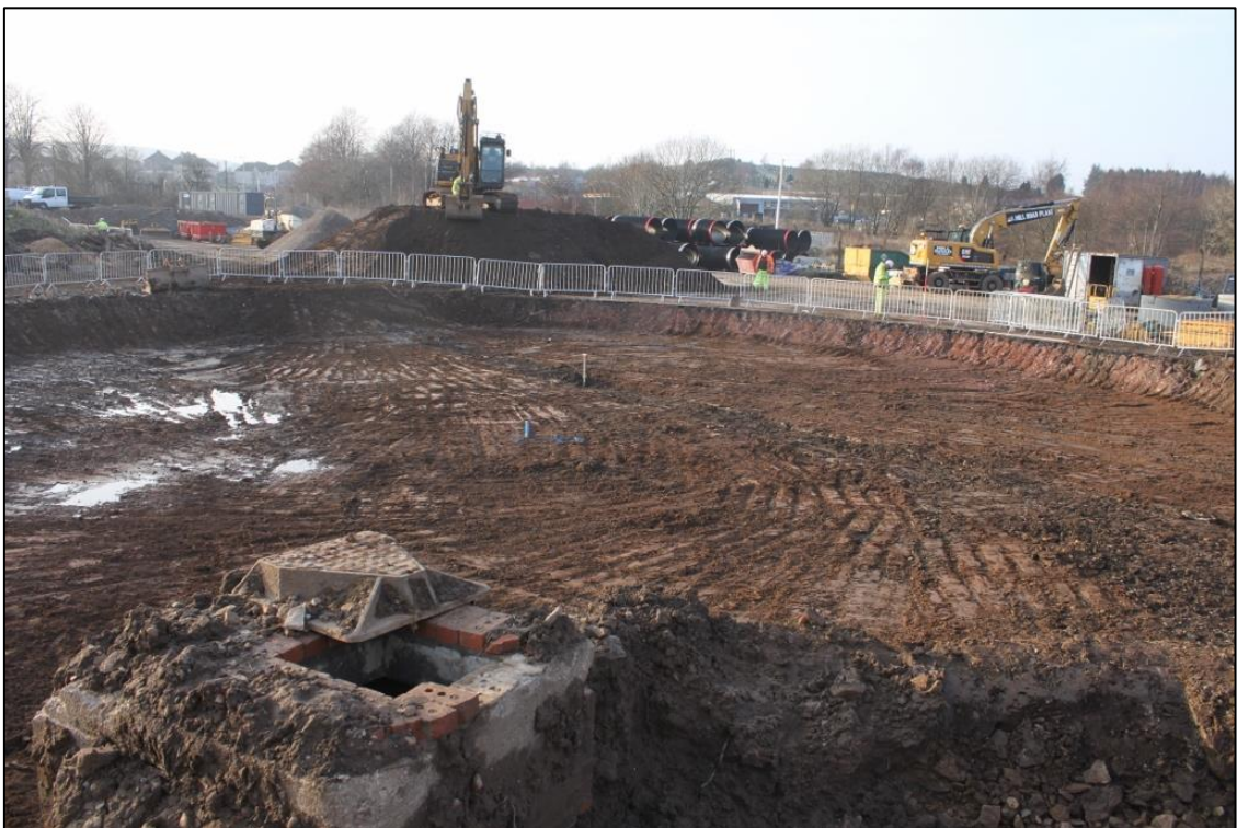
Figure 5b: View of 20th century drainage and pipe (013) within storm tank excavation. From the ESE
