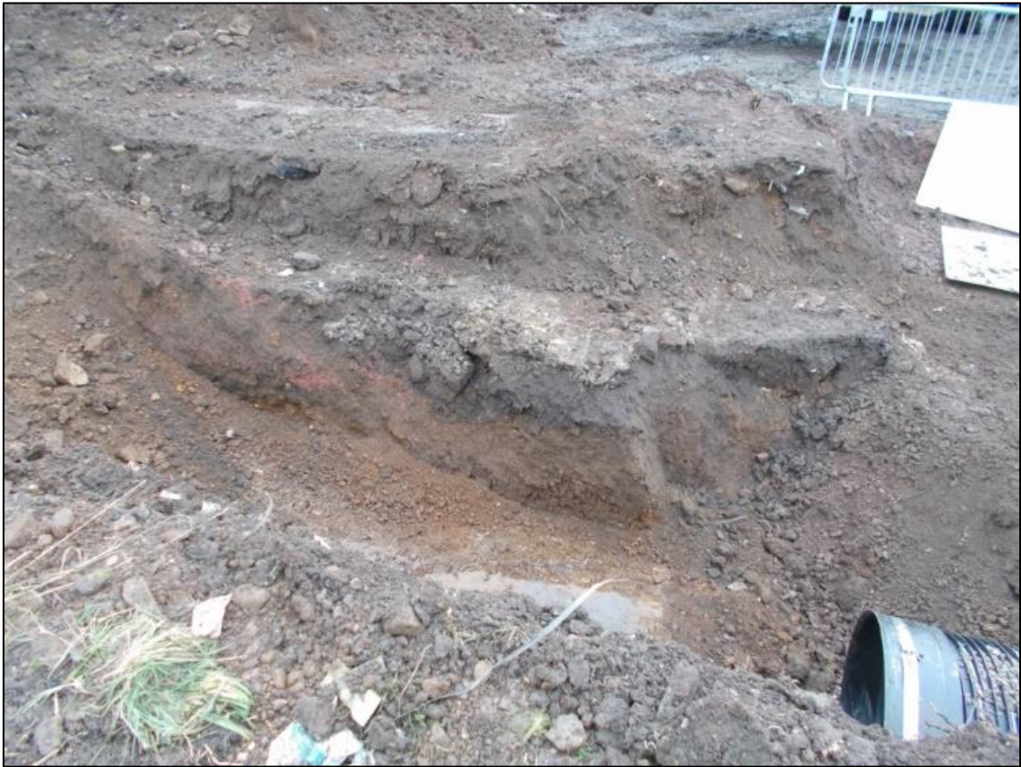
Figure 5a: View of layers (001-003) with in pipeline trench in Area A. From the SW.
