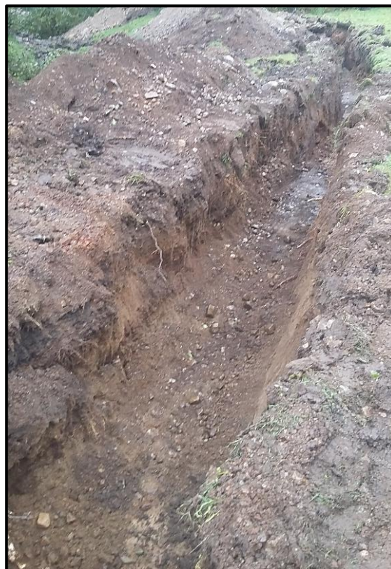
Figure 3b: Post-excavation shot of pipe trench to the northeast side of Allt Mhoille. Taken from the northeast.
