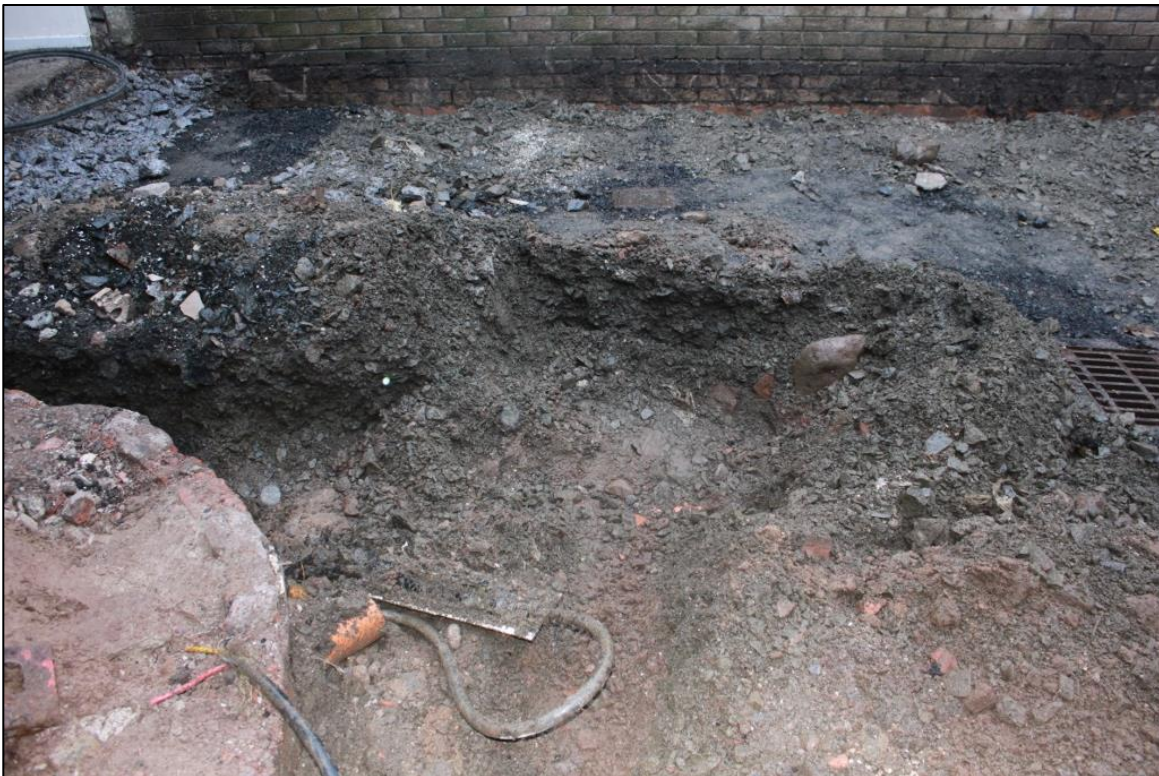
Figure 4b: View of Trench 4 before the removal of the existing manhole. From the S.
