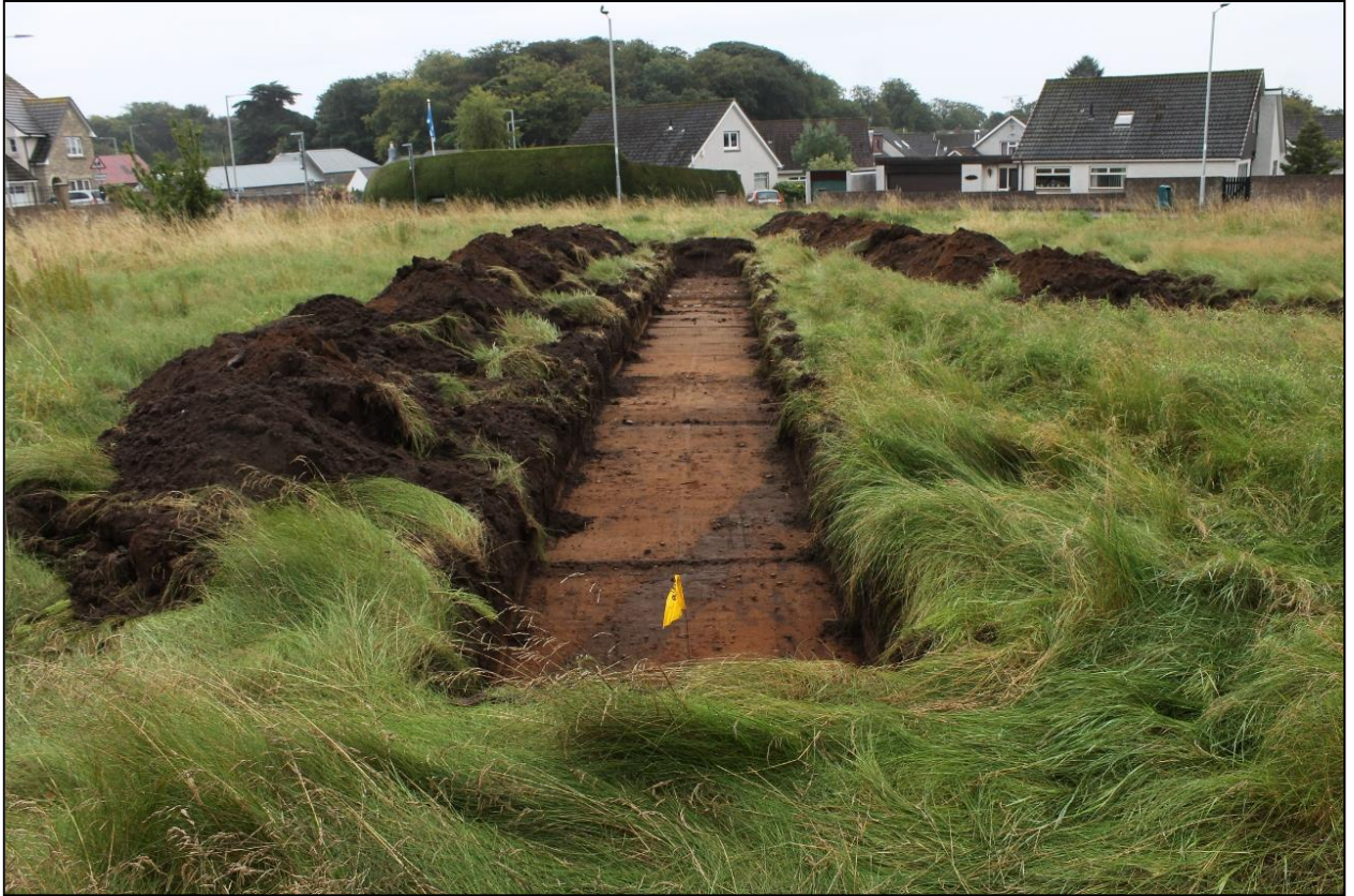
Figure 4a: Trench 2 demonstrating context (002) and the linear feature of a modern field drain [006].
