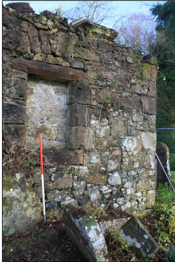
Figure 7a: Fabric 4, with re-used fabric (including quoins) combined with vertical pinning stones
