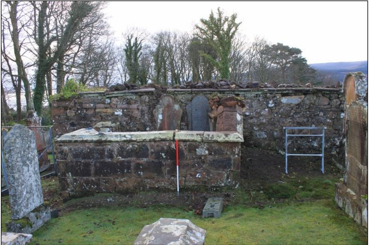
Figure 9a: Fabric 7, Low Enclosure With Stone Coping which Abuts North Elevation at East end
