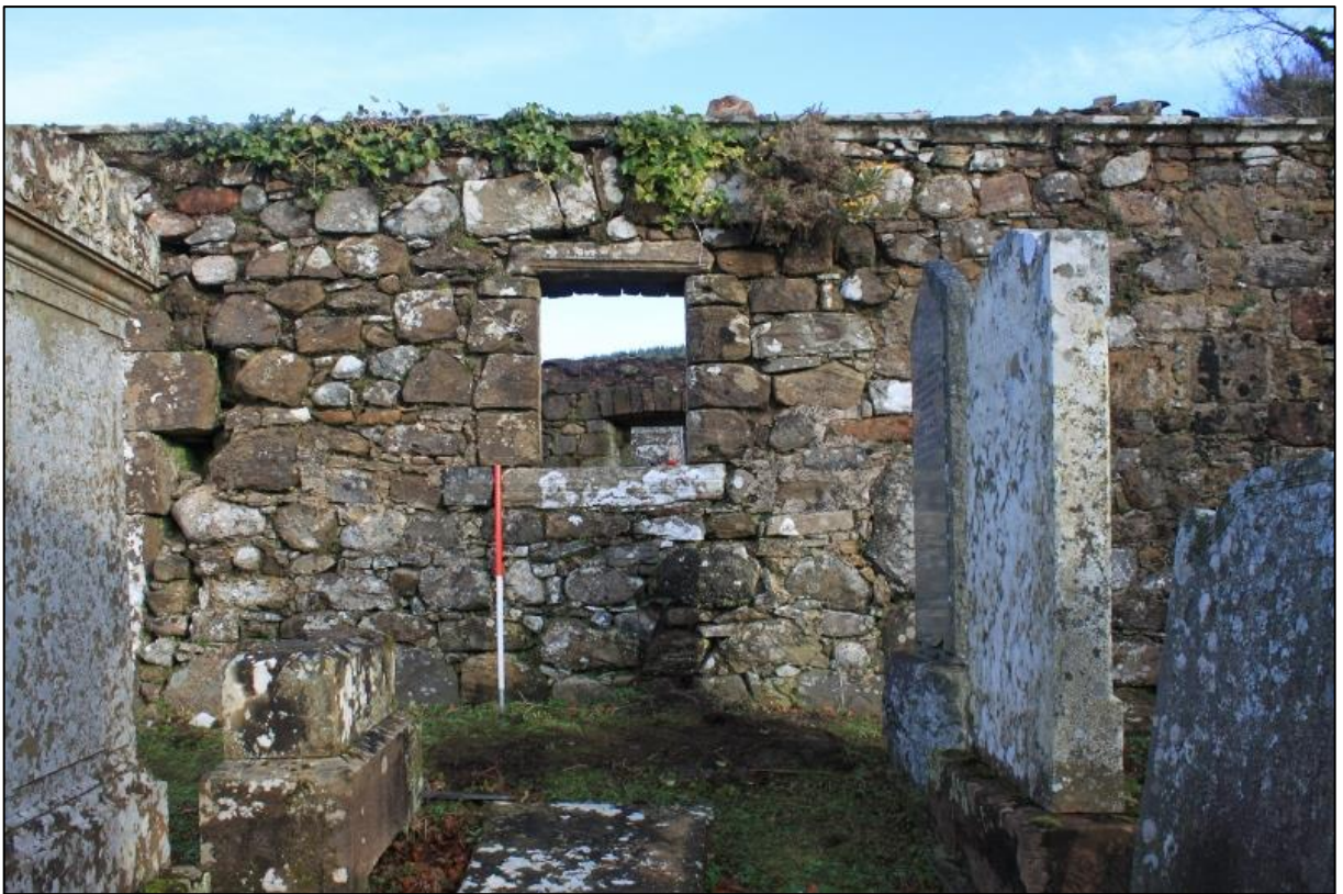
Figure 5b: South Elevation: Fabric 1 in lowermost 3 courses, with Fabric 2 above (excluding wallhead)
