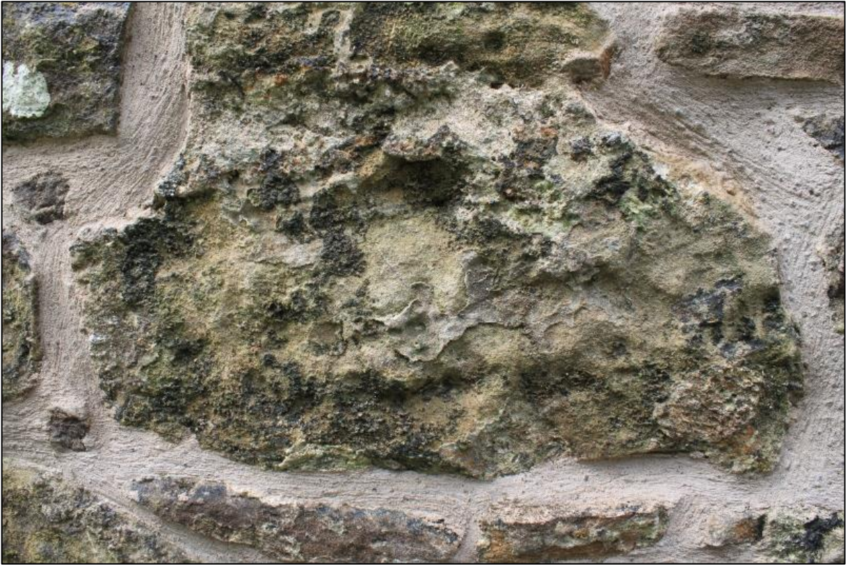
Figure 10a: East Elevation (External) – Relict Harling on Masonry (Joints Repointed during 2017 consolidation works)
