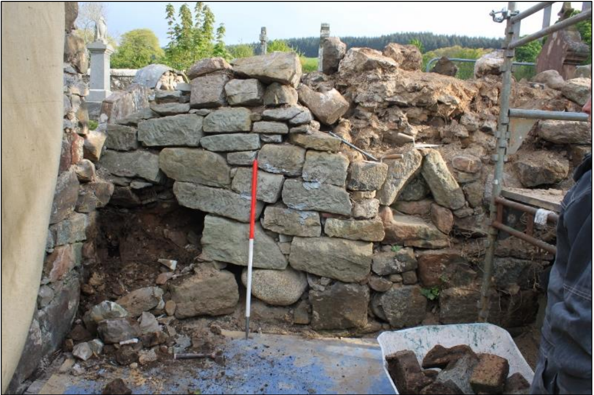
Figure 4a: North-west corner (internal elevation): brick & cement buttress removed to reveal void to rear (former site of tree)
