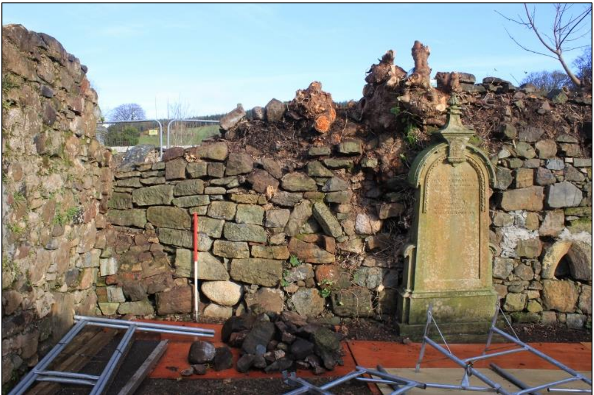
Figure 9b: Fabric 8, Brick/Concrete Buttress in North-West Corner (note also Portland cement to right of memorial stone.
