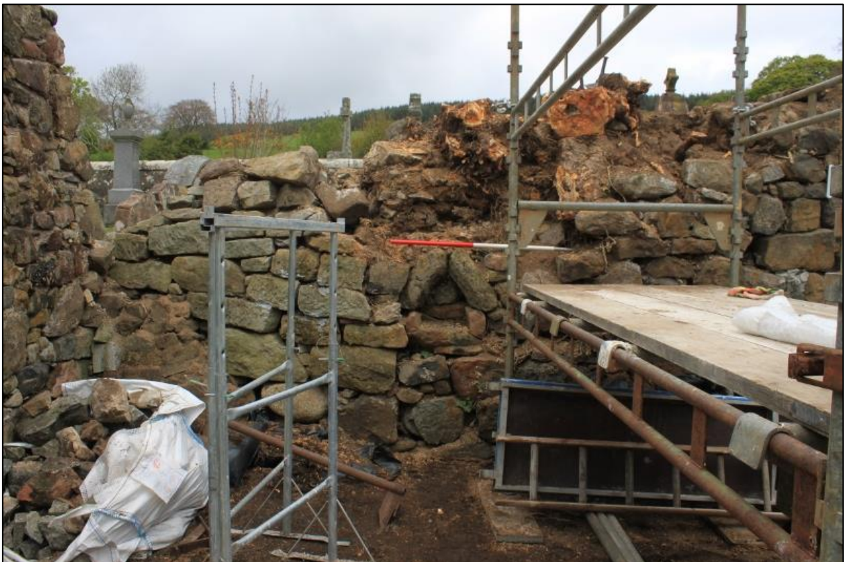
Figure 3b: North-west corner (internal elevation): works in progress, upper courses removed to reveal substantial portion of root mass
