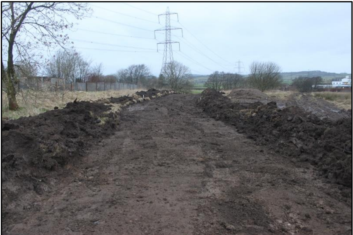
Figure 1b: Post excavation shot of footpath showing subsoil (003). Taken from the southeast.
