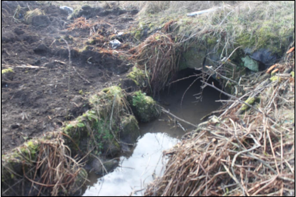
Figure 3a: Covered 'Arched' sluice channel and south eastern stone lining [006] mid excavation. Photo taken from the northeast.
