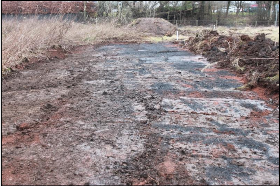
Figure 1a: Post excavation shot of footpath showing topsoil (001) and made ground (002). Taken from the South
