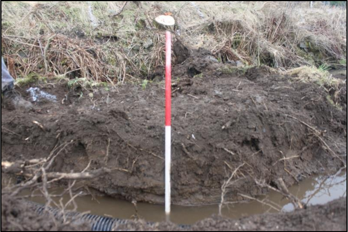
Figure 4a: South facing section of burn diversion with the pipe laid showing (001) and (003). Photo taken from the south.
