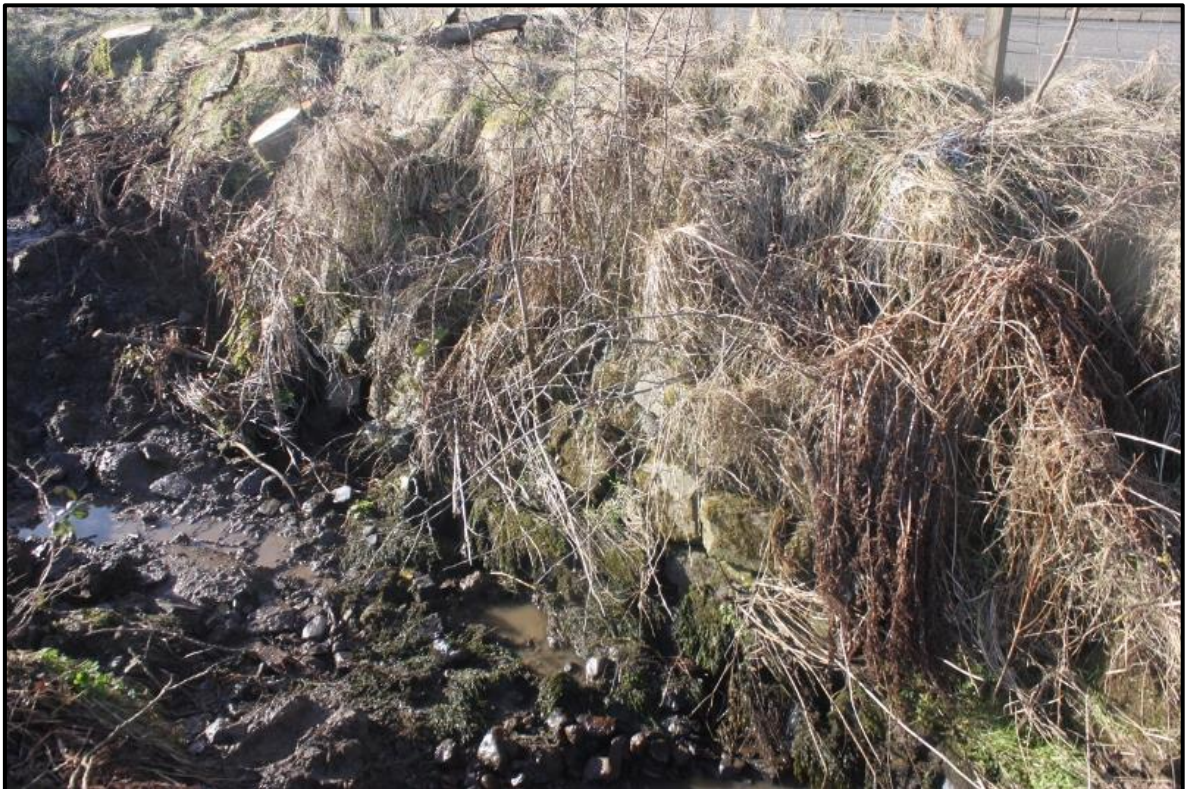
Figure 3b: View of the northwest side of sluice channel, showing stone wall [007]. Photo taken from the east.
