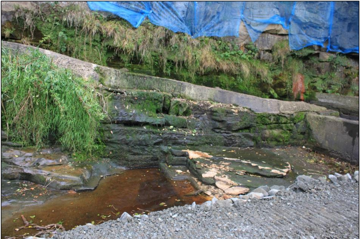
Figure 3b: View of shuttered concrete wall [005] and the sandstone wall [003] beneath. From the S.
