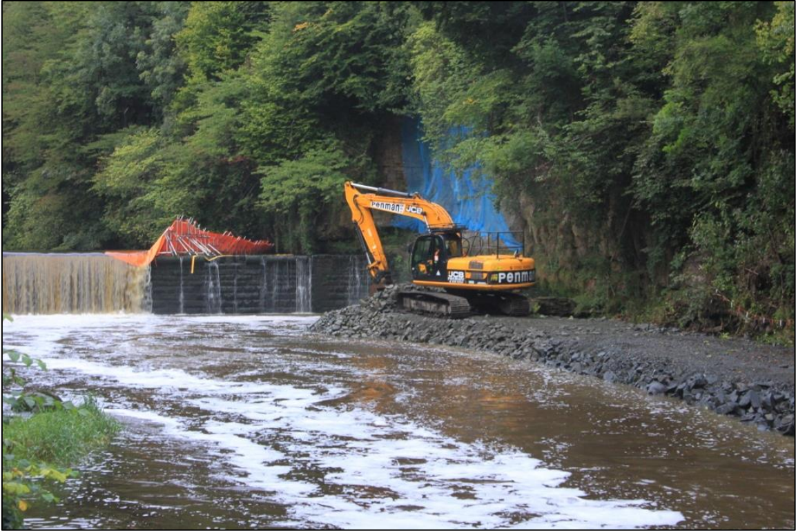
Figure 6a: General view of the Weir and the Fish Pass at the start of site works. From the ENE.
