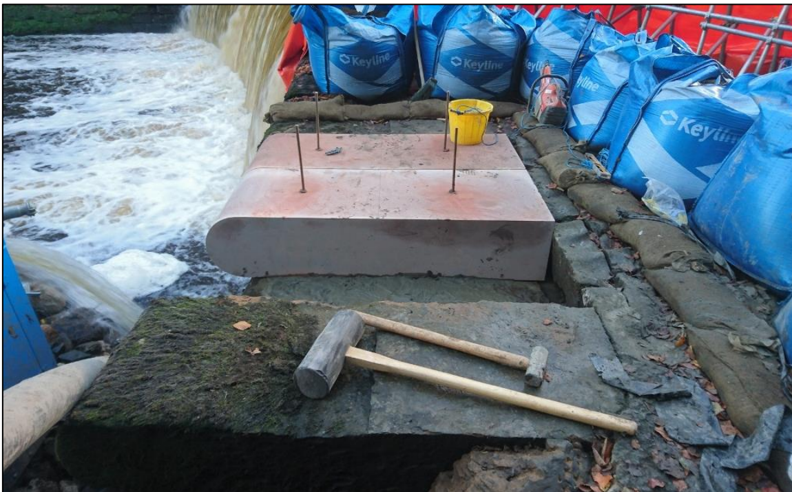
Figure 7b: View of repairs at N end of Weir. From the N.
