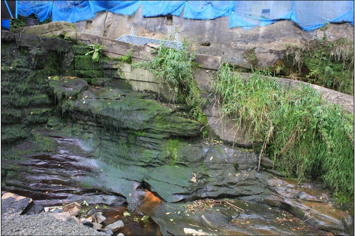
Figure 3a: View of shuttered concrete walls [010] & [005] and the sandstone wall [015] beneath. From the SSE.
