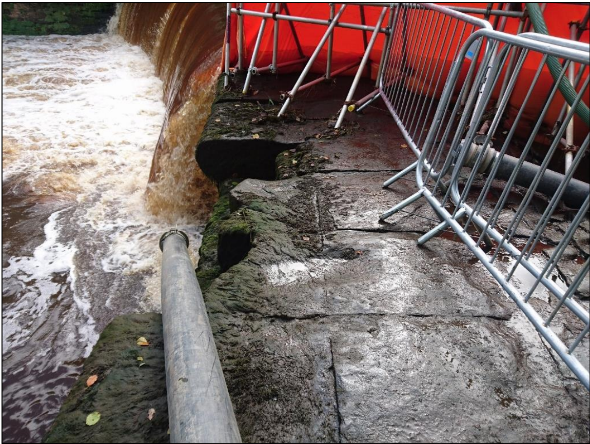
Figure 7a: View of damaged crest blocks at N end of Weir. From the N.
