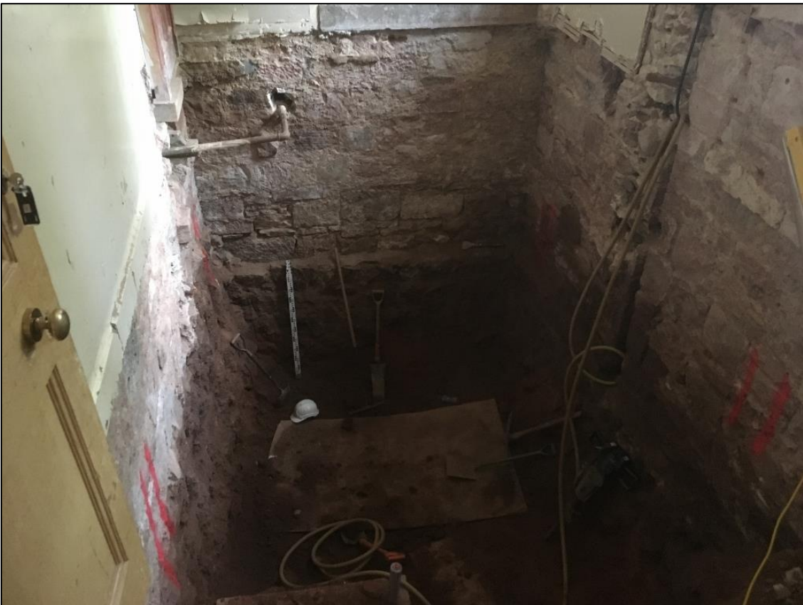
Figure 3b: Post excavation view of lift shaft trench at 3m from existing floor level. From the NE.
