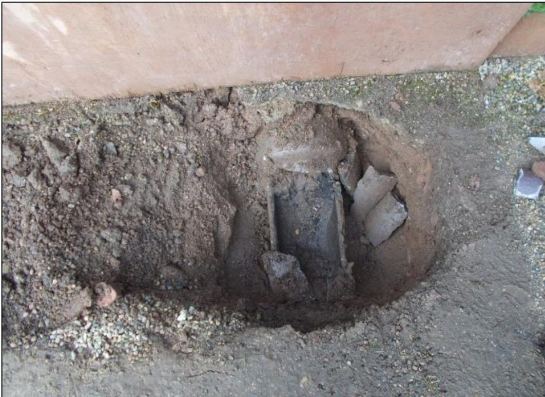
Figure 6b: Post excavation view of Gardeners pit showing ceramic pipe (014). From the SE.
