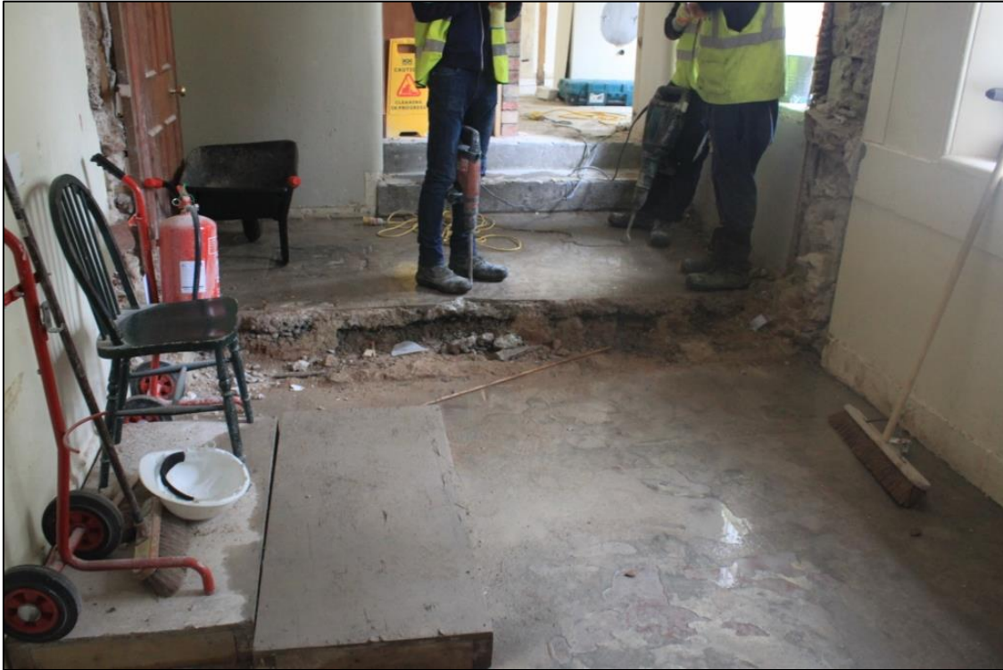
Figure 2a: Pre excavation view of Rooms 21/23 from the NE. Shows raised concrete surface (007).
