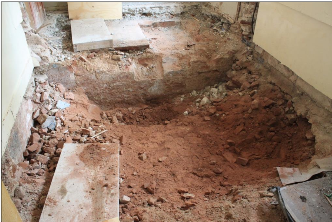
Figure 2b: Mid excavation view of Rooms 21/23 showing wall [008] and rubble layer (003). From the NE.
