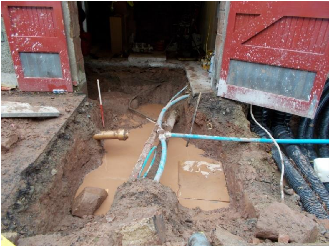
Figure 5a: View of the trench in Bobby's Building and courtyard. From the SE.
