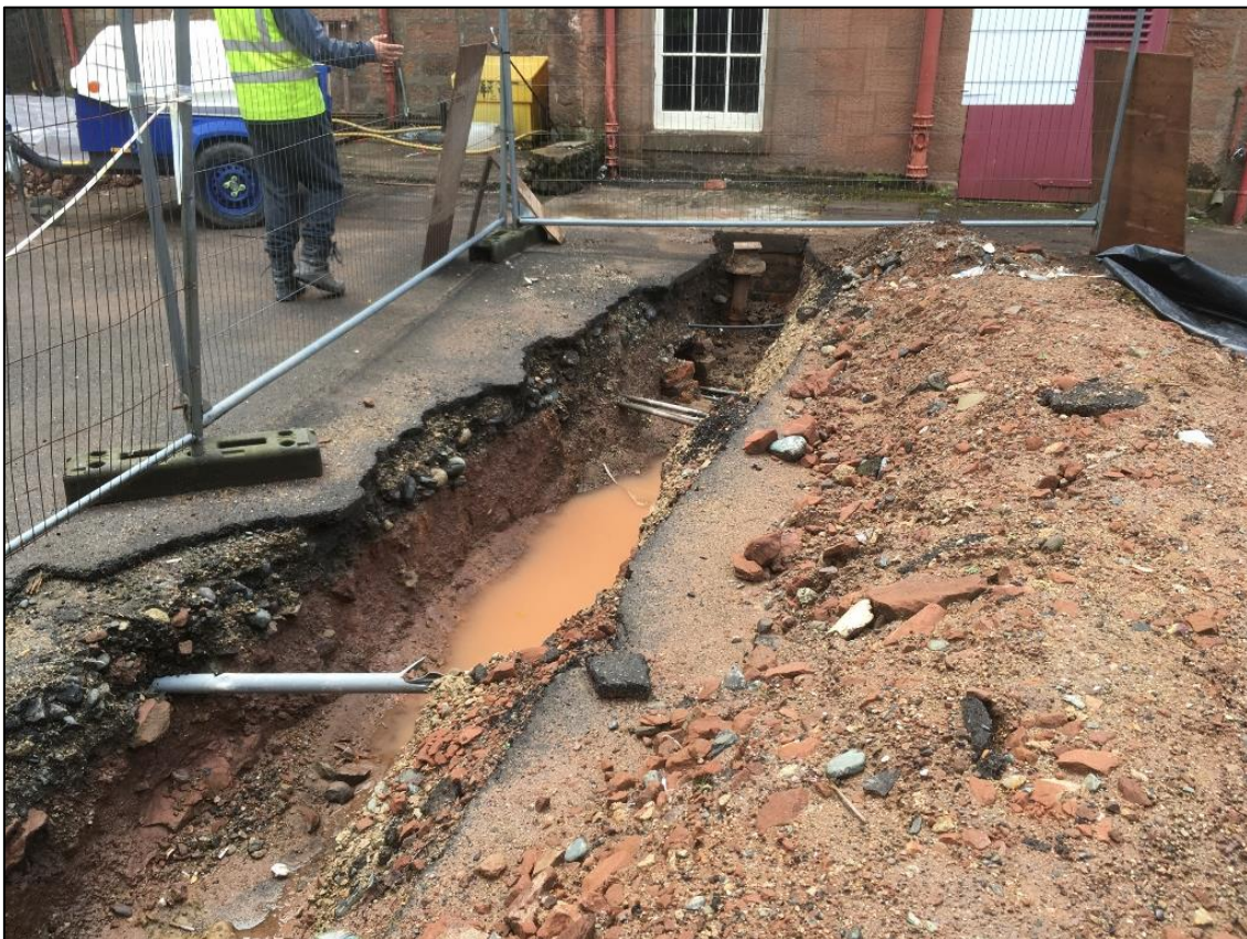
Figure 4b: Post excavation view of the umbilical trench in the courtyard. From the NW.
