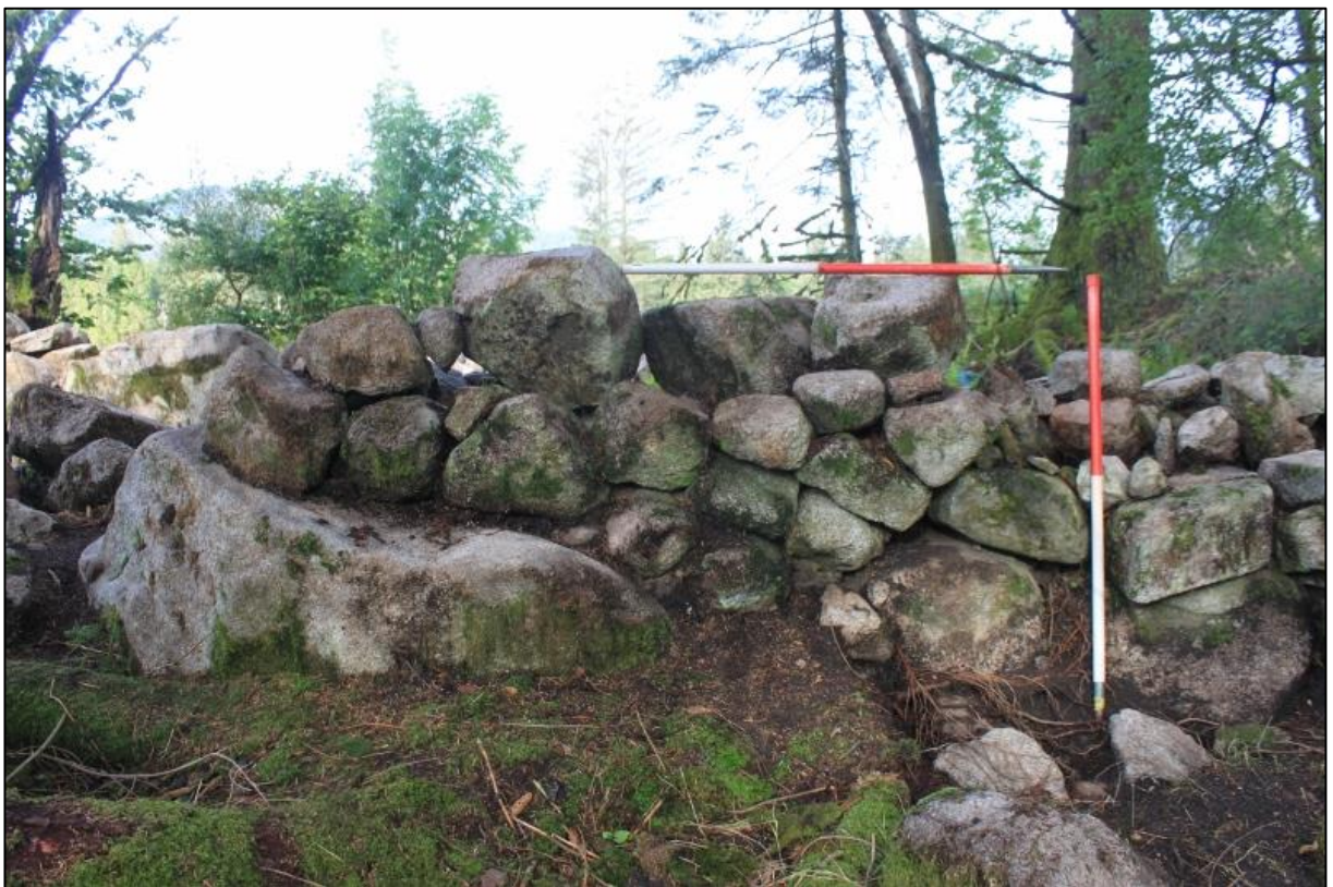
Figure 3b: External east facing elevation of [008] showing higher surviving section of wall
