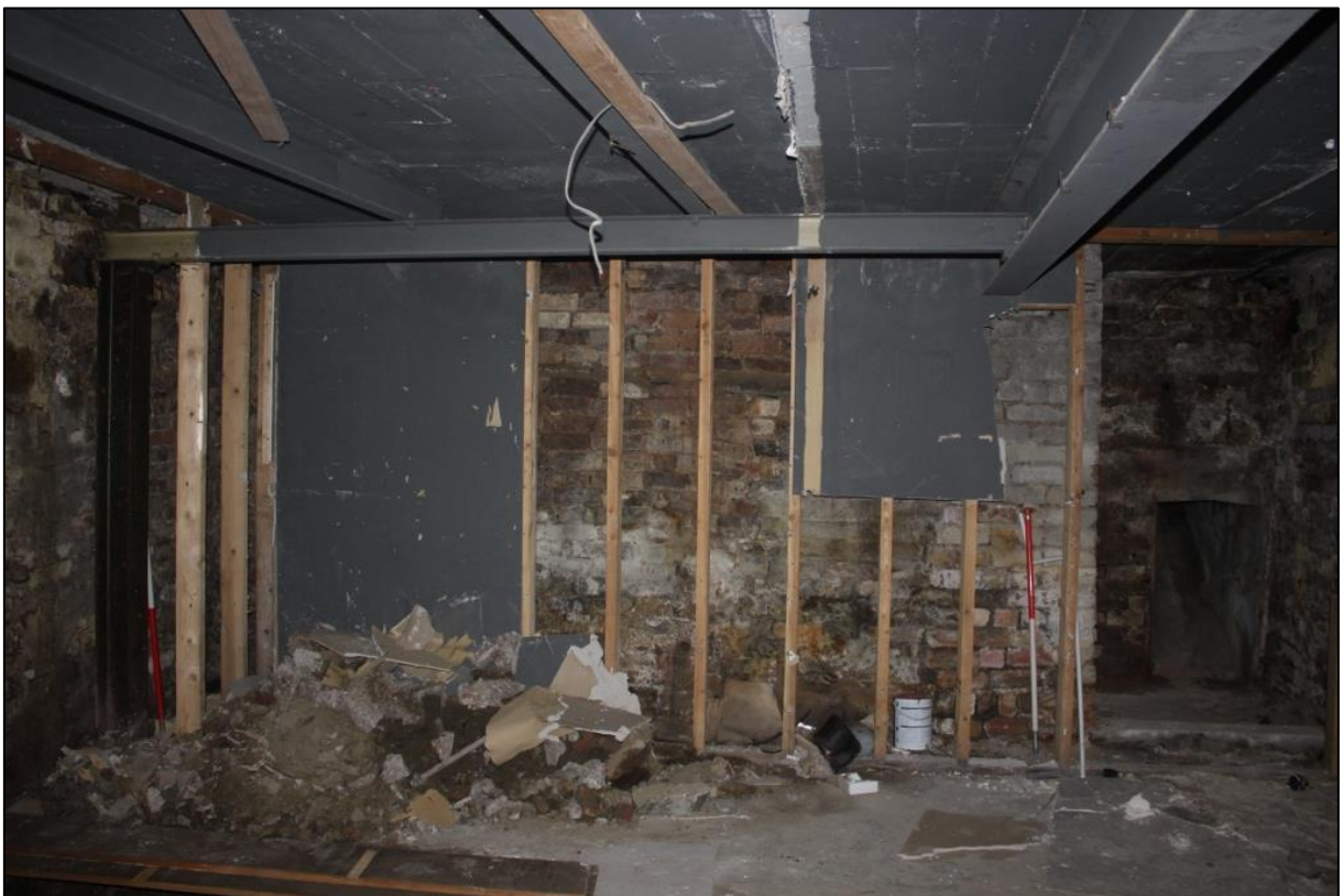
Figure 12b: View of Room 10a showing N facing wall of Building 1a. From N.
