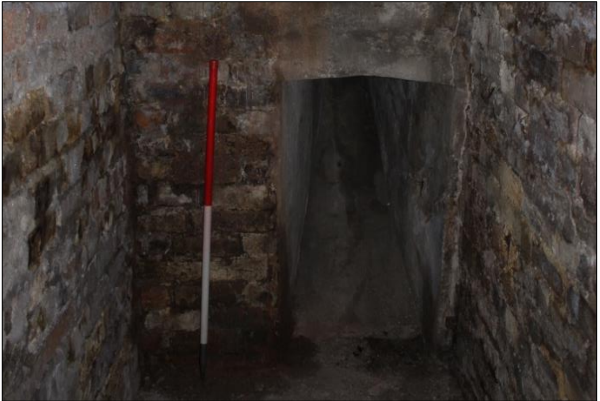
Figure 13a: View of coal chute in N facing wall, Room 10a, Building 1a. From the N.
