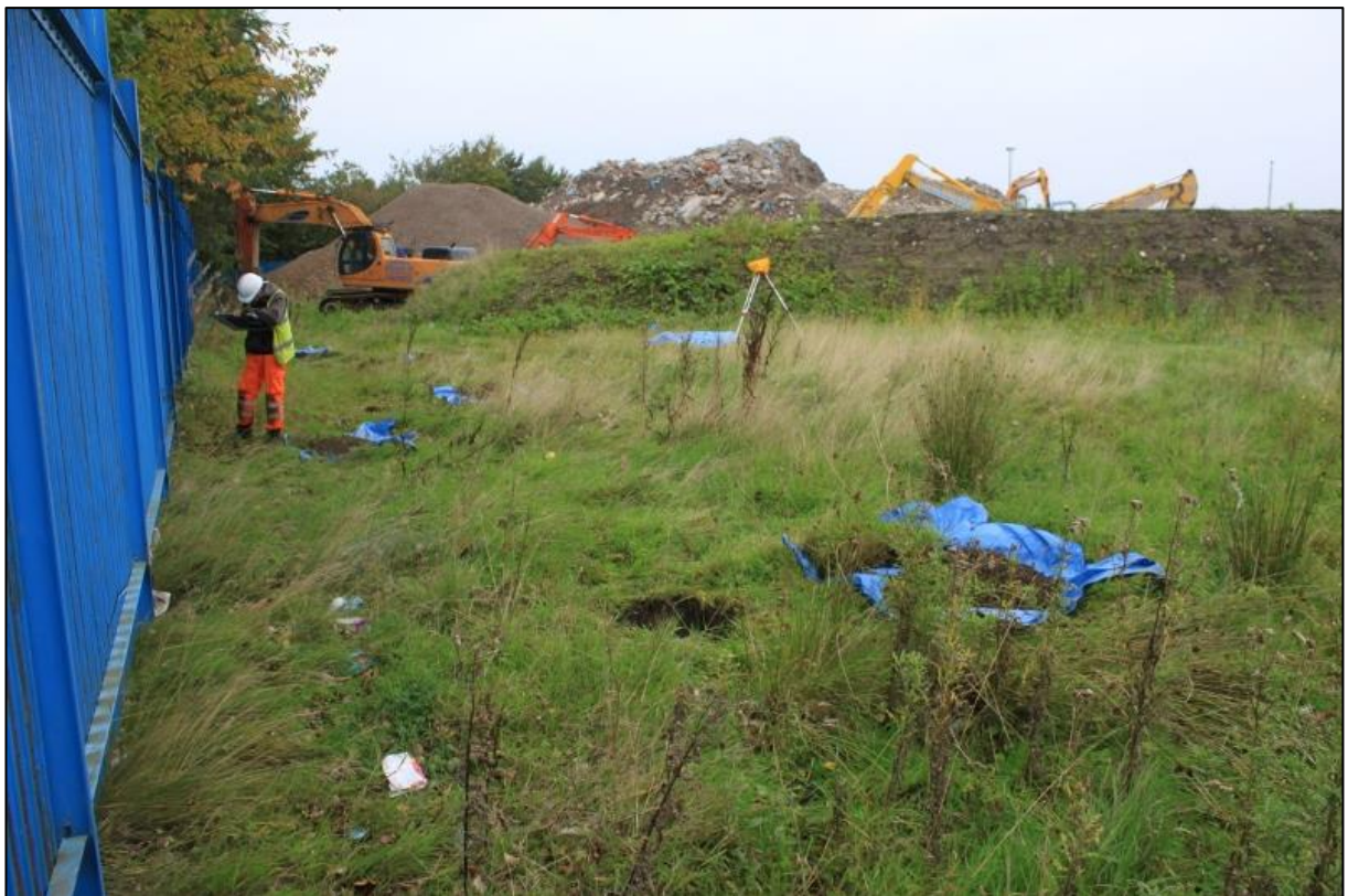
Figure 4b: TP array from SW, palisade fence and bund
