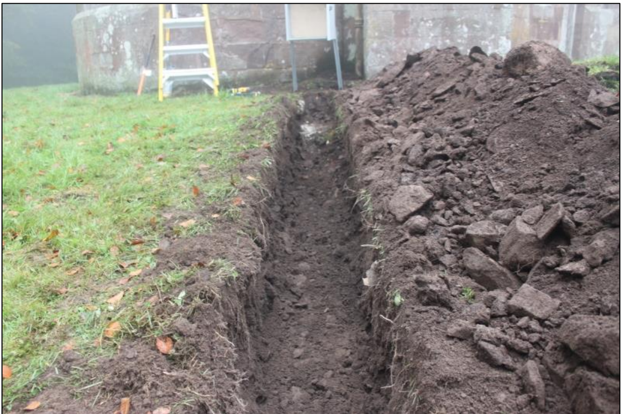
Figure 3b: Shot of service trench showing subsoil (002). Photo taken from the northwest.
