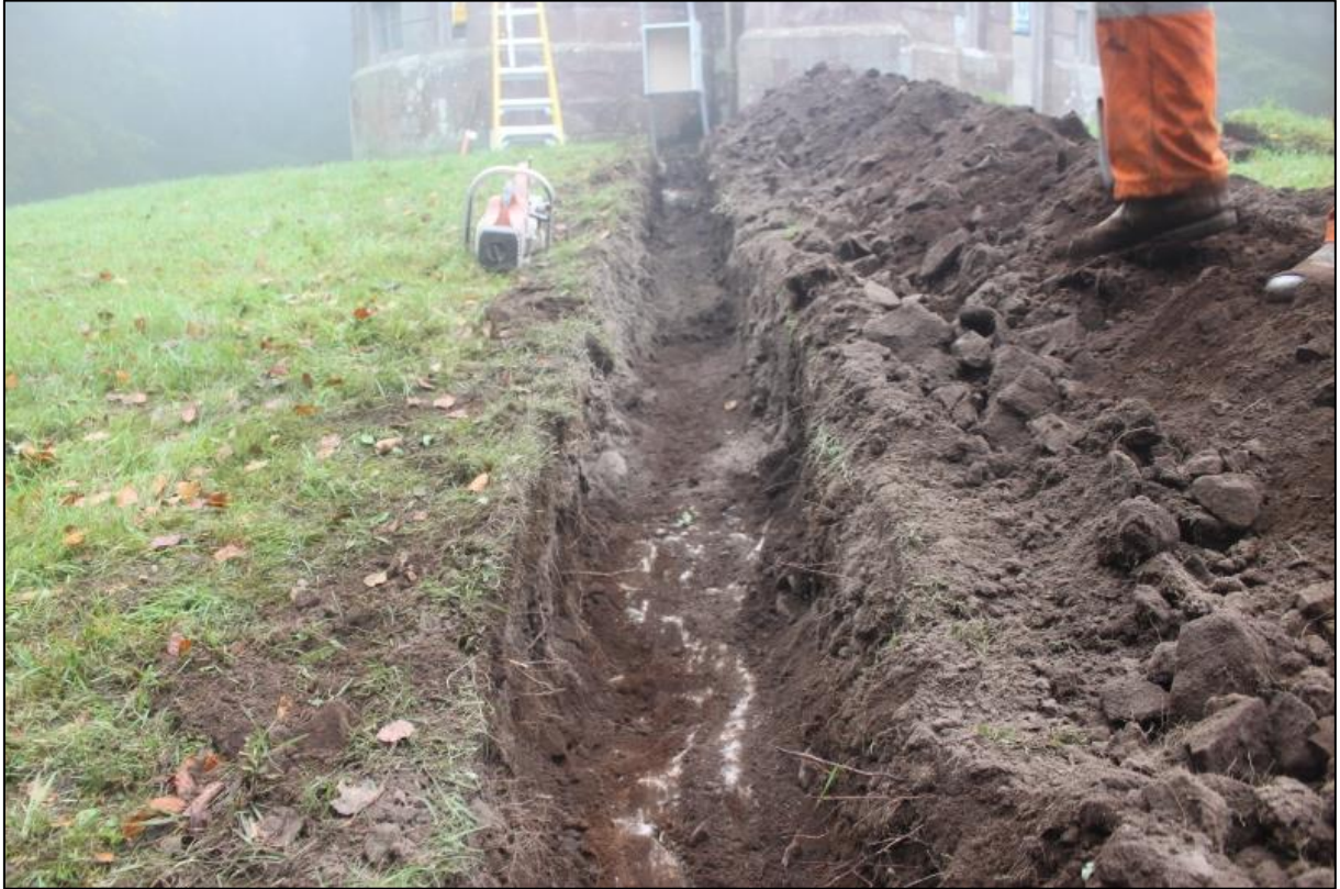
Figure 3a: Post-excitation shot of service trench showing bedrock (003). Photo taken from the northwest.
