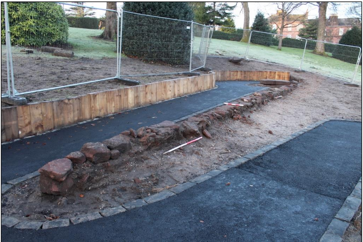
Figure 6b: General view of the public access works around well [005] and wall [004] from ESE.
