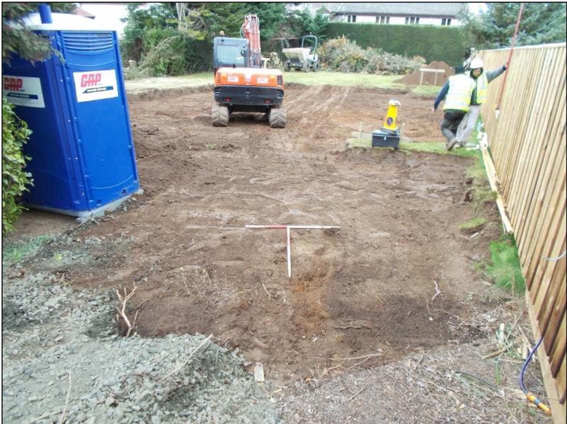
Figure 4b: General view of the area for the driveway from the east-northeast
