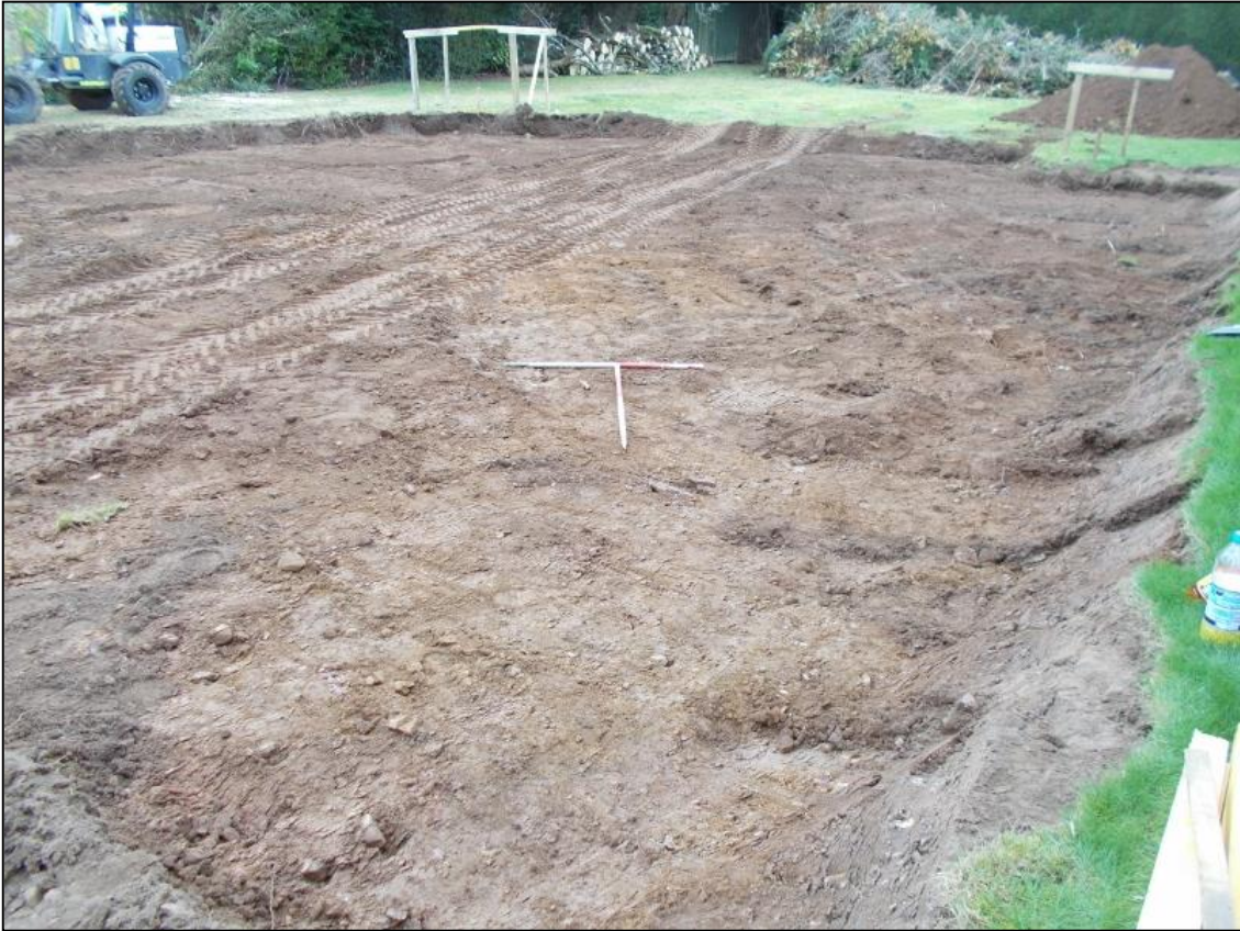
Figure 4a: General view of the house plot from the northeast showing subsoil (002)
