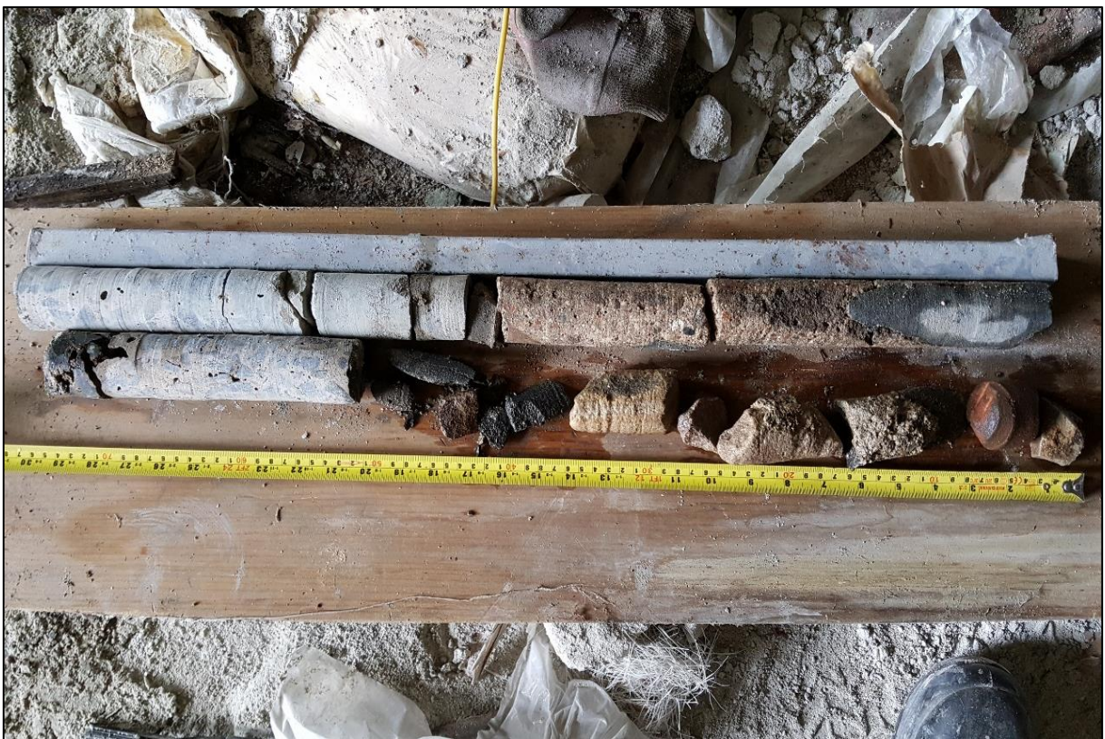
Figure 3b: Two full depth cores through retaining structure, existing surface left of image.
