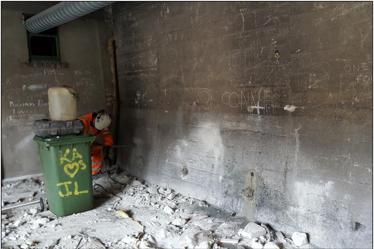
Figure 3a: Coring through shuttered concrete finish in garages on line of Moat Wall.
