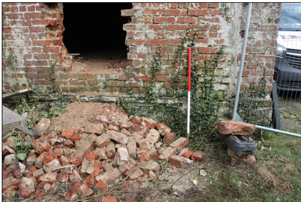
Figure 6b: S Elevation of Element 1, SE Corner, Showing Plinth Courses Composed of Mortared Rubble
