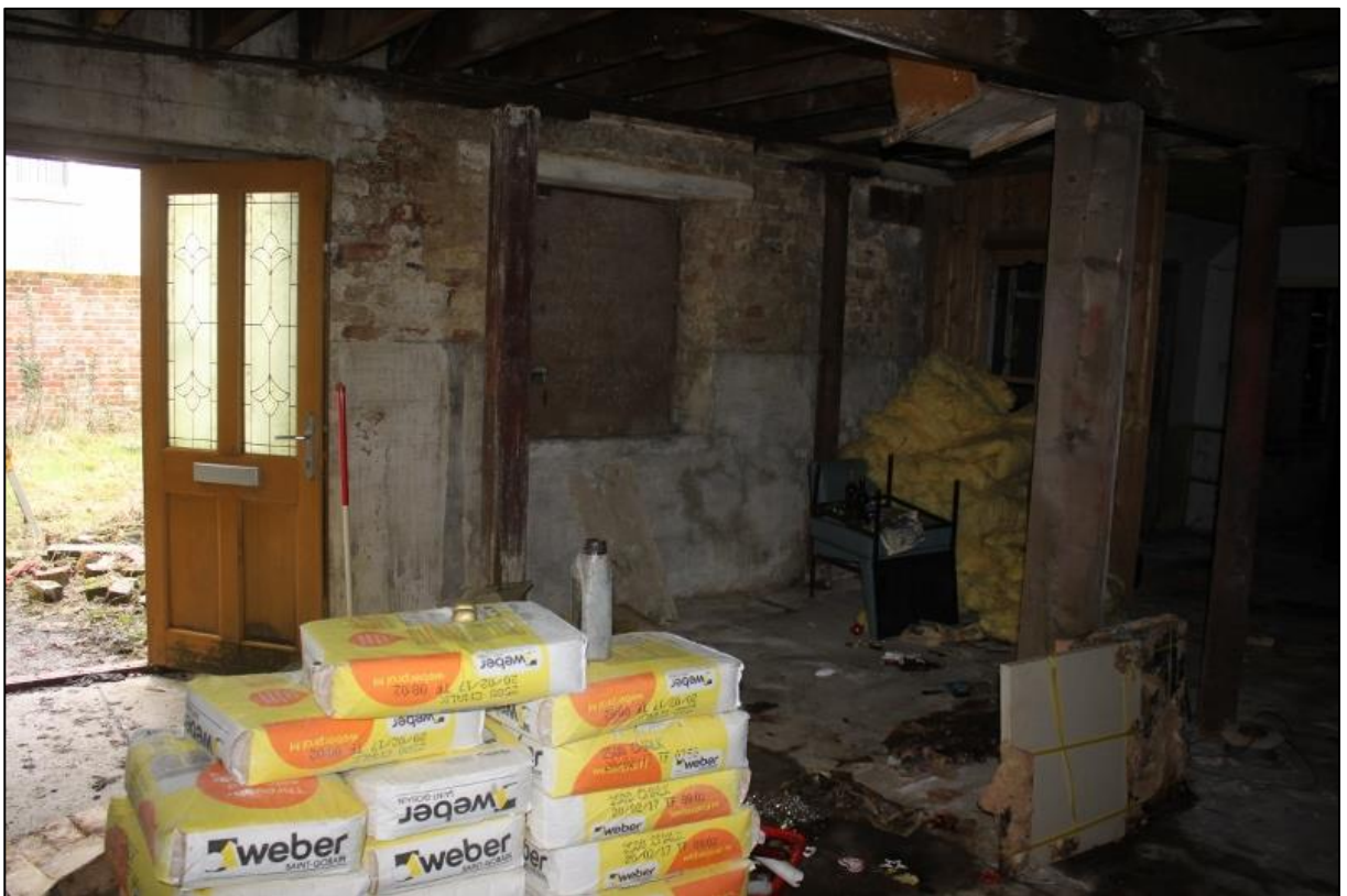
Figure 9b: Element 1, Modern Doorway and Window in W Wall (W Elevation), with concrete lintels
