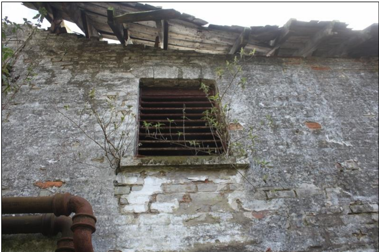
Figure 7b: Detail of Louvred Opening at 1 st floor level, N end, Showing Original Timberwork, Broached Sandstone Sill and Segmental Arch
