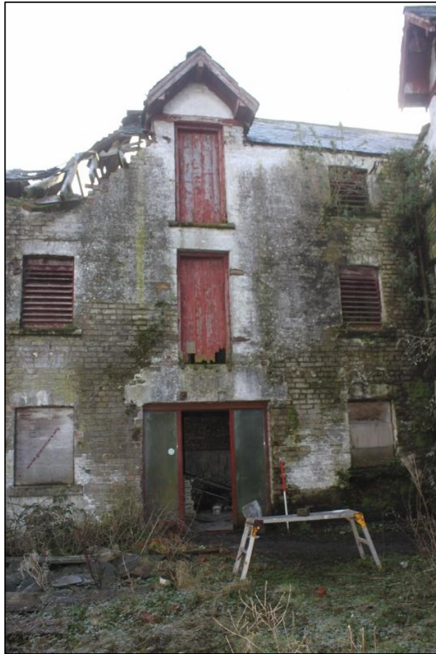
Figure 6a: S end of W Elevation, Element 2, Showing Transition from Two- to Three Storey Structure
