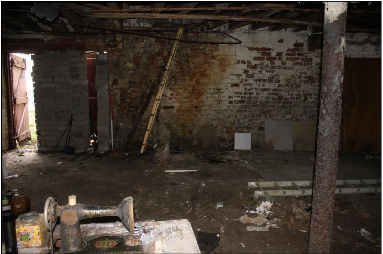
Figure 12a: Room C, E End of N Wall, with Modified Doorway to left
