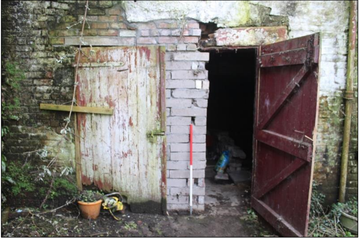
Figure 9a: Element 1, Original Entrance in N Elevation with Broken Timber Lintel (to right) and Modern Repair
