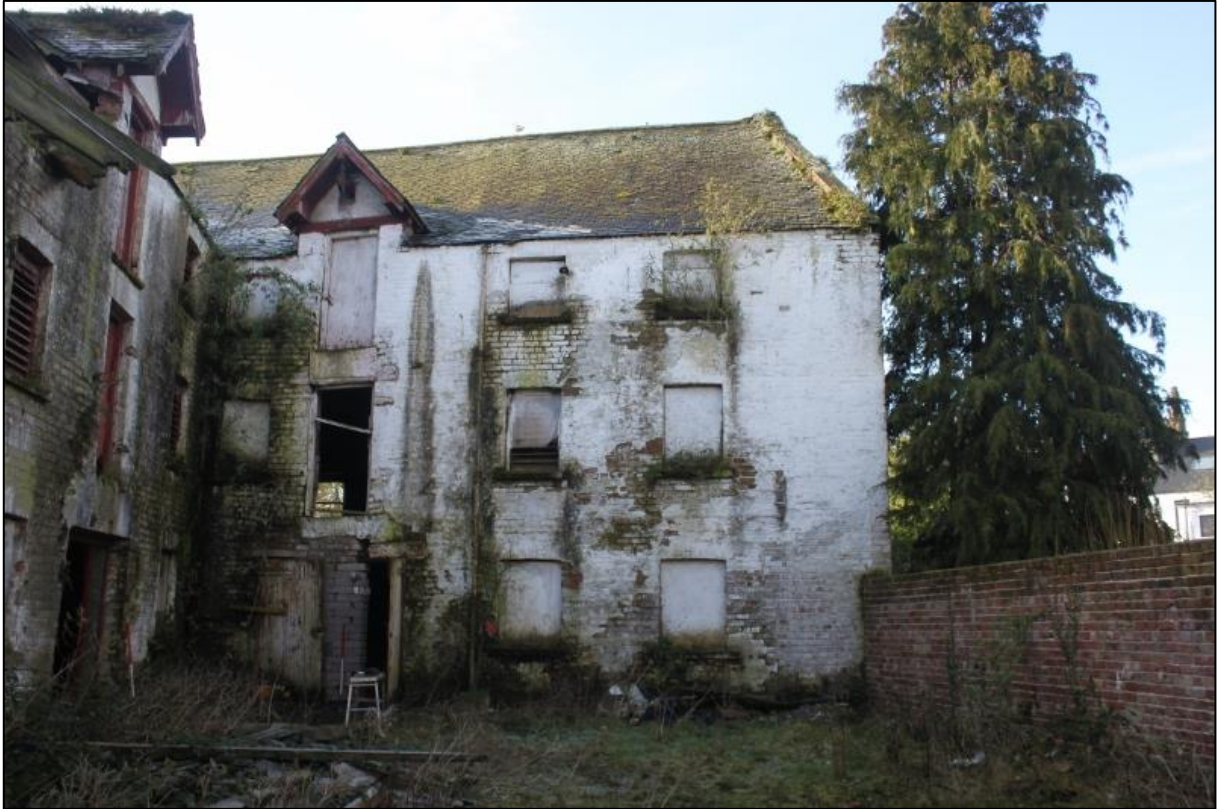
Figure 7a: N Elevation of Element 1, Showing Arrangement of Door/Hatch and Window Openings
