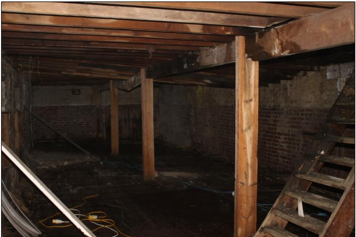
Figure 14b: General View of Room D, Showing Central Line of Timber Posts and Access Stair to Attic Level
