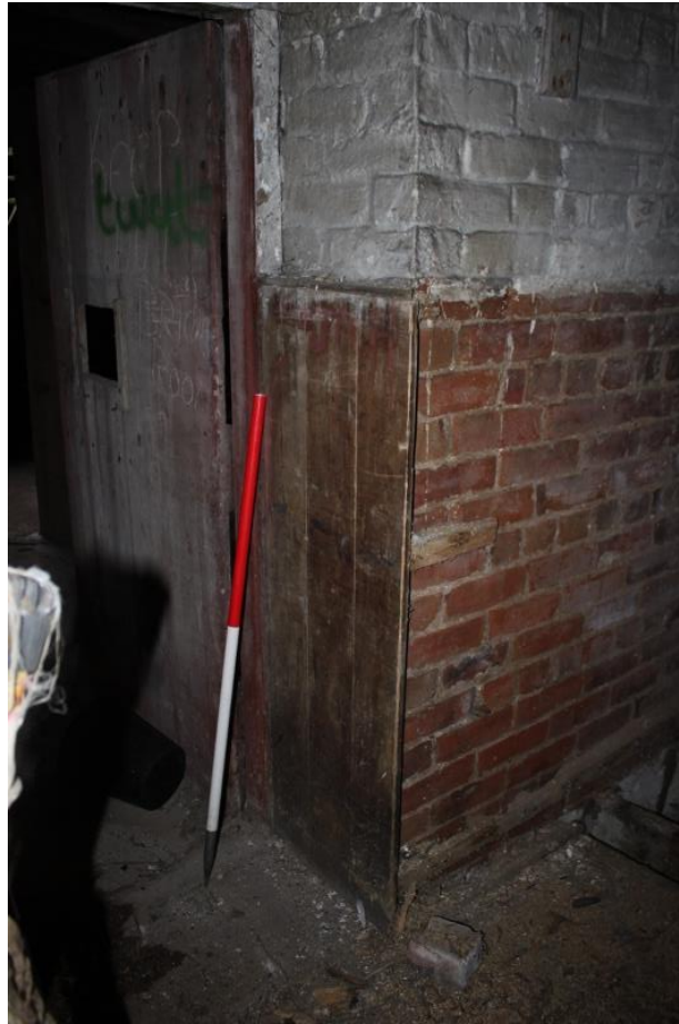
Figure 17a: Room E - In Situ Timber Panelling at Entrance to Room D
