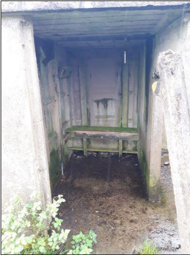
Figure 5a: Interior of roofed chamber in Orlit post at S8 showing bench along rear wall
